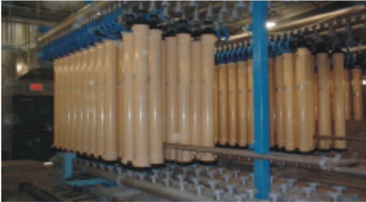
Microfiltration water plant, Petrolia, PA
