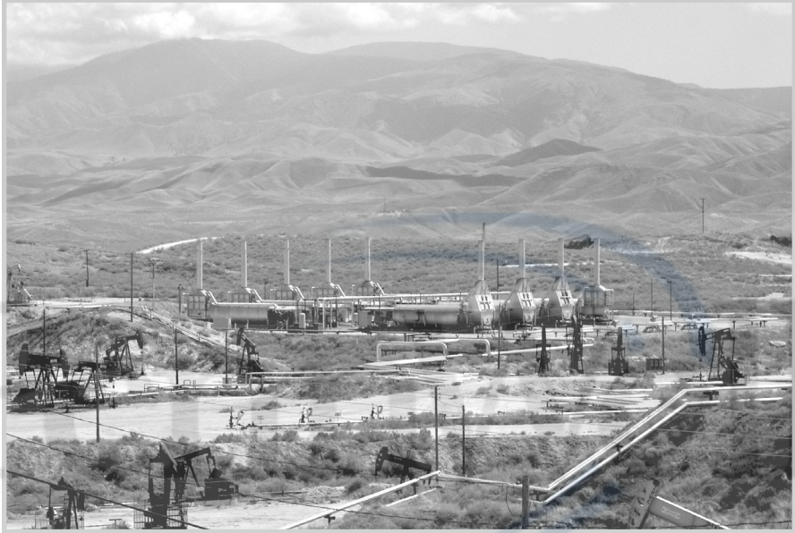
Fig. 8–16. Steam generators operating in a steam drive project. The Midway-Sunset Field, California. Courtesy of Aera Energy.
