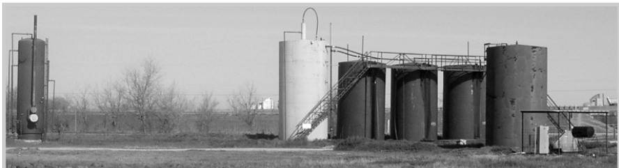
Fig. 9-8. Typical oil field processing facilities. From the left, a heater treater, a gun barrel FWKO, three oil storage tanks, and a large water storage tank with an injection pump and injection well in the right foreground.
