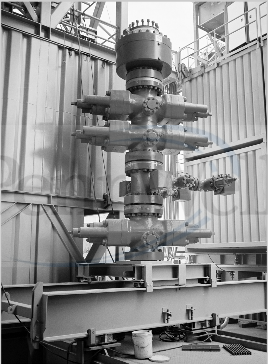
Fig. 5–16. BOP stack ready for installation. The device at the top is an “annular” preventer used to close against the kelly. The three devices below it are used to close against the drill pipe or to shear the drill pipe to seal it. Courtesy of Helmerich & Payne.
