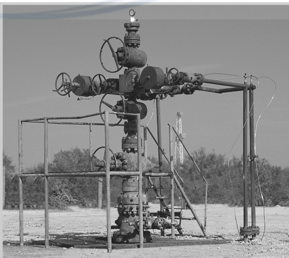
Fig. 6–21. Christmas tree for a high-pressure gas well. Wheels are used to open and close the valves which control production rates. Courtesy of Cooper Cameron.
