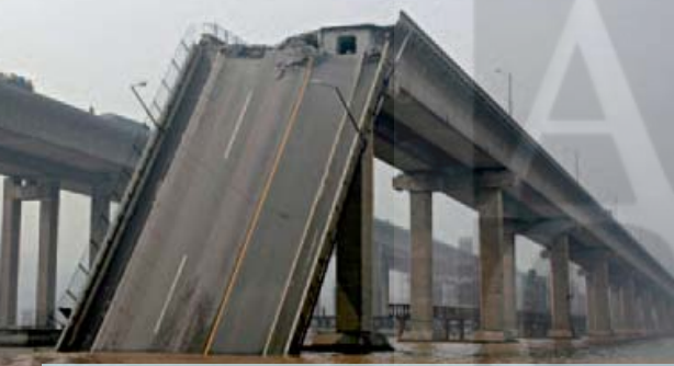
In 2007, a bridge collapsed in Nanhai, China, after a boat crashed into it.
