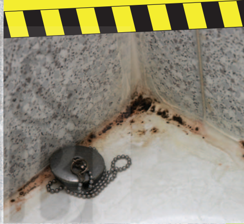
This damp, dirty bathroom corner is a perfect home for black mould.
