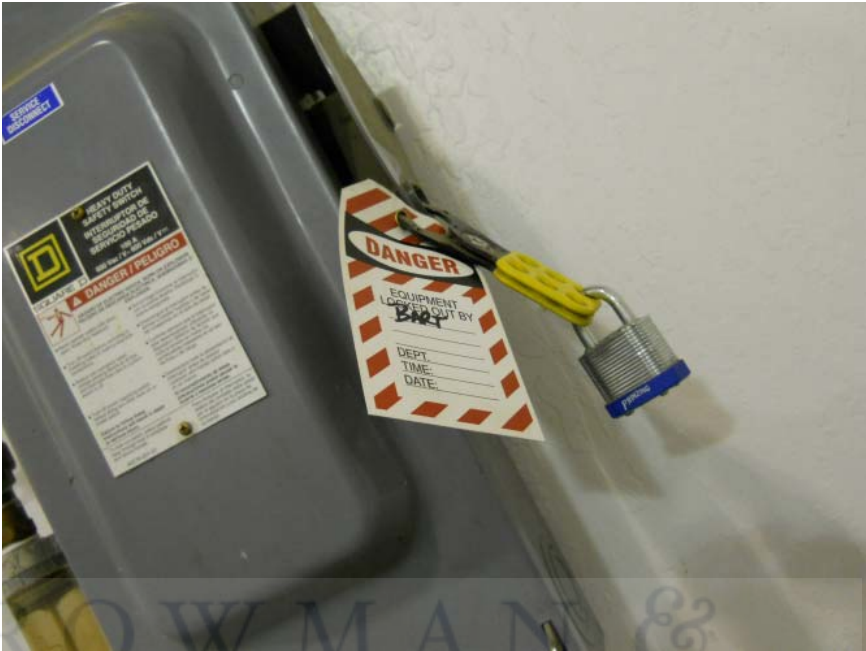
Figure 3.2. LOTO electrical box.
