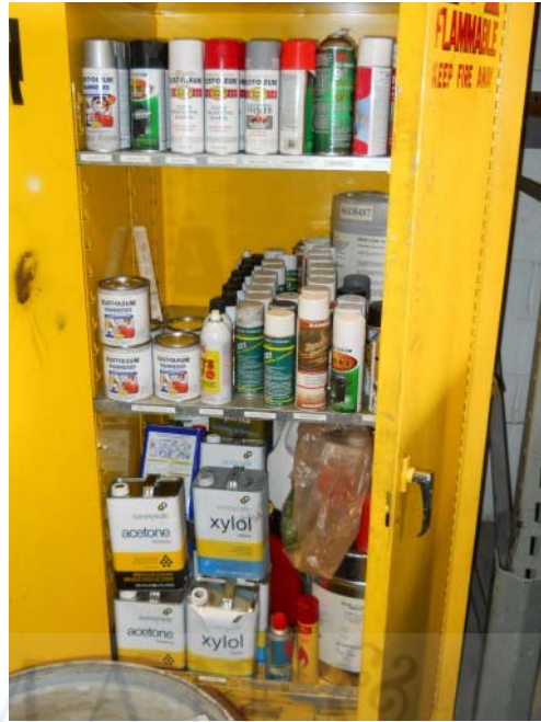
Figure 9.2. Open flammable liquid storage with placarding.
