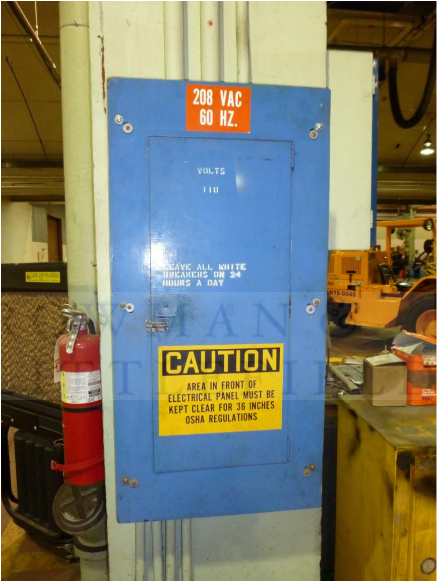
Figure 8.1. Electrical panel with a warning sign.
