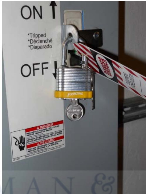
Figure 8.2. Locked and tagged electrical box.
