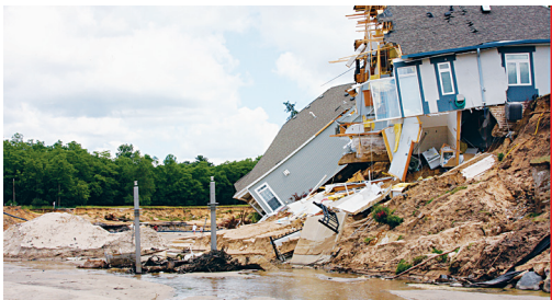
Landslide and mudslide damage.
