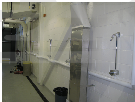
Figure 12-7: Multiple individual decontamination showers along the wall inside an ambulance bay at the Halifax Infirmary. Note drain channel along the floor, which drains into the a skimmer tank. Note also the lack of privacy curtains isolating casualties being decontaminated.
