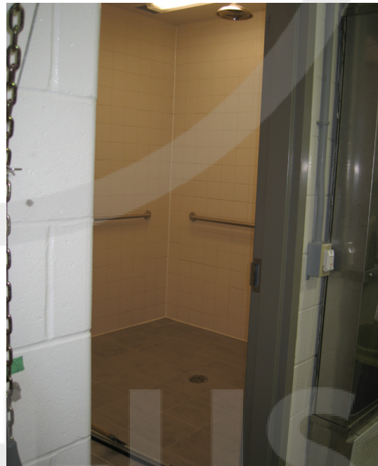
Figure 12-5: Individual decontamination shower off ambulance bay. Halifax Infirmary, QEII HSC.
