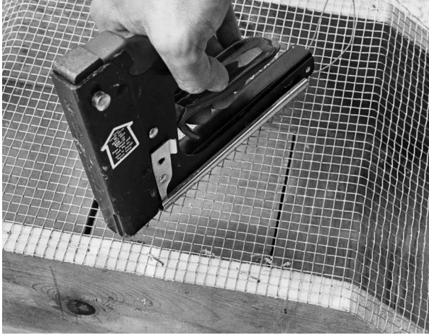
Using a stapler to staple the hardware cloth to the frame of the box.
