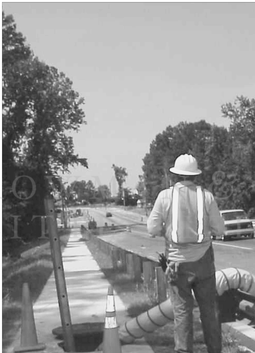
Figure 16-3. Confined space hazard
