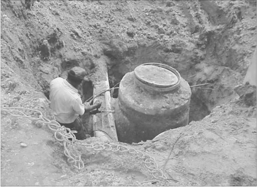
Figure 16-4. Potential for collapse
