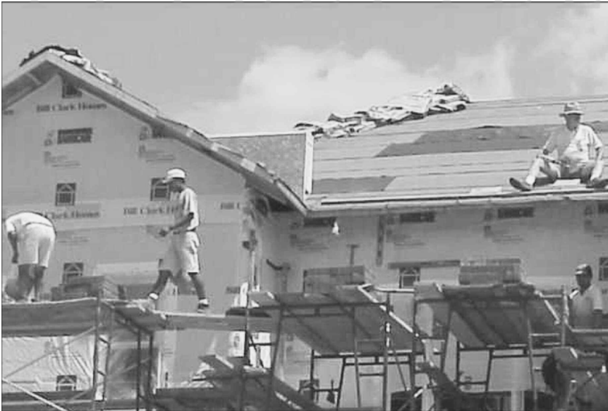
Figure 16-1. Lax safety practices in residential construction
