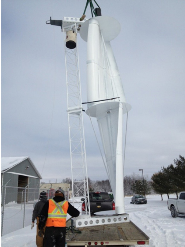
Figure 2.5. A small-scale wind turbine designed for telecommunication base transceiver stations during installation on a USA Department of Transportation telecommunication tower, 2012.
