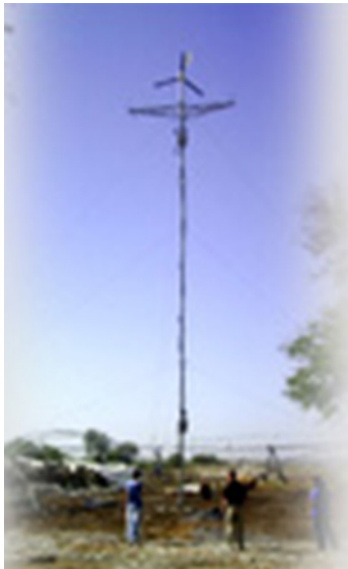
Figure 7.6. Wind turbine installed at Heelat Ar Rakah.
