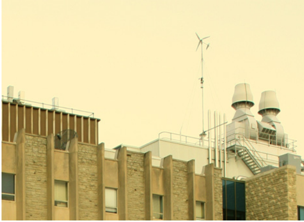
Figure 5.4. A small HAWT installed on the rooftop of the Western University Engineering building.
