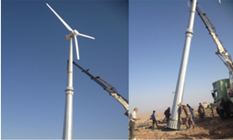
Figure 7.12. Free-standing tower for 20 kW wind turbine.
