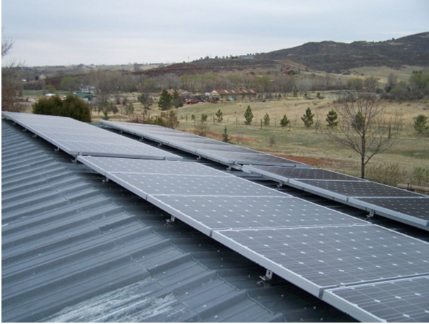
Figure 9.7. Metal roof flush-mounted PV array.
