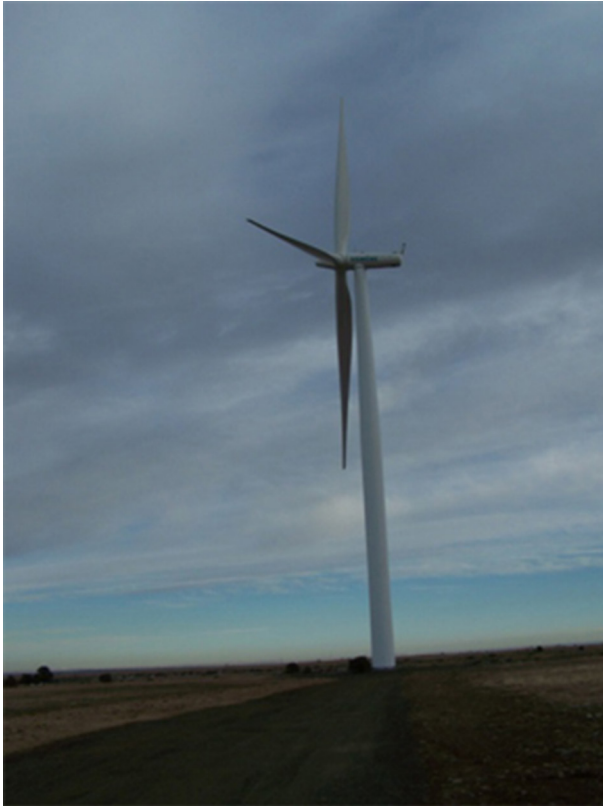
Figure 2.3. Wind turbine generator at National Wind Test Center. (Source: Courtesy of NREL.)
