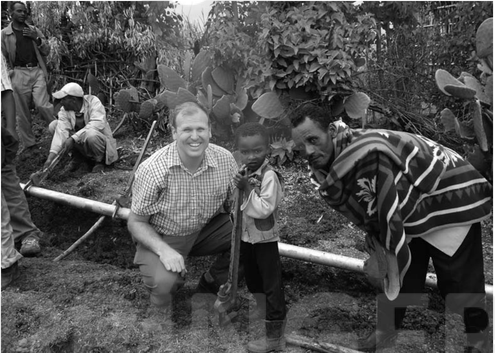
Gary White at the pipeline construction site (Ethiopia). Photo courtesy of water.org Flickr site.
