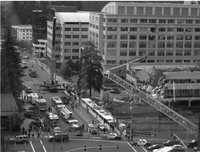
Figure I3.1b. Crane failure in Bellevue, WA, November 2006.
