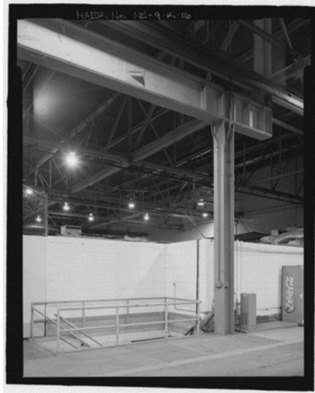
Figure 2.8. A beam (foreground top) supported by a column. Trusses are seen in the upper right.
