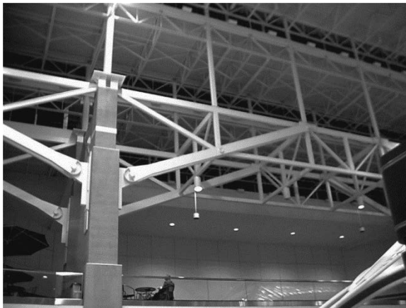
Figure 2.1. While the various members that make up the truss assembly may or may not be axial members, the rods supporting the hanging lights clearly are axial.
