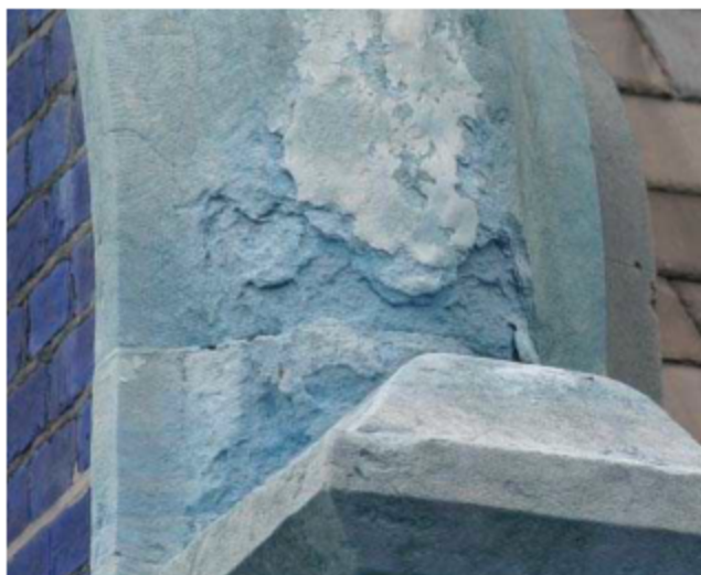
The damage on this building was caused by acid rain.
