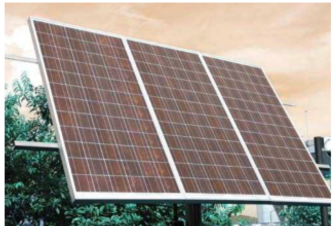
Solar panels convert the sun's energy into electricity.
