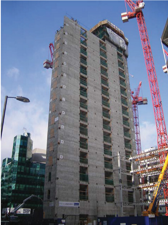
View from the south-east corner of slip-form core construction progressed to level 15 of 21, with the first four-storey bay of steelwork commenced.
