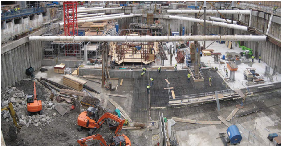
Site view to the south, showing the slip-form platform prepared for launch from the lower basement raft slab, between propped secant pile and existing buttress retaining walls.
