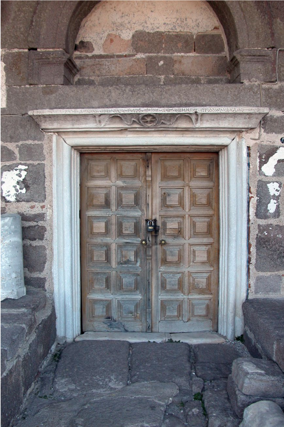
FIGURE 29.1 Behramkale (Assos), mosque of Murad I, c. 1380. Gate with reused Byzantine lintel from a church of St. Cornelius. Source: Zeynep Yürekli. Reproduced with permission.
