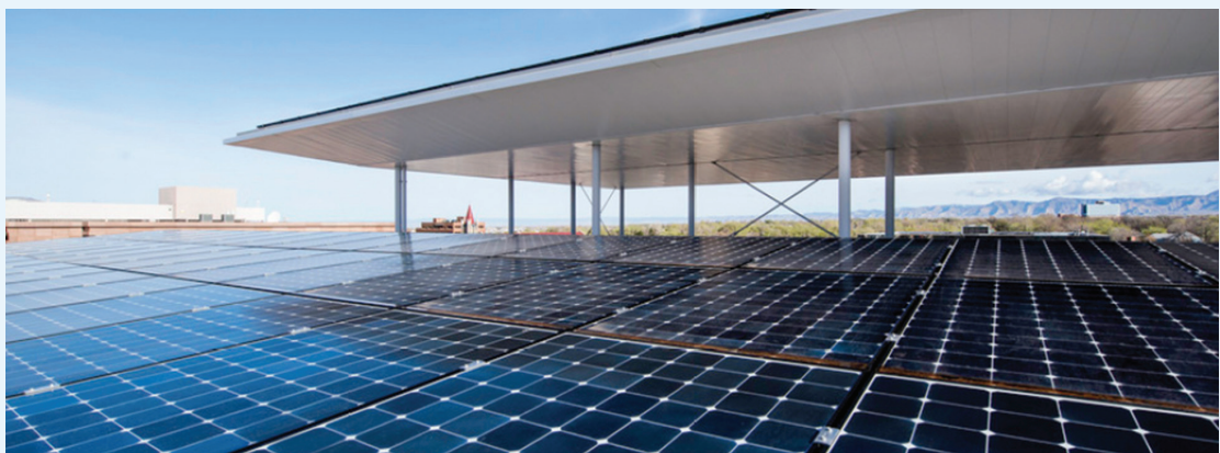
Figure 2-13 Rooftop PV array Photography by Kevin G. Reeves; Courtesy of DLR Group
