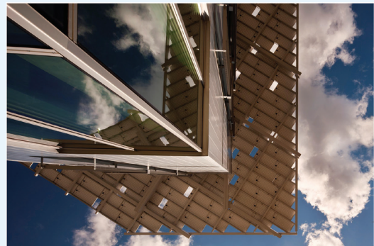
Figure 10-9 PV array overhang Image courtesy of The Miller Hull Partnership © Nix Lehoux
