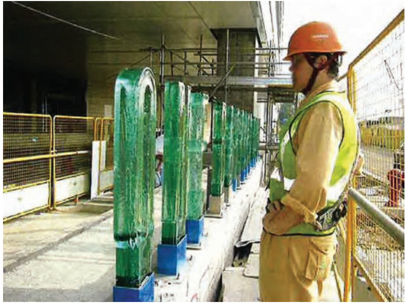
2.42 Observation phase: A construction worker inspects the partially completed installation of the monumental cast glass letters.
