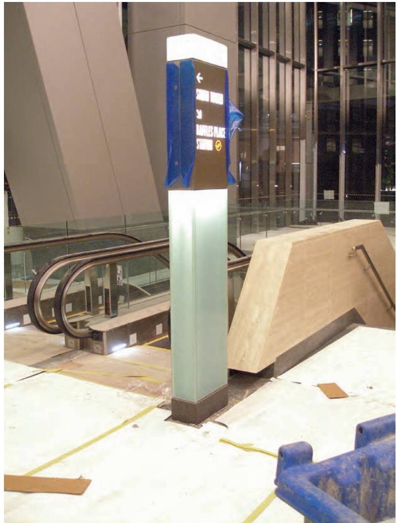
2.40 Observation phase: A finished pylon sign installed onsite still wears some of its blue protective sheathing.
