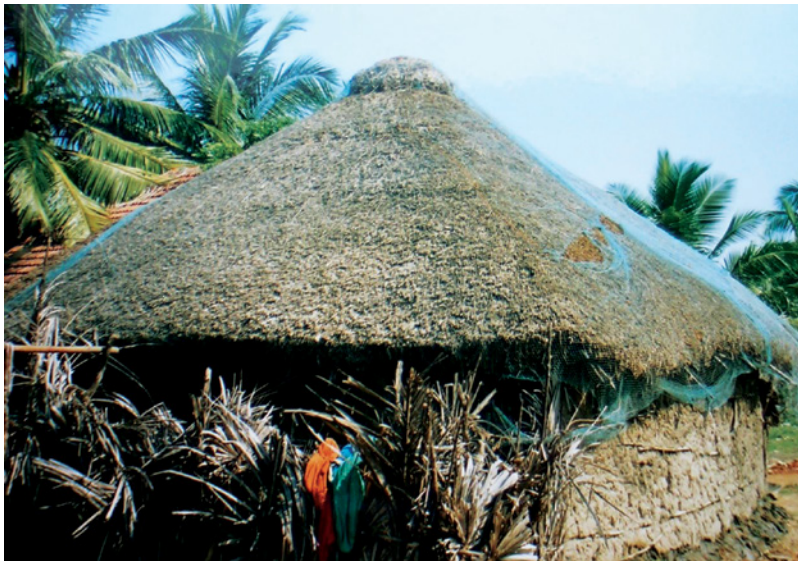
Figure 4.7 Traditional thatched 'kutcha' hut with fishing net used as storm protection. A practice used in the cyclone prone East Godavari region of Andhra Pradesh, India (Source: Boshier, 2002).
