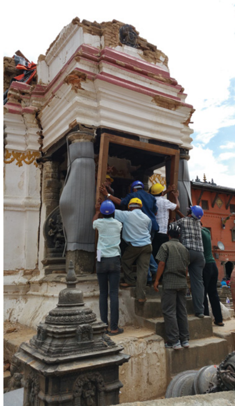
Figure 2.3 Reconstruction in Nepal after the 2015 earthquakes (Source: Reproduced with permission of Rohit Jigyasu).
