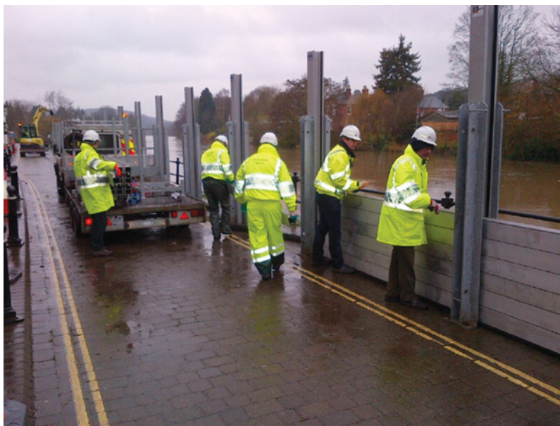
Figure 3.23 Part of the innovative temporary aluminium barrier system being deployed on the banks of the River Severn in Bewdley, England (Source: Reproduced with permission of David Throup).
