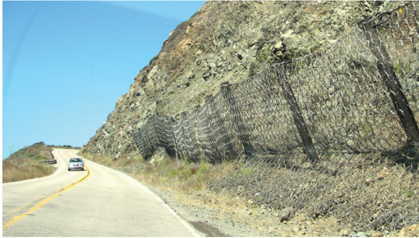
Figure 7.8 A catch fence installed along a slope to prevent debris and rocks falling onto the road (Source: emdot on Flickr).
