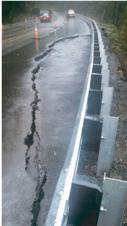
Figure 7.6 Cracking on road surface due to slope movement (Source: Oregon Department of Transportation).
