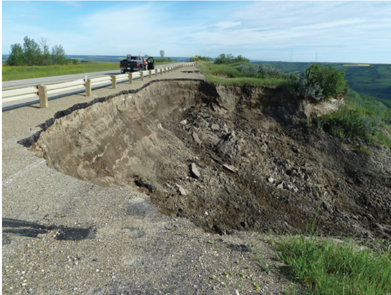
Figure 7.1 Landslide damage to a highway in Peace River, Alberta, Canada (Source: Reproduced with permission of Matthew Spriggs).
