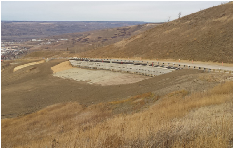
Figure 7.9 An anchored pile wall installed to stabilise a slope that was causing damage to a road in Peace River, Canada (Source: Alister Smith).
