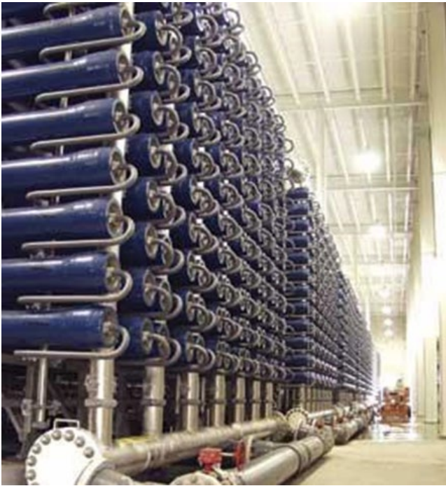
Figure 11.16 Tampa, FL water desalinization plant. Source: http://www.chem1.com/acad/webtext/solut/solut-4.html .
