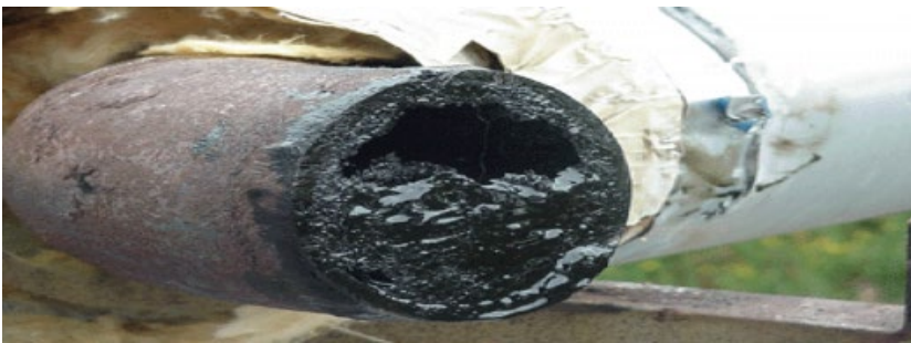
Figure 8.11 Pipe plugged with decomposed heat transfer fluid.
