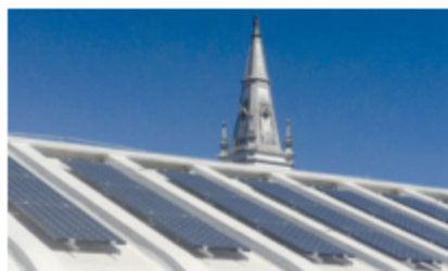
Figure 4: Photovoltaic energy power plant at BPE. (Rio de Janeiro. Secretaria de Cultura, 2014).
