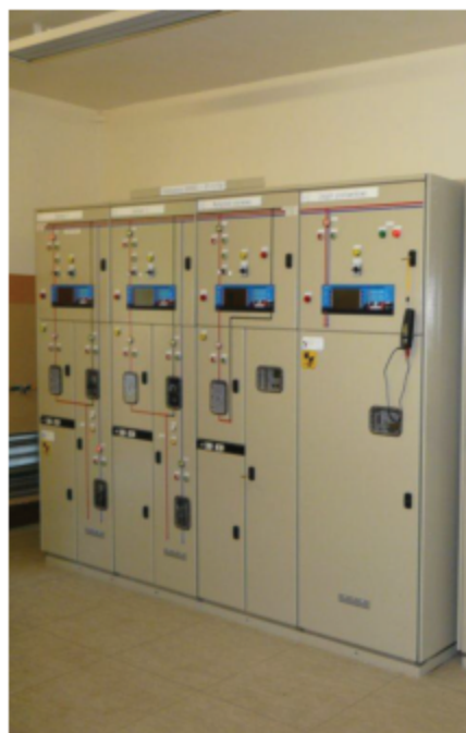
Fig. 4.14. DC switchgear of trolleybus substation, Gdynia, Poland
