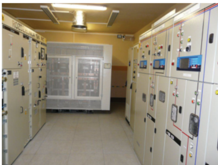
Fig. 4.13. Equipment of trolleybus traction substation: HV switchgear (left), rectifier unit in compact design (middle), DC switchgear (right), Gdynia, Poland
