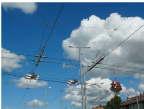
Fig. 4.9. High speed crossing of the tram and trolleybus overhead line. Szeged, Hungary
