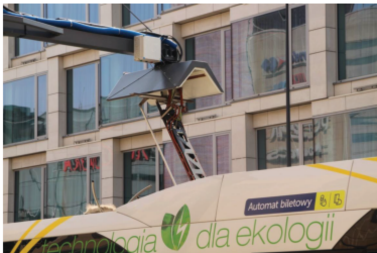
Fig. 2.3. Pantograph of charging system system Shunk (Kraków, Poland)
