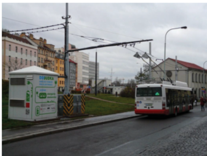
Fig 3.5. The charging station at Palmovka terminus with "Dobudka" converter station
