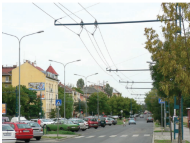
Fig. 4.5. Trolleybus contact line with additional overhead wires which reduces the overall resistance (Budapest, Hungary)
