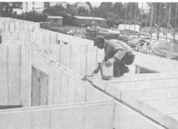
Fig. 5 - Partitions and roof (partially erected) of housing units constructed with autoclaved cellular concrete.
