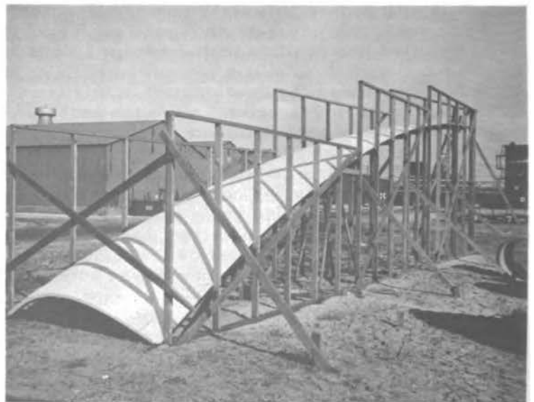
Fig. 2 - Full-scale section of 100' diameter dome, showing extruded polystyrene foam "form boards" arched in place before spray application of concrete surface.
