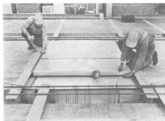
Figure 5. Polyethylene coated paper liner is spliced and sealed with polyethylene coated cloth tape.
