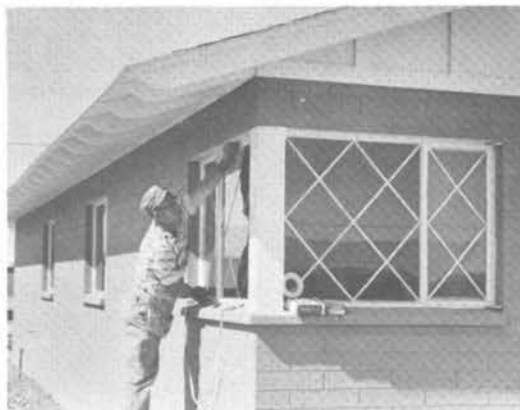
Figure 2. Lead tape is used to simulate leaded windows or diamond wood grilles.
