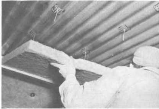
Figure 1. Insulation impaled on hangers attached to corrugated sheet with adhesive.
