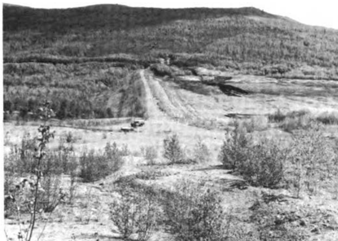
Fig. 6. General view of Hess Creek Dam from the west borrow area showing eroded spillway channel in the background
