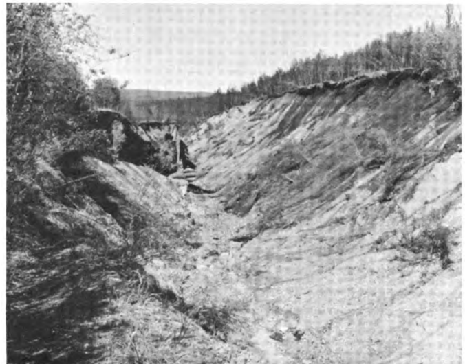
Fig. 7. View upstream in eroded spillway channel. Flat center area is at original elevation of the spillway apron
