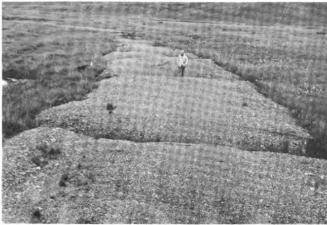
Fig. 5. Roadway destroyed by thawing of ice-wedge tops at Umiat, Alaska. Gravel fill was not thick enough to replace insulating effect of the organic mat which it destroyed (photo by Gordon W. Greene)
