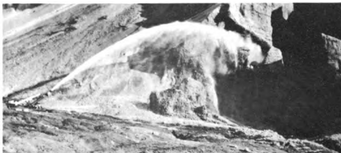
Fig. 2. Hydraulic stripping of muck overburden to expose underlying frozen gravel and sand
