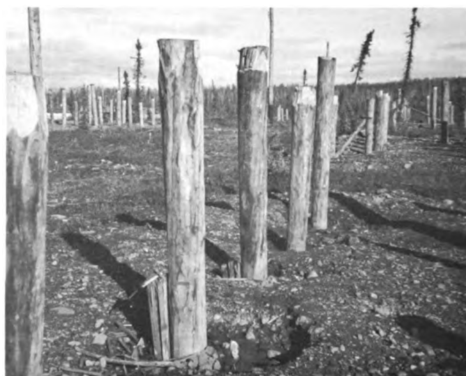
Fig. 8. Straightened piles. Note variability of driven depth, wedges, and ground subsidence
