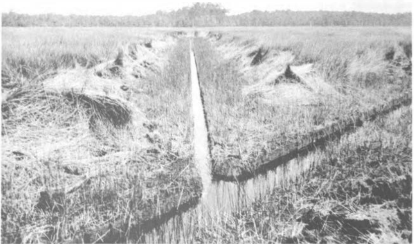
FIGURE 25 A 30-inch main ditch and 10-inch lateral ditch in a salt marsh. Spoil dirt is placed in piles, permitting water to flow from the marsh into the ditch. Ditch is dug to low tide level, allowing access of mosquito fish. (USDA photograph)
