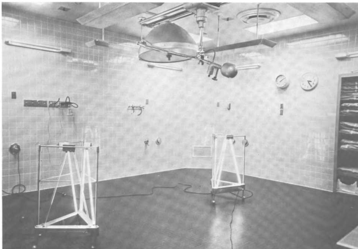
Fig. 5-D. The same room with ultraviolet lights turned off and conventional lights turned on. Note the air inflow disc in the ceiling above the wall clock. The upright Duke-Hart UV lights are used to decontaminate the floor, the sidewalls, the air and the entire room after a known contaminated wound is treated. The intensity of the upright lights is about 100 \text{ MW/cm}^2/\text{min} at a distance of about nine feet. At a distance of 20 feet, these lights are still effective in killing bacteria in the air and on exposed surfaces.
