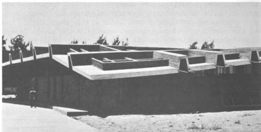
FIGURE 1 (a) Damage to school at Varto, Turkey, from (b) earthquake on August 19, 1966. (Photo U.S. Geological Survey, R. E. Wallace.) (b) Sagging roof due to column failure at the Agricultural University from the earth- quake at Lima, Peru, on October 3, 1974. (Photo L. A. Wyllie, Jr.)
