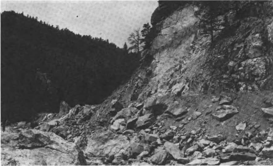
FIGURE 56 Rock Fall along Highway
