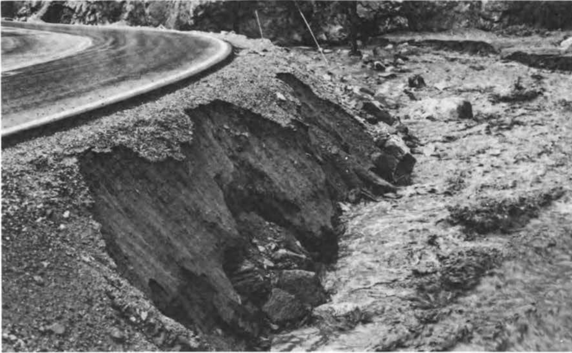
FIGURE 45 Repaired Highway Embankment Eroded by Water from Tributary
