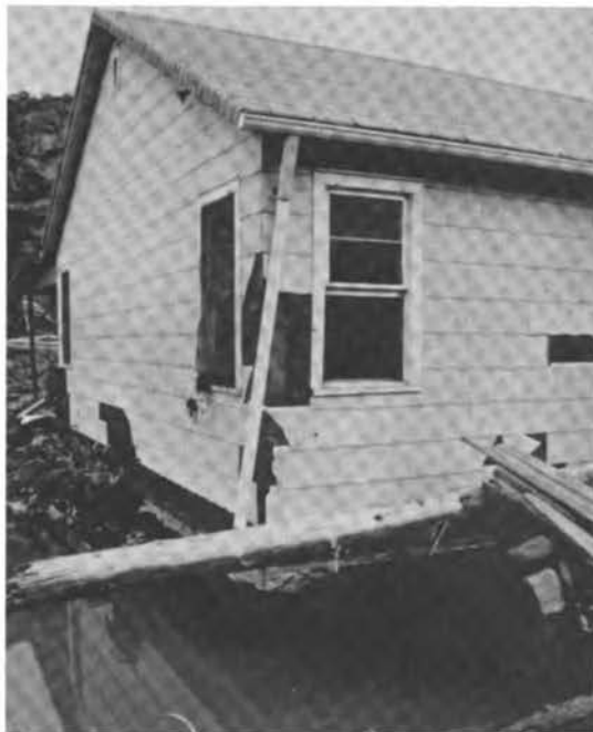
FIGURE 54 Erosion below Slab on Grade Foundation
