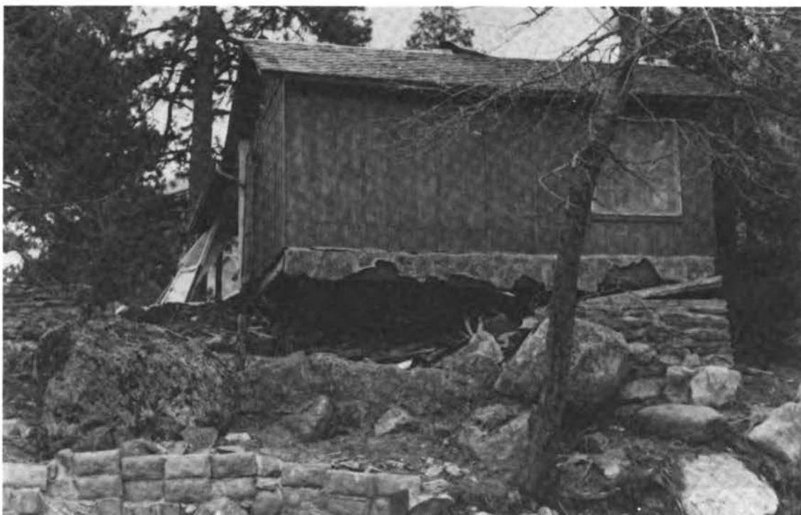
FIGURE 49 Failure of Timber Foundation with Stone Masonry Facing
