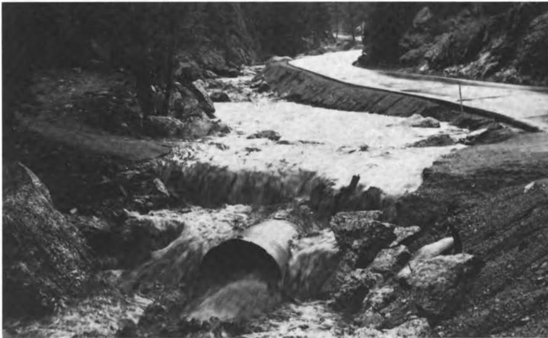
FIGURE 46 Storm Waters Washing over Culvert
