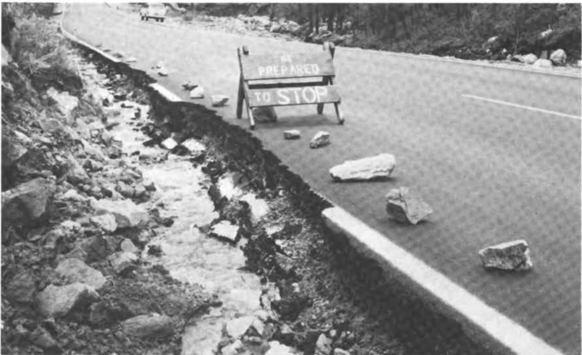
FIGURE 44 Repaired Pavement Eroded by Scour in Drainage Ditch
