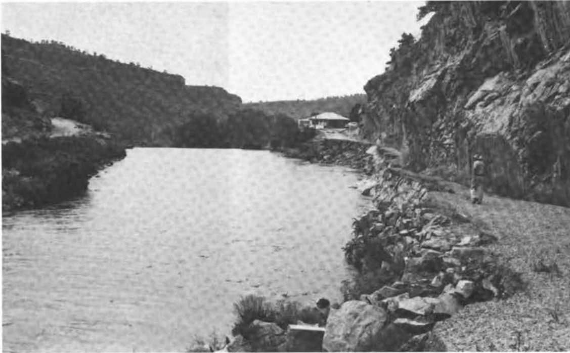
FIGURE 37 Erosion of Road between Bridge and Dam at Loveland Filtration Plant
