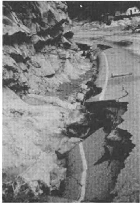
FIGURE 38 Scour in Drainage Ditch on inside of U.S. Highway 34
