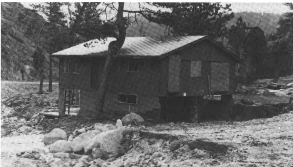
FIGURE 50 Failure of Concrete Block Foundation
