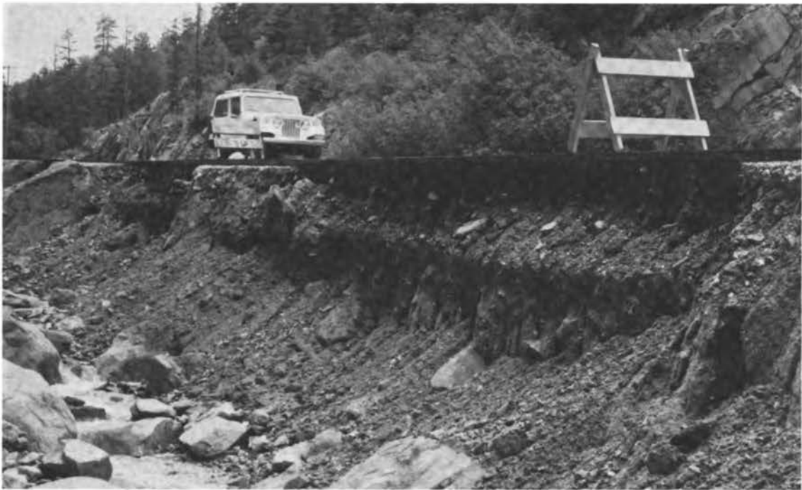
FIGURE 43 Repaired Highway Embankment Washed out by Subsequent Storm
