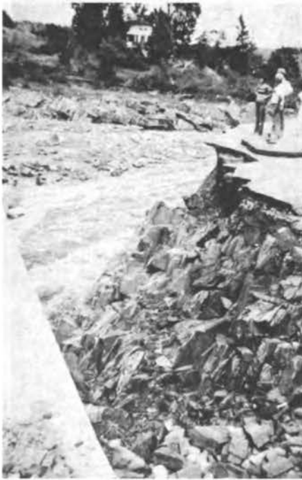
FIGURE 40 Erosion of Backfill Material at Bridge Abutment
