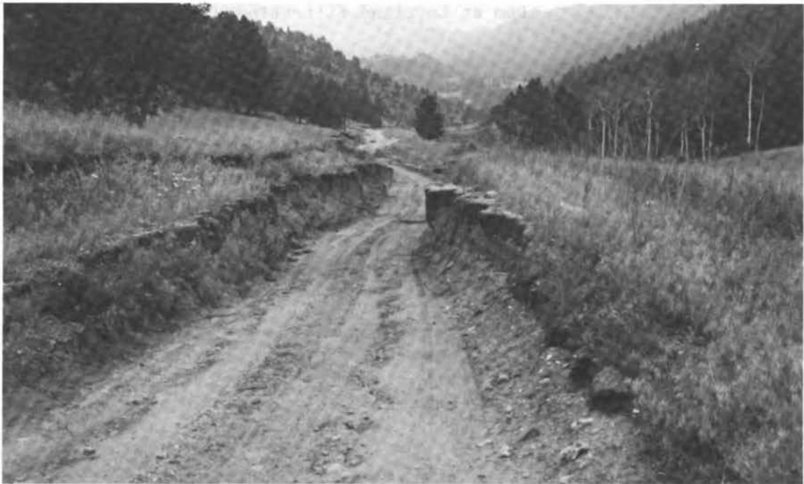
FIGURE 39 Extensive Gullying in Dunraven Glade Area
