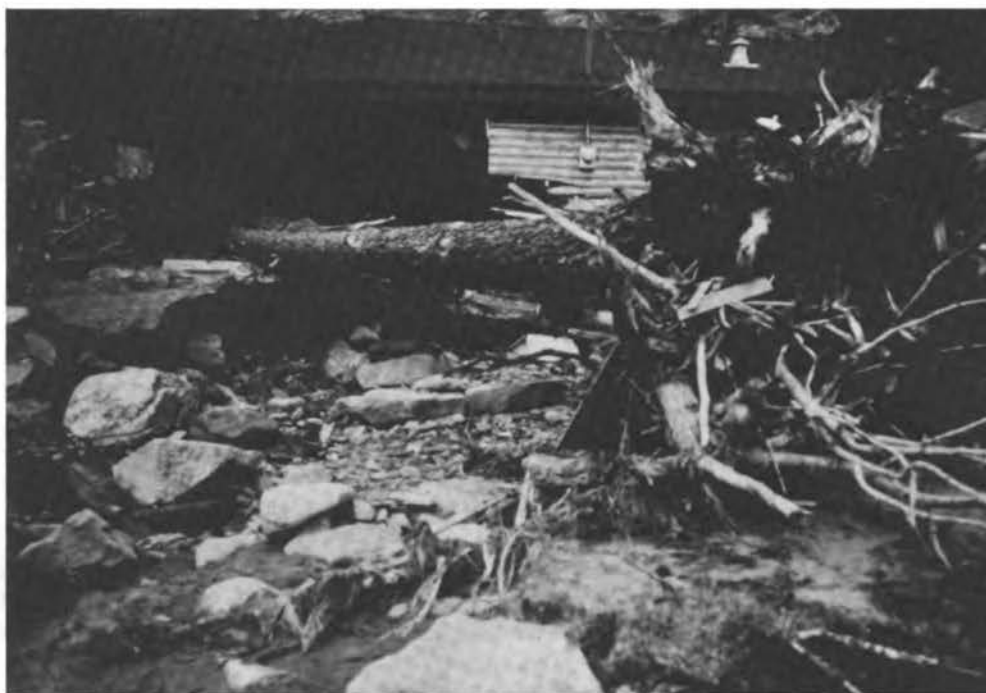
FIGURE 66 House Damaged by Tree Hurlled through Upstream Wall
