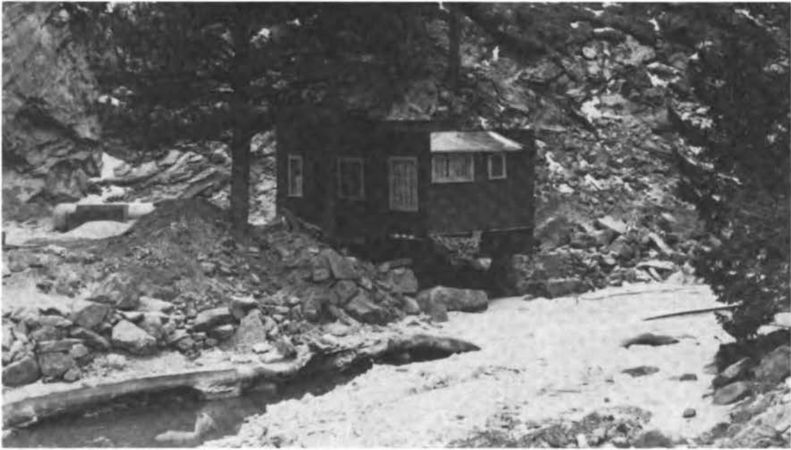
FIGURE 51 Erosion of Foundation Bearing Material
