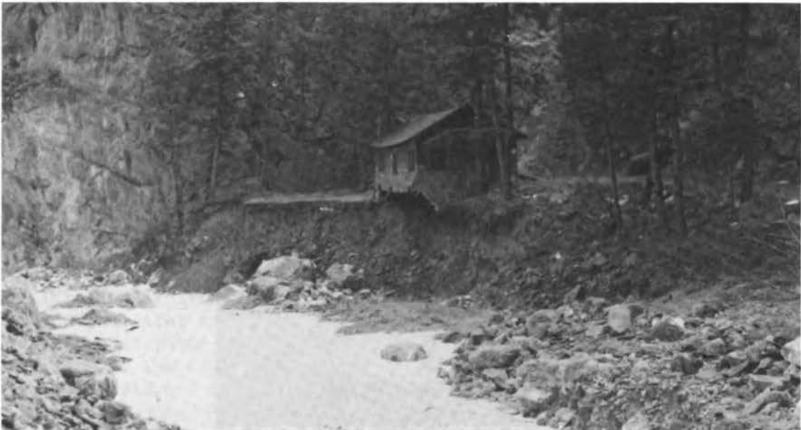
FIGURE 52 Erosion of Debris Fan below Foundation
