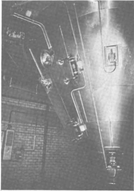
Fig. 65: \frac{3}{4} " suppression system on the cone of a spray dryer
