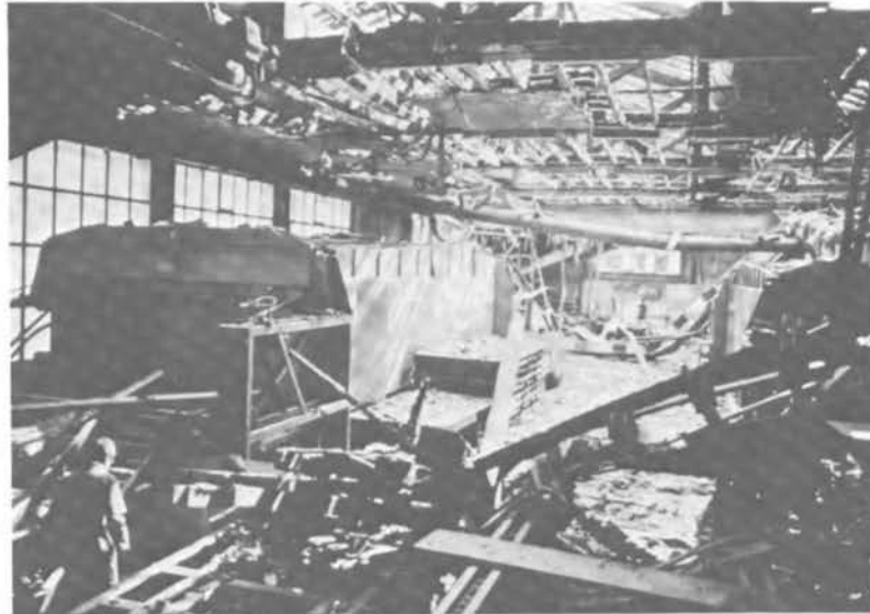
Fig. 2: Production room of a chip board factory after a wood dust explosion
