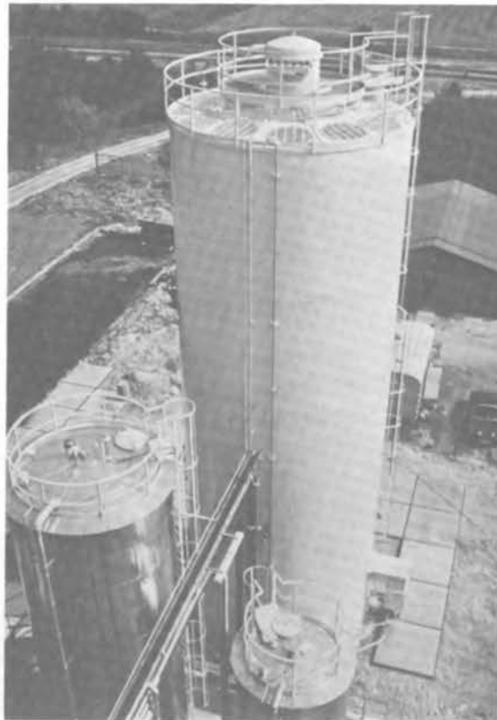
Fig. 53: Roof area of a silo designed for pres- sure relief
