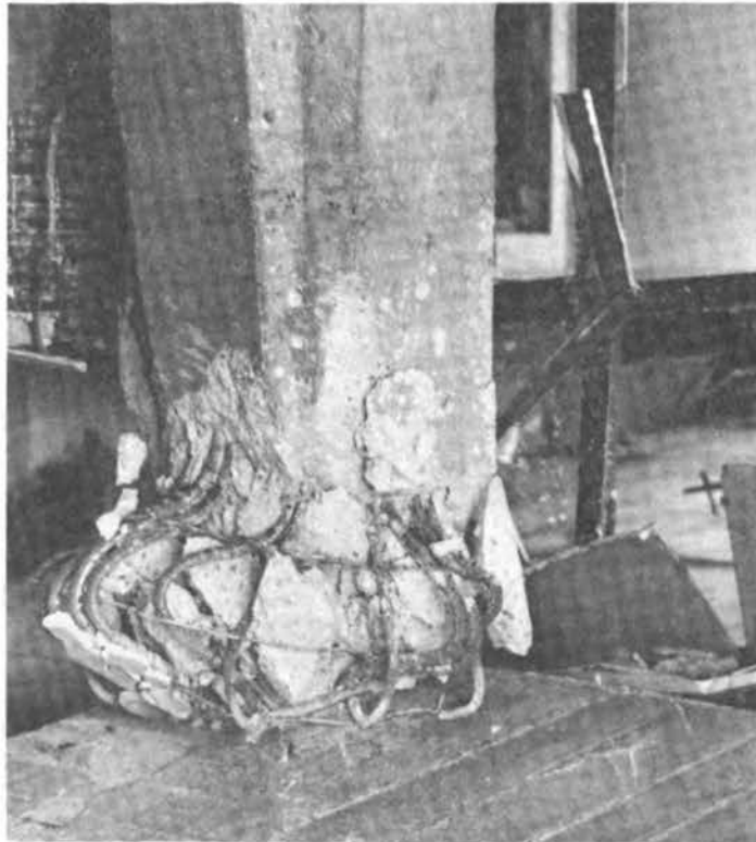
Figure 27 Computing center, column failure in ground story.
