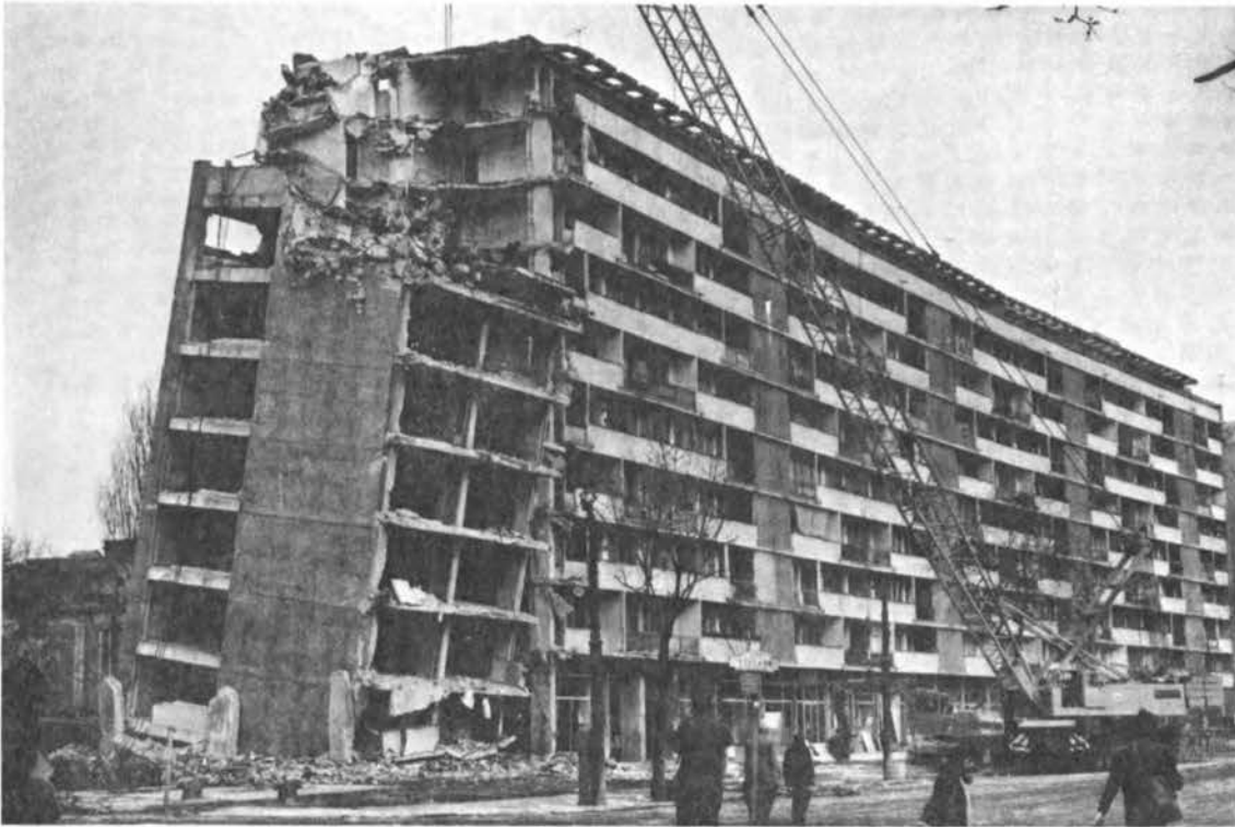
Figure 19 Partial collapse of new apartment building.
