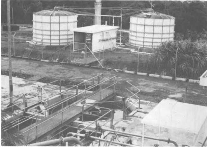
FIGURE 4.8 Two 95-m 3 bag-type digestors used at the Animal Health Research Station near Bogor, Indonesia. The center column is used to scrub carbon dioxide and impurities from the biogas. The shed contains the controls, compressors, and heating systems for the digestors. (Sanamatic Tanks Pty. Ltd.)
