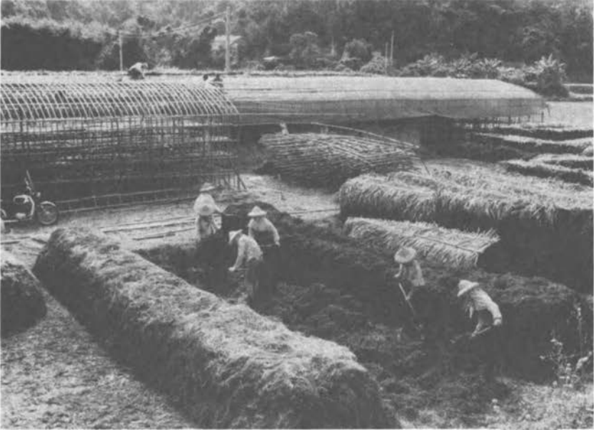
FIGURE 2.2 While mushroom-growing houses are being erected, rice straw compost is prepared for use. (J. C. Lee)
