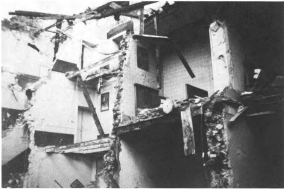
Figure 23. Typical damage to old construction. Note paintings and furniture still in place in the lower photo.
