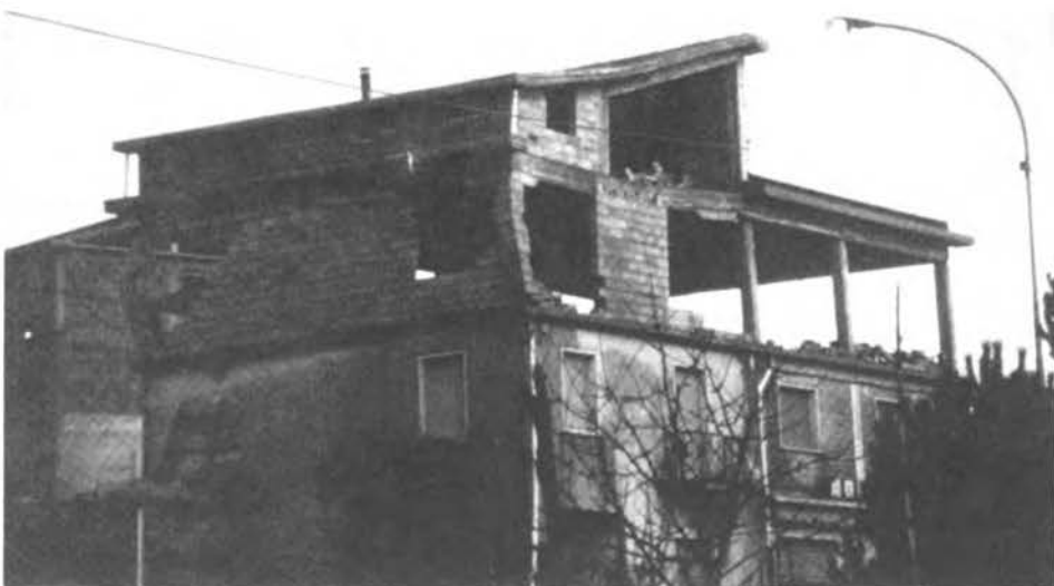
Figure 22. Damage in the town of Lioni. (a) Many two-story and 3-story residential units such as these suffered the typical failures caused by infill walls.
