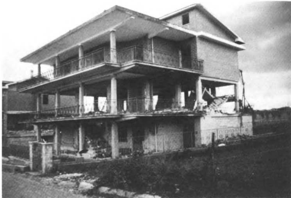
Figure 13. Examples of damage to concrete frames with infill walls.
