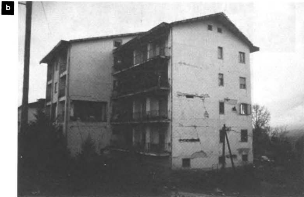
Figure 20. Damage to housing and police headquarters. (a) This 4-story housing unit was totally collapsed. Debris operations had not yet reached this structure. (b) Typical damage to multistoried concrete frame units. Note the outline of the frame.
