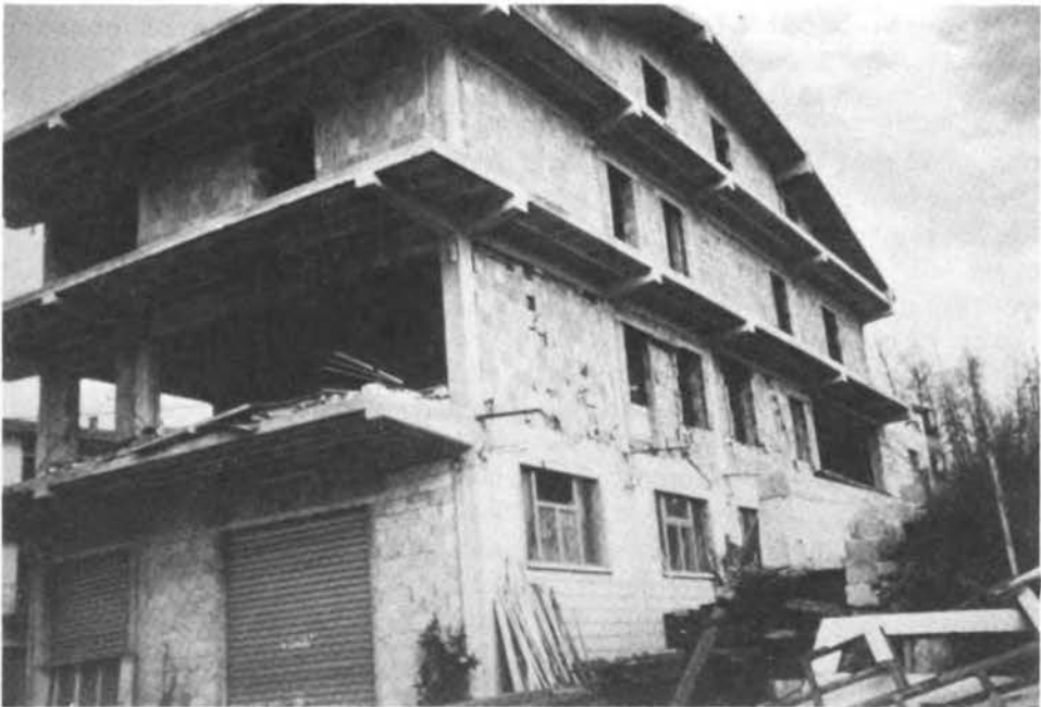
Figure 13 (cont'd). Examples of damage to concrete frames with infill walls.
