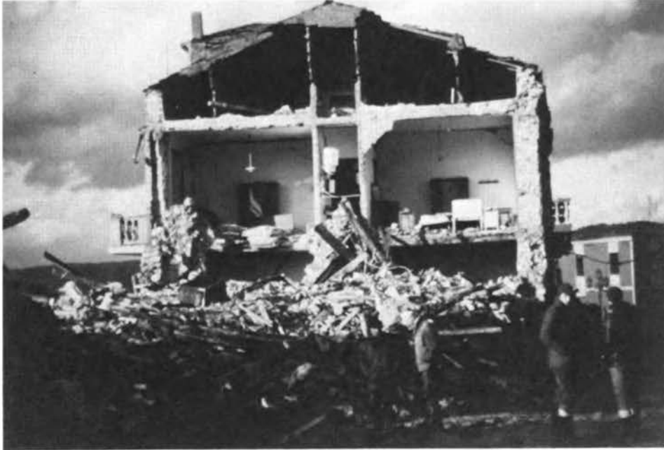
Figure 9. Typical failure of residences with wood floors and roof.
