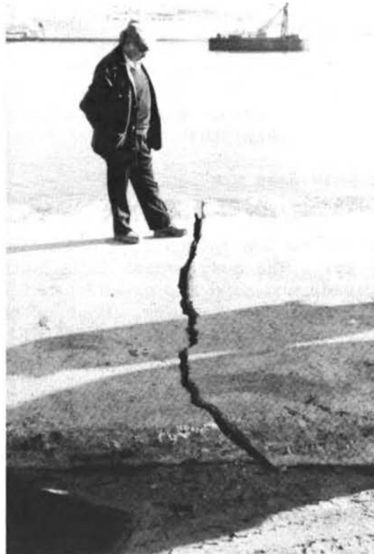
Figure 34. Damage at the harbor of Salerno. Crack in large masonry and concrete pavement of the quay.
