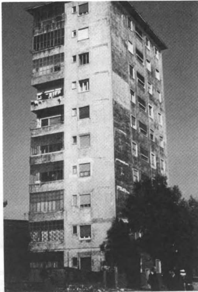
Figure 15. Damage to concrete structures with infill walls. (a) A large housing project of 5-story and 10-story units, all constructed of concrete frames with infill walls. (b) Shows a 10-story surviving unit, similar to the one that collapsed.
