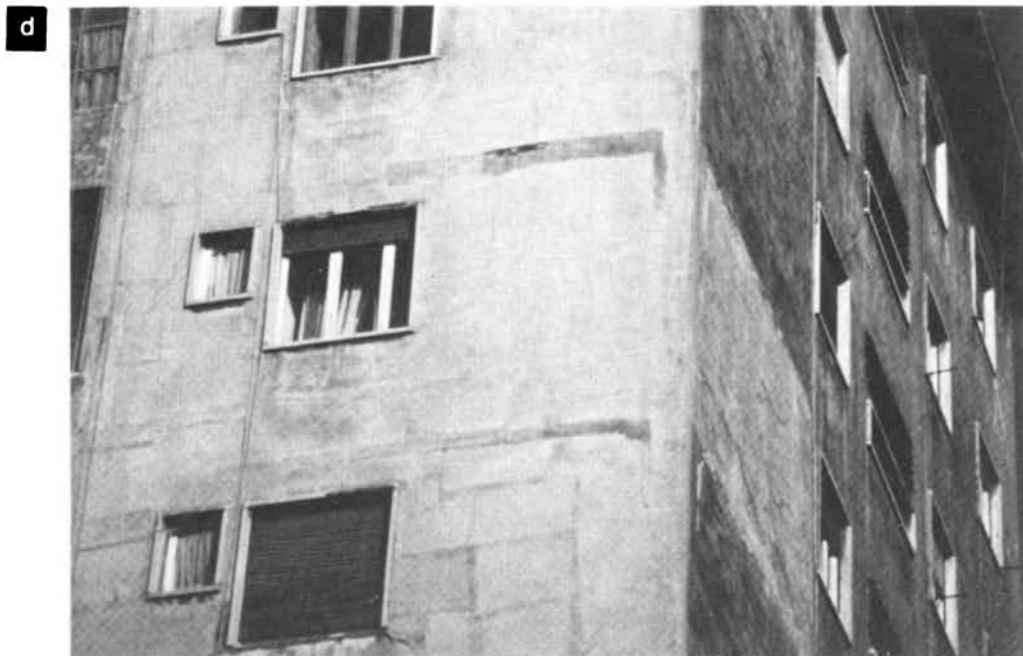
Figure 15 (cont'd). Damage to concrete structures with infill walls. (c) Shows basement of collapsed 10-story unit. Note damage to nearby residence due to collapse of high rise unit. (d) Patchwork of some kind had been done in the past at floor lines of surviving unit.
