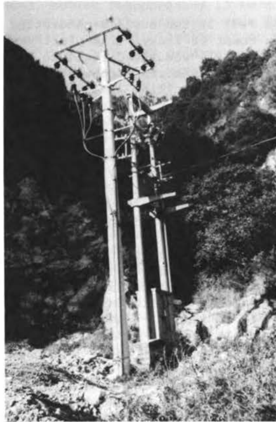
Figure 32. Electric power near Salerno. Small distributing station.
