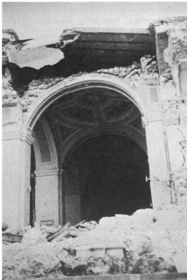
Figure 27. Damage in Balvano. Two views of the collapsed church in Balvano.
