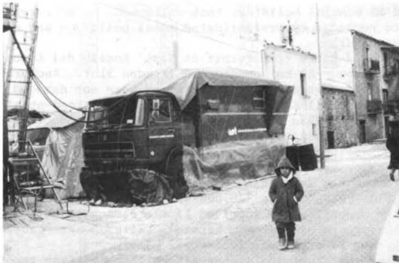
Figure 29. Mobile generator unit supplying approximately 10 kilowatts of electrical energy to communications and other equipment in Balvano.
