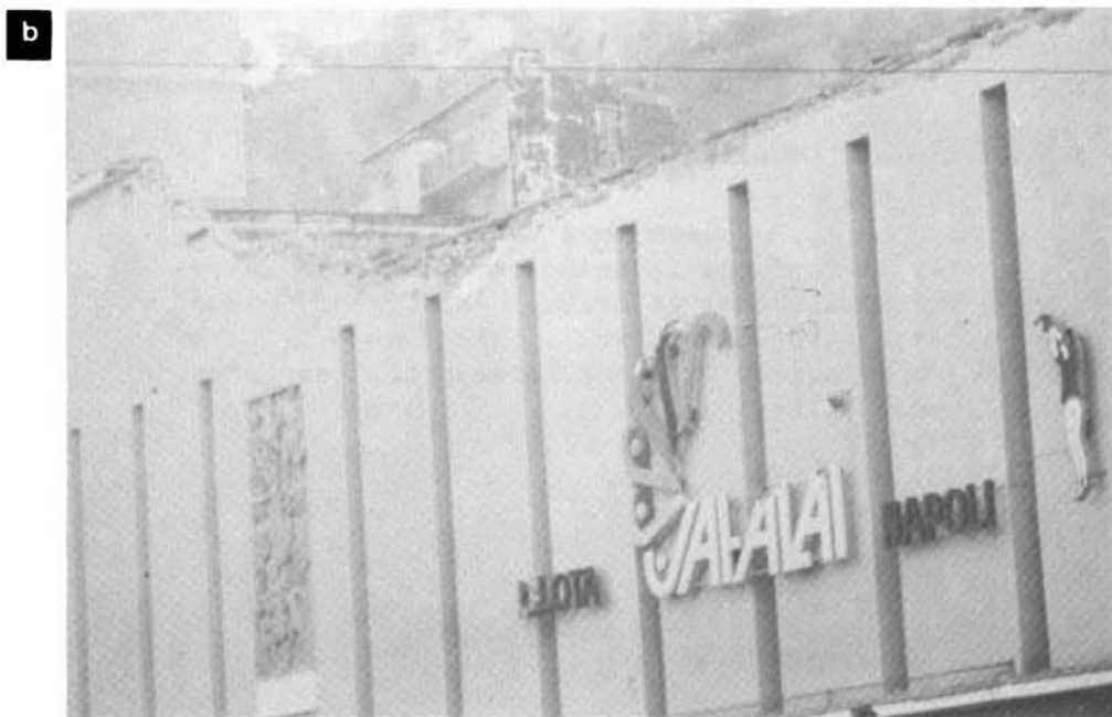
Figure 17. Damage to the Jai Alai stadium. (a) The stadium had a failure of its high, unbraced parapet wall. (b) This close-up shows that the very high, unreinforced parapet was not properly anchored to the wood roof system.
