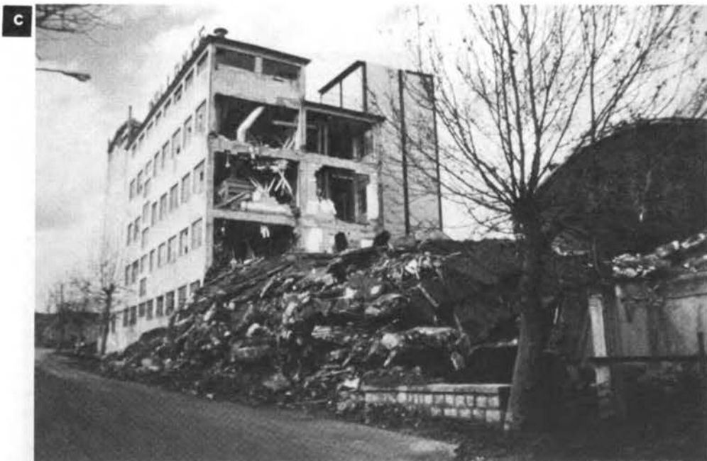
Figure 21 (cont'd). Damage to the Pallante factory. (b) The Pallante "pasta" factory has a concrete frame with infill walls. (c) One unit of the factory has collapsed. Some infill walls of the remaining structure have also failed. The failure occurred at a construction joint.
