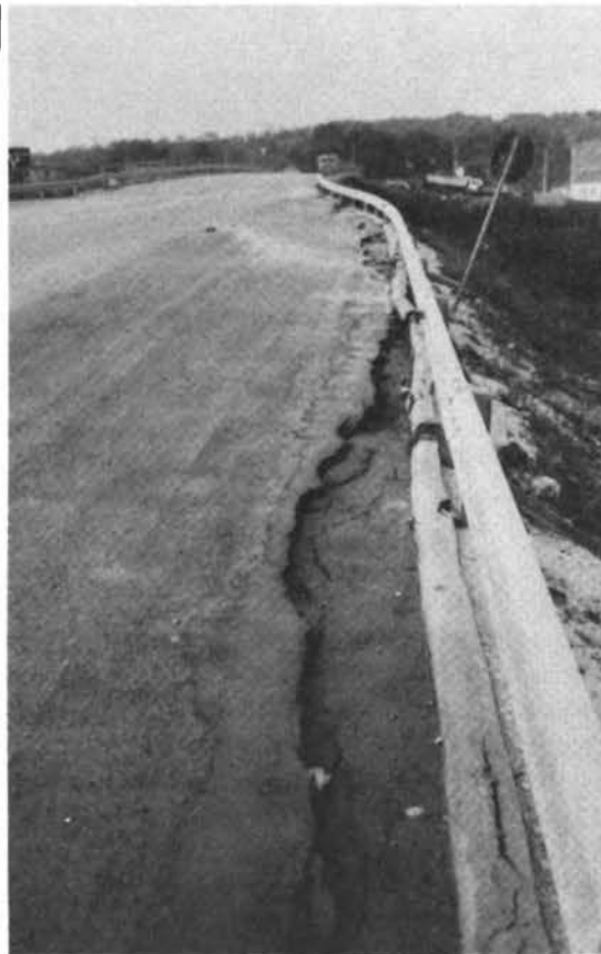
Figure 36. Damage to roads. (a) Cracks in road pavement near Lioni. (b) Damage to pavement and slope of roadway near Lioni.
