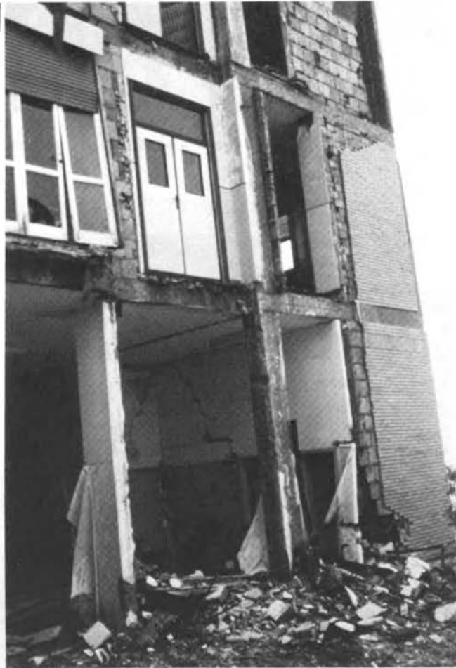
Figure 19 (cont'd). Damage at Sant' Angelo dei Lombardi (g) Two views of the damaged hospital. (h) Close-up view of the corner of the hospital shows the damaged walls and columns. An aftershock could easily cause the rest of this structure to collapse.
