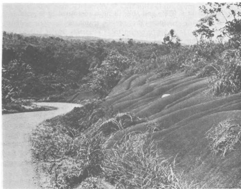
FIGURE 8-2 Erosion along roadways, such as this road associated with the Surinamu Reservoir above Port Moresby, Papua New Guinea, can be a serious source of sediment. Particular caution should be exercised in the drainage area during and after construction. (Courtesy, C. R. Goldman)
