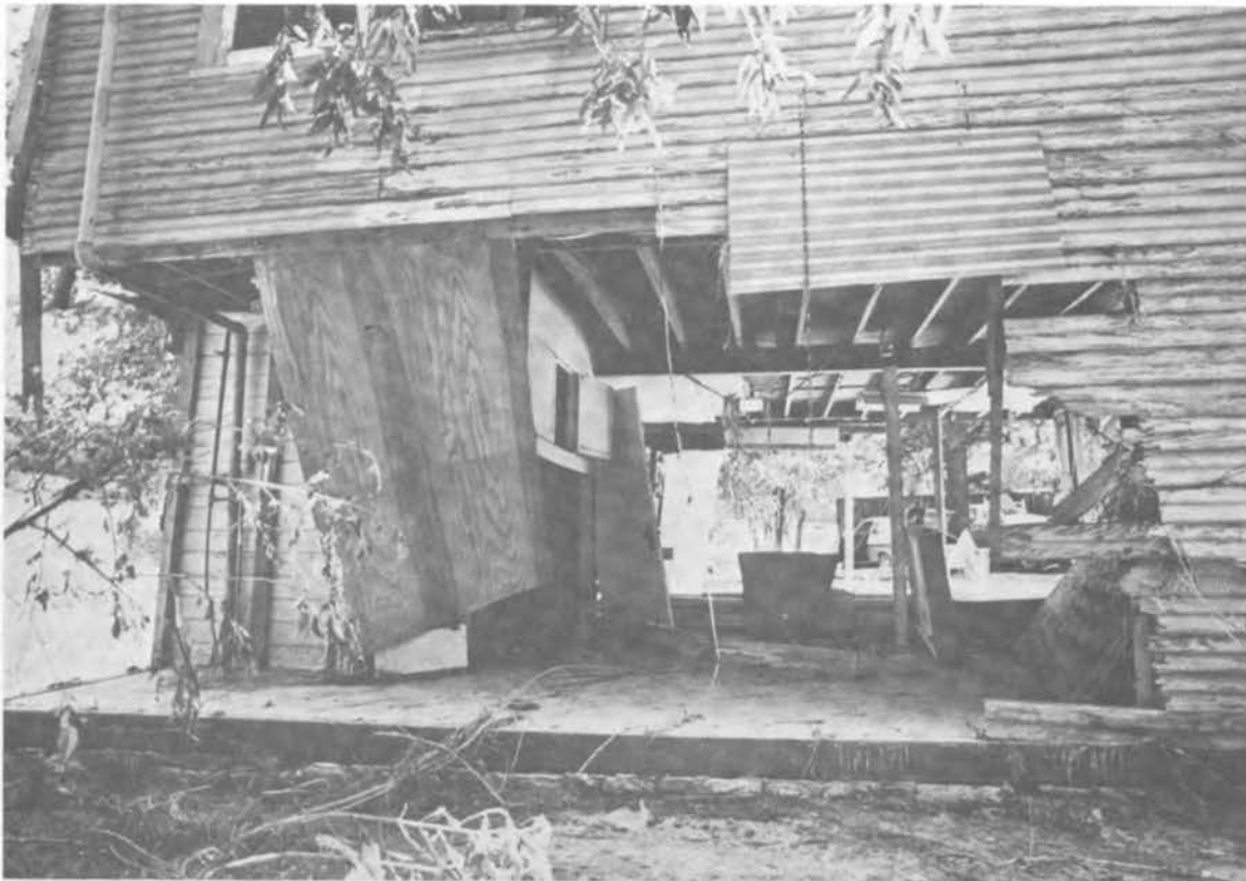
FIGURE 3.3 Washed-out first floor of a house on Tenth Street. (Photograph courtesy of the Austin American-Statesman .)
