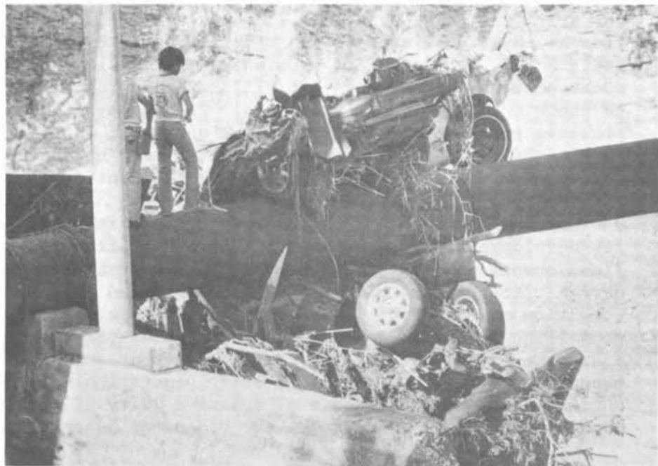
FIGURE 3.7 Debris washed against water main crossing Shoal Creek.
