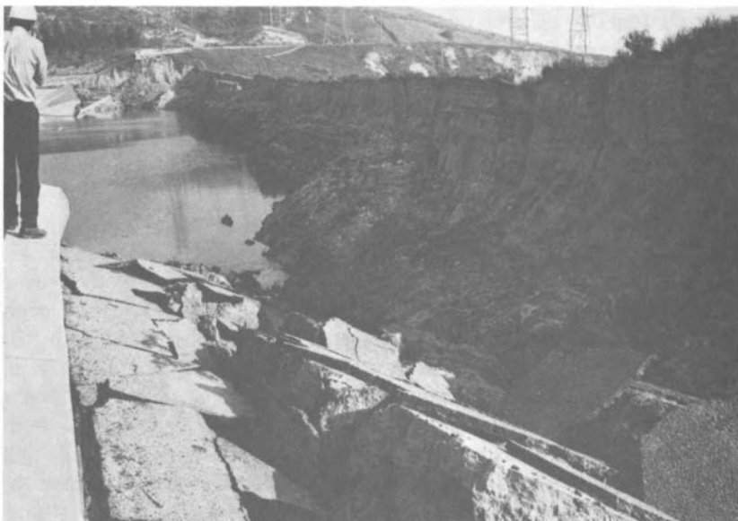
The upstream slope of the Lower San Fernando Dam slid beneath the water during the 1971 San Fernando earthquake, leaving just 4 ft of freeboard. This 140-ft-high earth dam was constructed prior to 1920 at a time when earthquake hazard was not considered.
