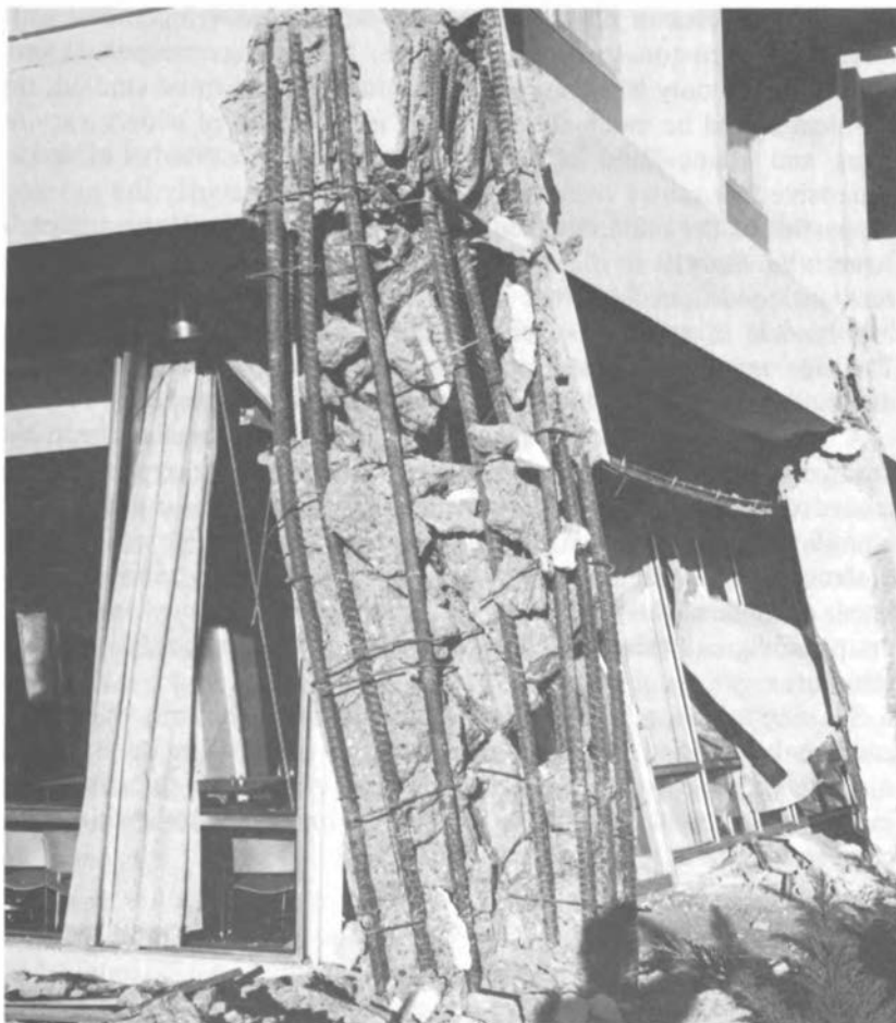
This reinforced column was shattered by earthquake forces. Research has developed methods of design that will prevent such columns from shattering.
