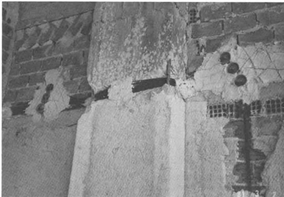
FIGURE 4.28 Conduits for electric cables pass through the column just inside the reinforcing bars and along the brick walls through channels chipped into the column and walls.
