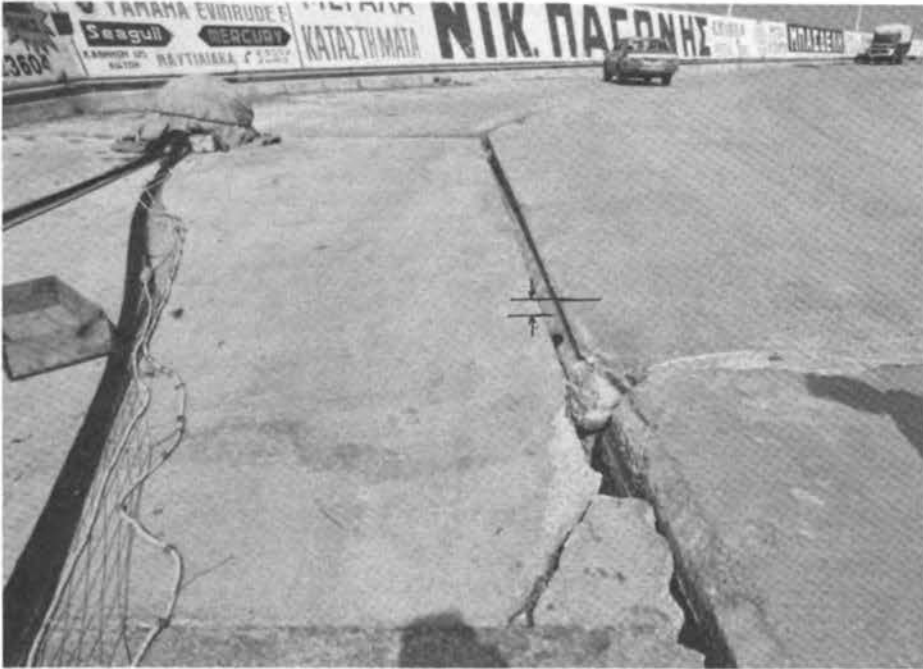
FIGURE 5.25 Jetty in Kiato. The expansion joints between the concrete blocks have been damaged. Note the differential settlement of about 20 to 30 cm.
