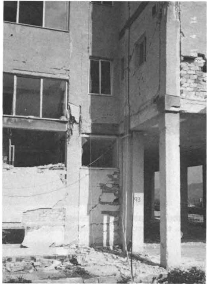
FIGURE 4.27 Typical damage of the column-to-beam connections in the block of flats in Loutraki. The lack of ties at the connections is common.
