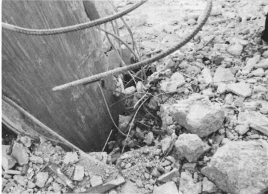
FIGURE 6.33 Apollo Hotel in Loutraki. The slabs sheared away from the column walls and came down one on top of the other.
