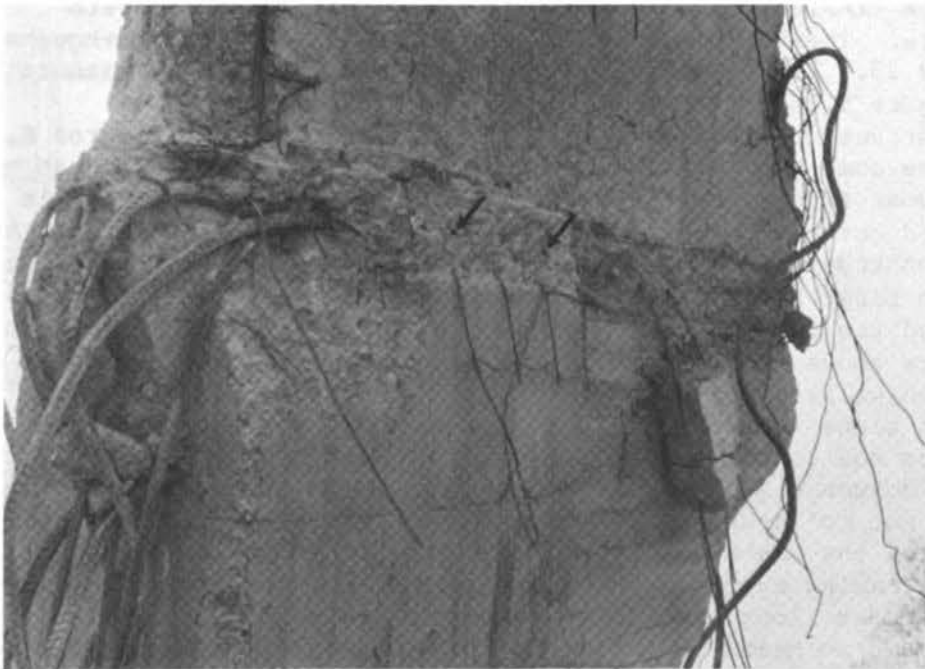
FIGURE 6.32 Apollo Hotel in Loutraki. Detail of the joint between shear wall and horizontal diaphragm. Note the slip of the horizontal reinforcing mesh wires of the slabs from the walls (arrows).
