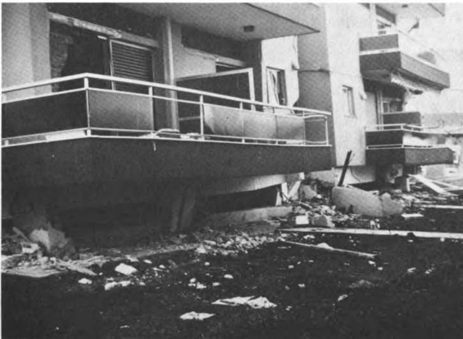
FIGURE 5.3 Failure of first-story columns.
