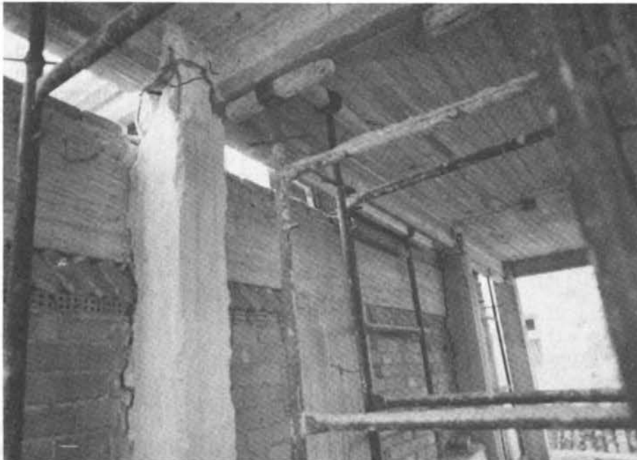
FIGURE 4.20 Hammer effect between two adjacent buildings not separated in Megara.
