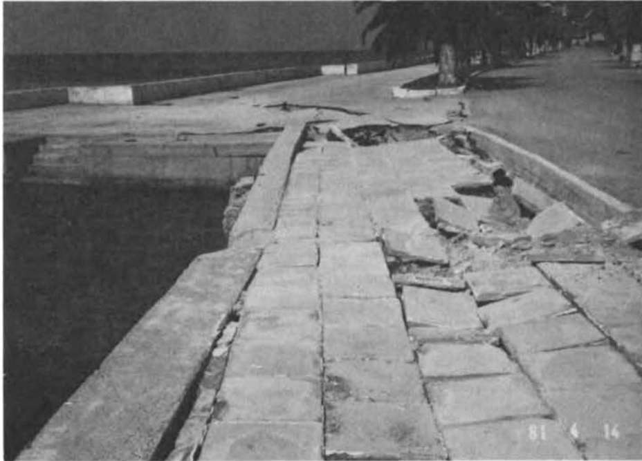
FIGURE 5.8 Quay wall in Loutraki. The earthen embankment has settled quite substantially.
