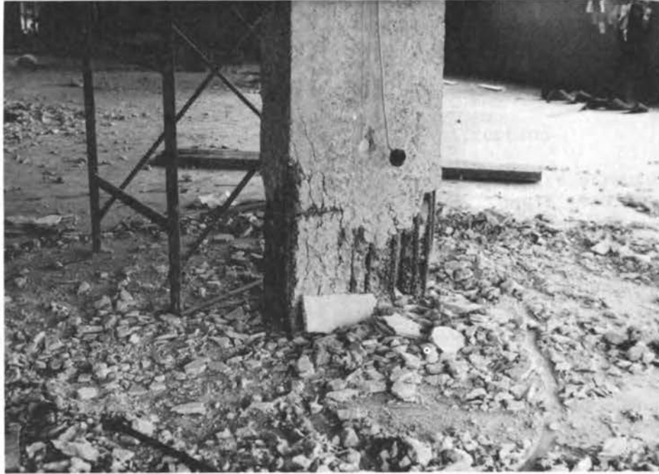
FIGURE 4.23 Poor quality concrete, too many bars, inappropriate aggregate gradation, and poor consolidation.
