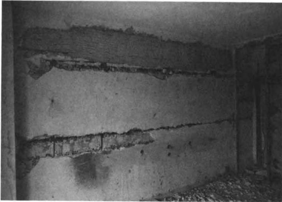
FIGURE 4.11 Brick wall reinforced by a concrete beam. The bricks under and over this beam as well as the ones at the top of the wall are crushed.
