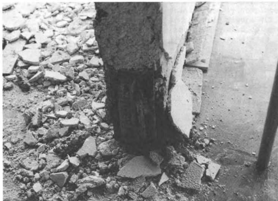
FIGURE 4.24 Poor detailing--too many steel bars appear in the lower part of the column. Most of the bars are from the lower story. The hooks opened and initiated the damage.
