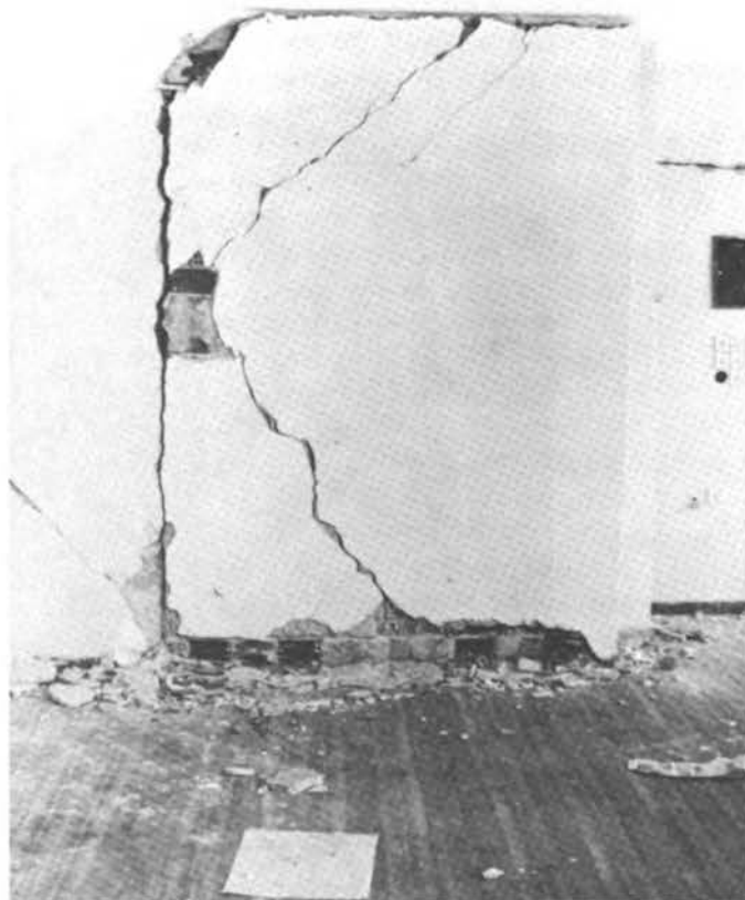
FIGURE 5.20 Infill wall damage.
