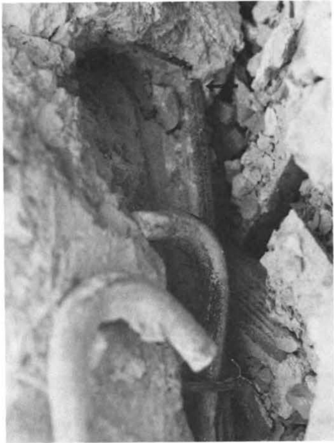
FIGURE 5.35 Detail of the collapsed hotel in Kineta. Note the slip of the hook and necking of the longitudinal bar (arrow).
