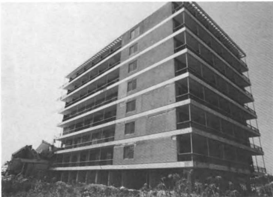
FIGURE 6.23 Galaxy Hotel in Vrahati. North view of section III. Columns and walls in the first floor were heavily damaged.
