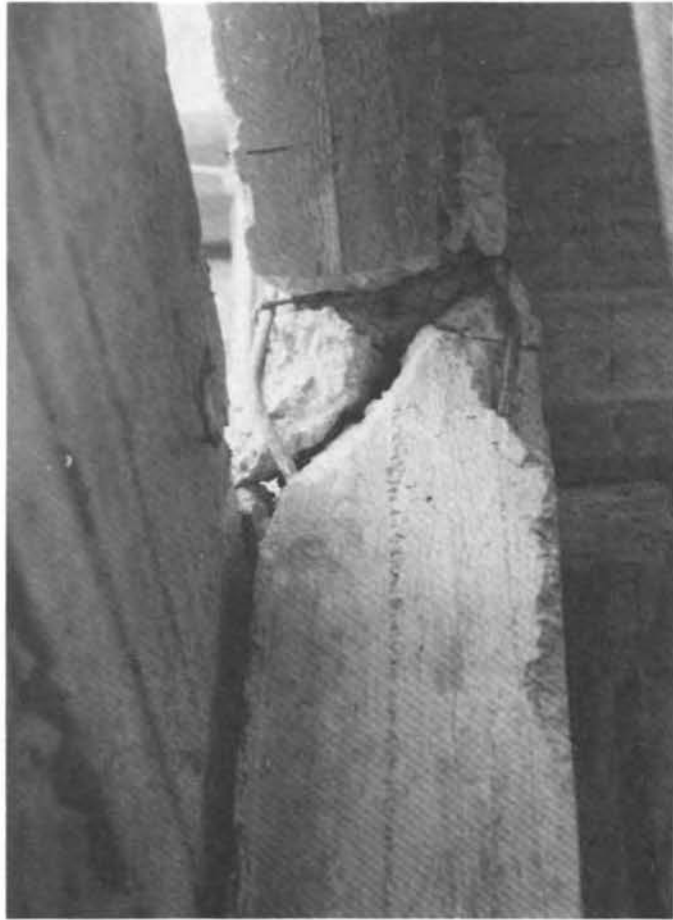
FIGURE 4.21 Detail of the damaged column in Figure 4.20. Note the gap between the two buildings after the earthquake.
