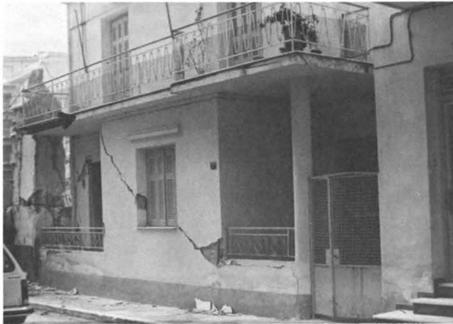
FIGURE 6.13 Contis Hotel in Loutraki. South view. A two-story building was located adjacent to the hotel. The arrow shows the excessive forces transmitted to this structure by the hotel during the rebound. Photograph courtesy A. Manis.
