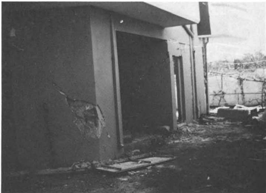
FIGURE 5.5 Failed wide column.
