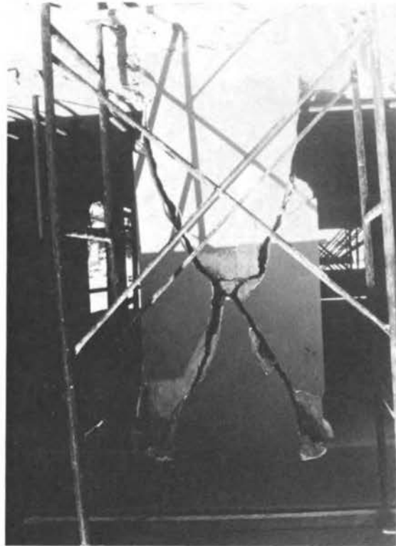
FIGURE 5.52 Heavily damaged stiff column at corner of apartment building shown in Figure 5.51.
