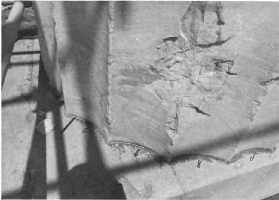
FIGURE 6.51 Lower part of the pillar at the southeast corner of the Parthenon. A clockwise rotation and displacement of the pillar to the east of about 1-2 cm was observed. Some fallen marble chips may be seen. Source: Dontas (1981).
