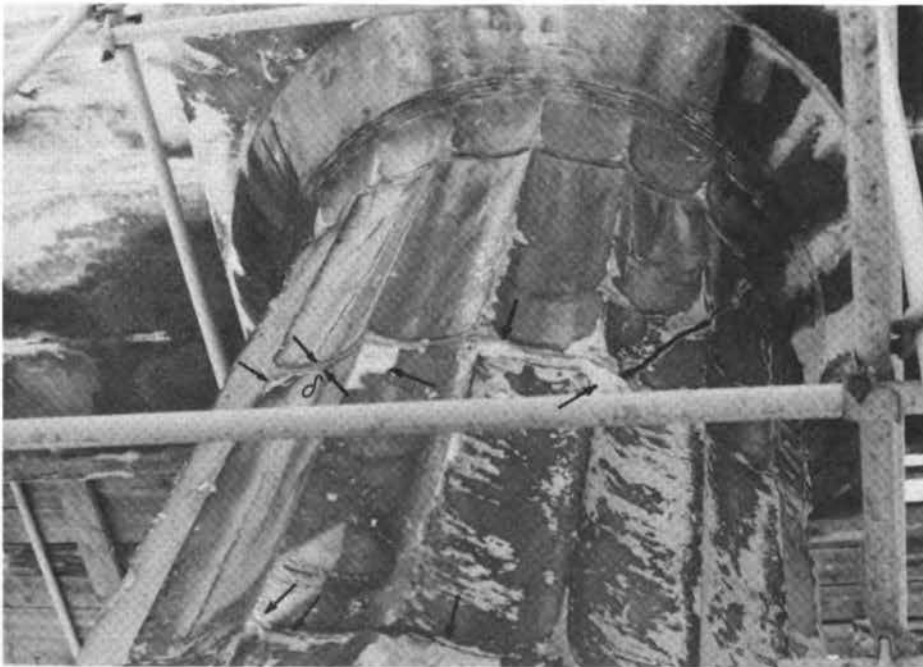
FIGURE 6.50 Upper part of the seventh pillar on the east side of the Parthenon. Arrows show spalling due to recent earthquakes. Source: Dontas (1981).
