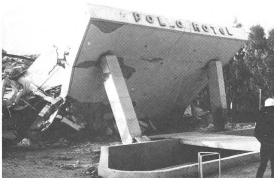
FIGURE 5.7 Collapse of Apollo Hotel in Loutraki.
