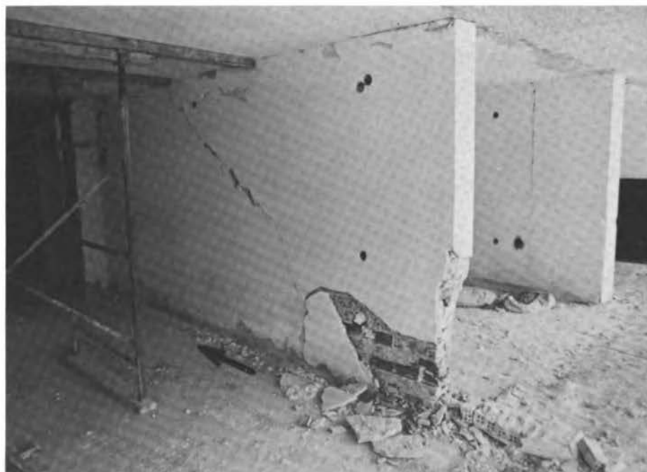
FIGURE 6.25 Galaxy Hotel in Vrahati. West view of the first story. The cracked walls are directed southwest to northeast.
