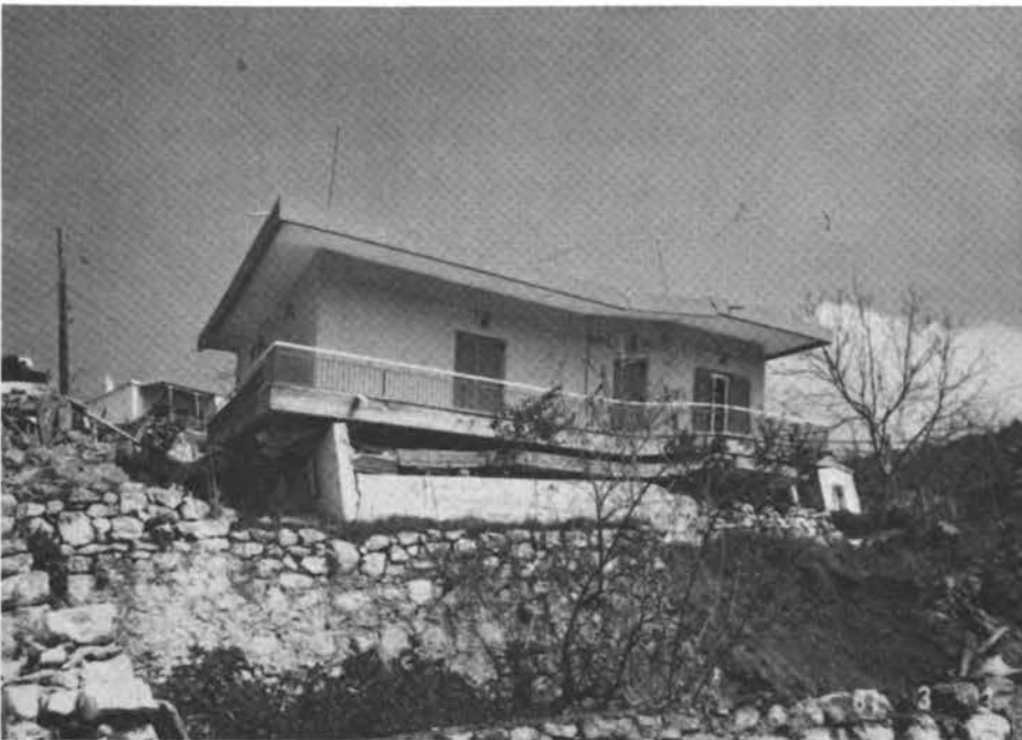
FIGURE 5.10 Damage to a three-story house built on sloping ground in Perahora. The retaining wall at the back of the house, which acts as a footing, functioned as the axis of rotation.
