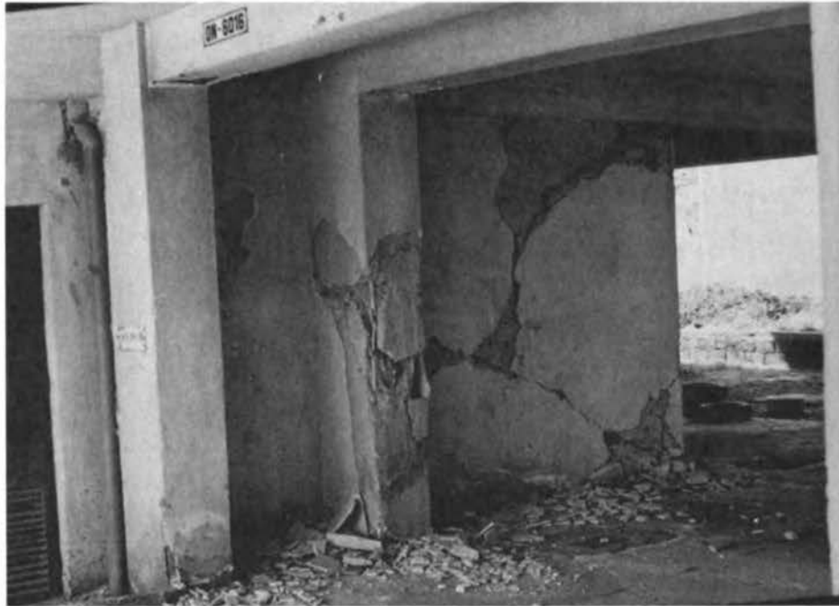
FIGURE 4.30 Typical shear failure of reinforced concrete column confined by a brick wall. The rupture of the masonry extends through the column.
