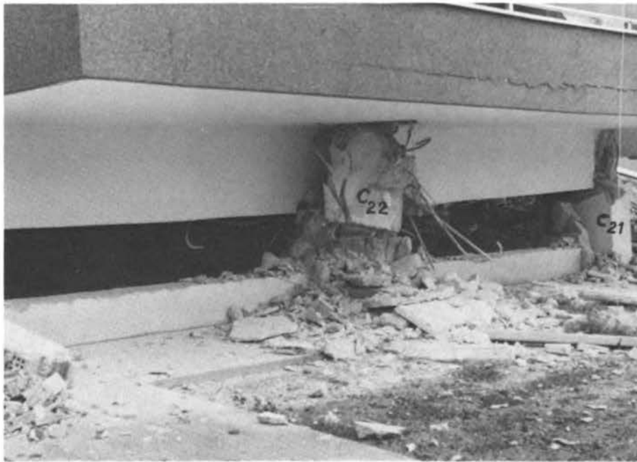
FIGURE 6.39 Block of Flats Segas in Loutraki. Columns c22 and c21 viewed from the north.
