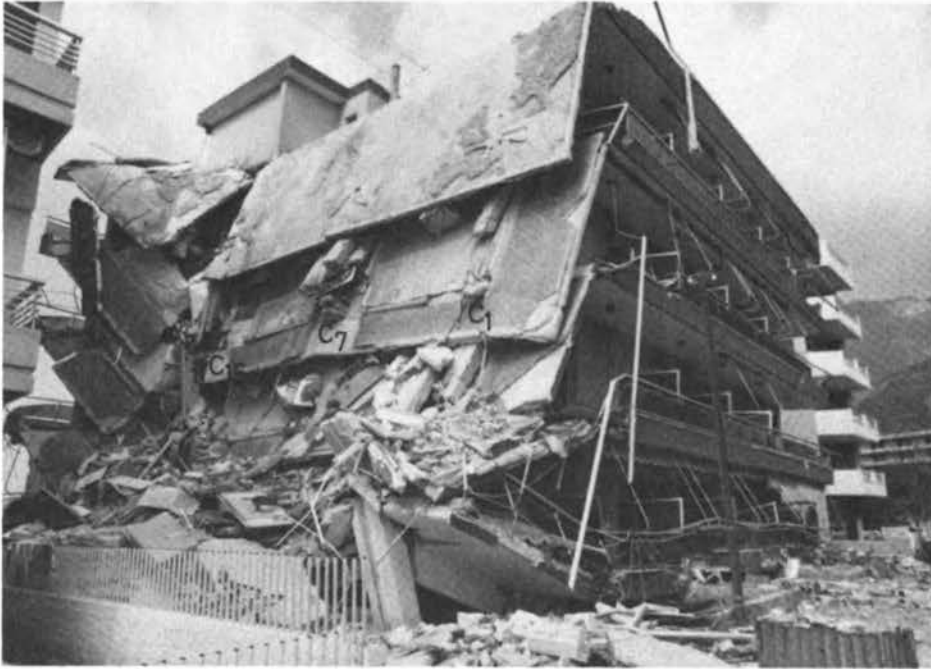
FIGURE 6.36 Block of Flats Segas in Loutraki. The structure from the southeast.
