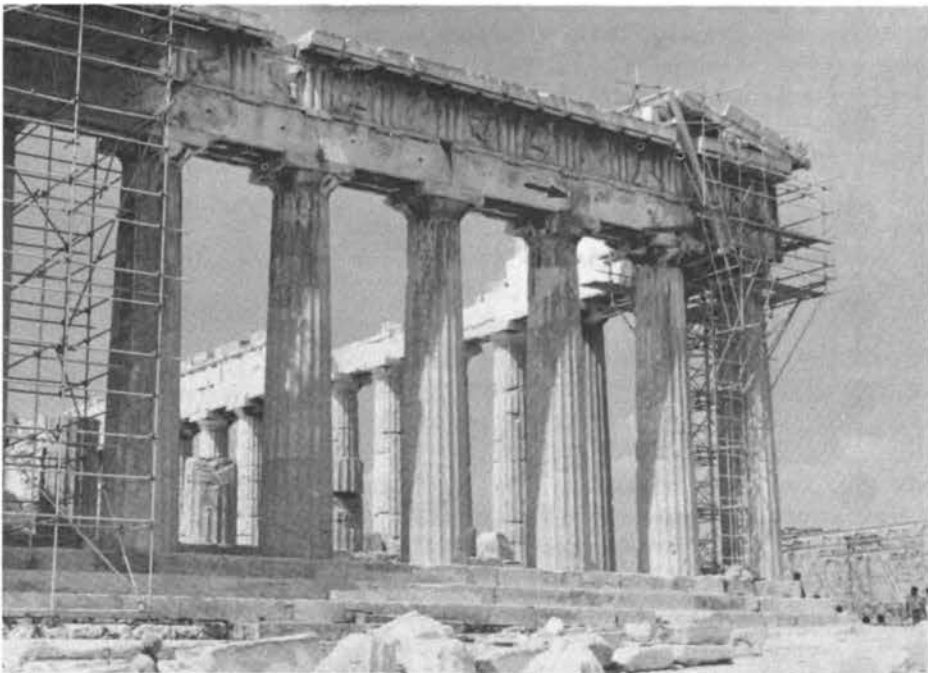
FIGURE 6.44 East view of the Parthenon. The arrow indicates a large crack in the head beam over the third pillar. There are also large cracks in the head beam between the first and second pillars.
