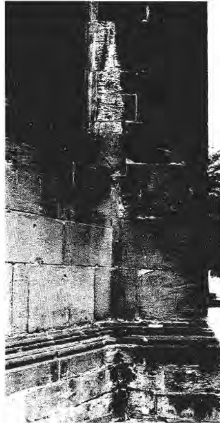
FIGURE 4 Freiburg Cathedral, West Germany, east wall, with lime crust (calcite) from joint near window covering honeycombs in sandstone.
