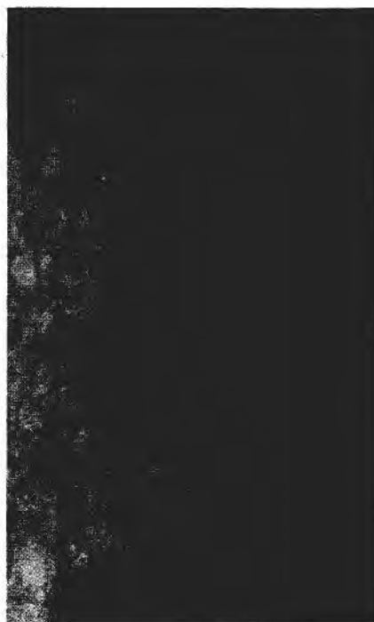
FIGURE 6 Detail of weathered protruding rib showing dislodged calcite grains and vertical cracks at the Field Museum of Natural History, Chicago. Scale in millimeters.
