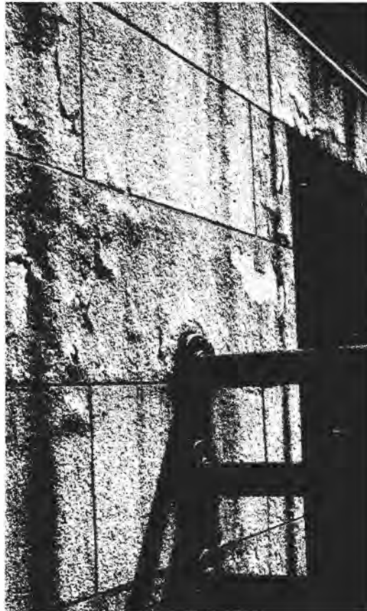
FIGURE 10 Granite surface stone in the lower course of a New York City landmark building has been subjected to the action of salt used in de-icing the adjacent street. The surface has lifted up in numerous places, forming blisters with a layer thickness that ranges from 0.5 to 1.5 mm.
