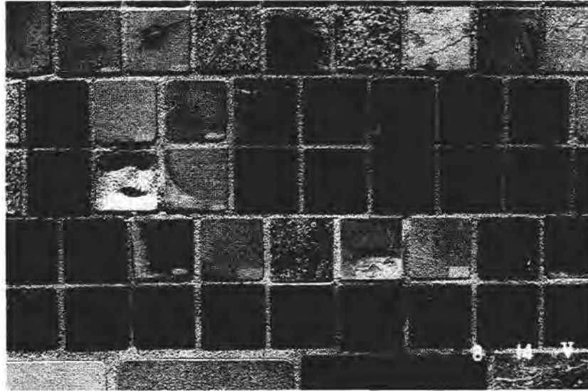
FIGURE 3 NBS stone test wall (see Figure 2), detail section. Some sandstones show weathering, discoloration, and salt efflorescence.
