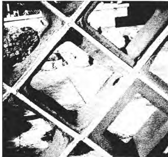
FIGURE 5 Salt disintegration of solar screen tile in Miami Beach, Florida.
