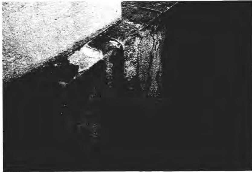
FIGURE 9 Strong flaking on granite at the base of Tweed Court House, lower Manhattan, New York.
