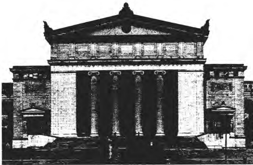
FIGURE 5 Field Museum of Natural History, Chicago, south entrance. Photo shows deep weathering and vertical cracks that have developed along ribs on columns.
