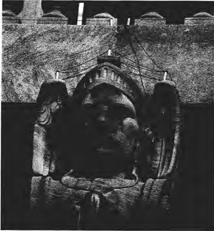
FIGURE 4 The Federal Building (Dept. of the Post Office Bldg.) Sculptor: A. A. Weinman? (1934?). Esthetic effects of antipest devices may be counterproductive.
