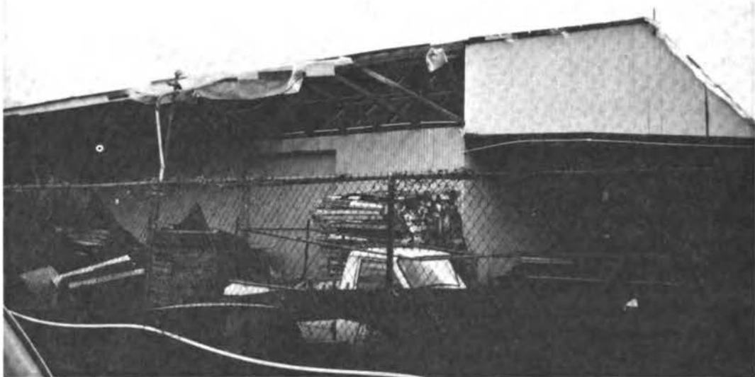
FIGURE 3.7 Damage to warehouse building, Kauai.
