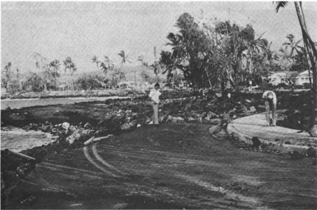
FIGURE 3.16 Undermined and destroyed section of Hoone Road at Poipu Beach, Kauai.
