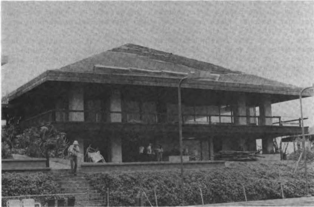
FIGURE 3.72 Wind damage to roof of Bali Hai Restaurant, Princeville, Kauai.
