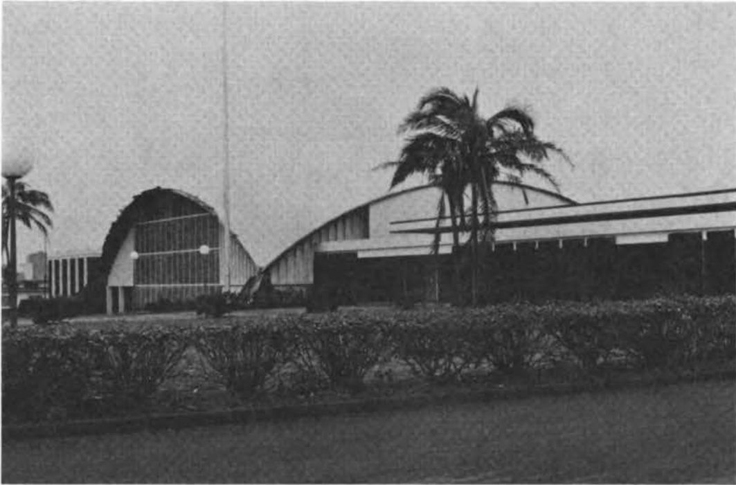
FIGURE 3.51 Convention Center at Lihue, Kauai (note minor damage to roof flashing at rake; some glass breakage occurred due to windborne debris).
