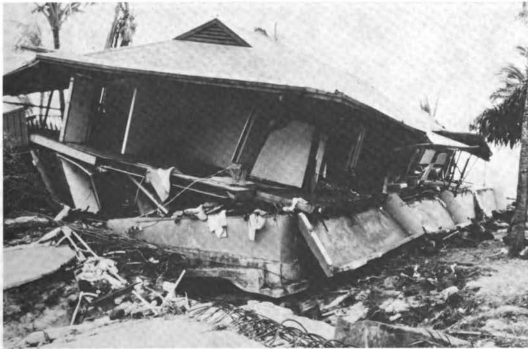
FIGURE 3.26 Damage to timber-framed unit at Sheraton-Kauai.
