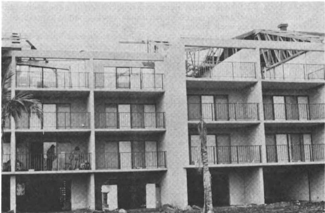
FIGURE 3.33 Wind damage to Prince Kuhio Condominium, Kauai (note geometric discontinuity in roof).
