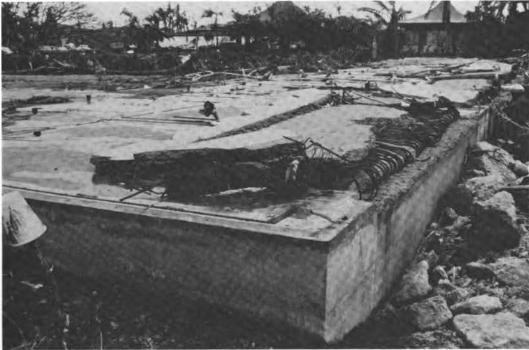
FIGURE 3.25 Remains of two-story hotel unit at Sheraton-Kauai (note lanai slab bent backwards 180 degrees).
