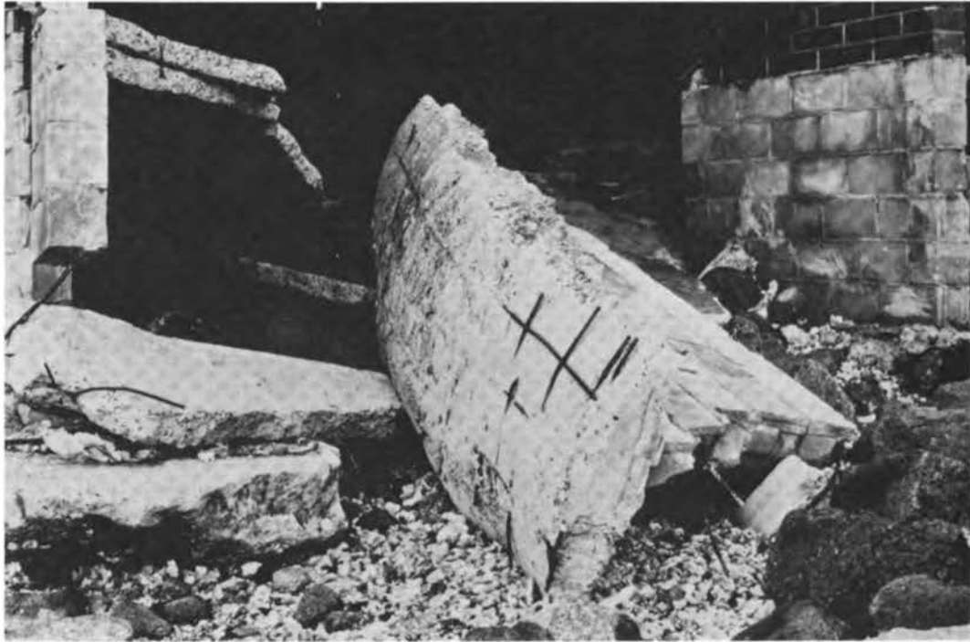
FIGURE 3.23 Damage to footing, Kuhio Shores Condominium, Kauai.
