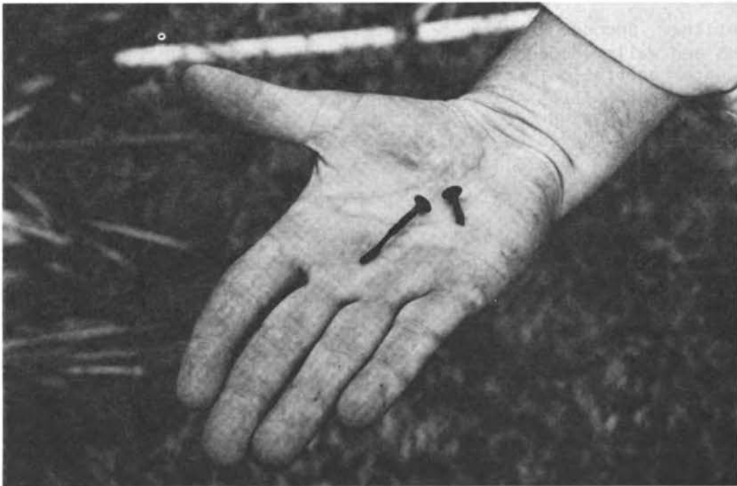
FIGURE 3.46 Corrosion of metal fasteners used to attach light-gage metal sheeting.
