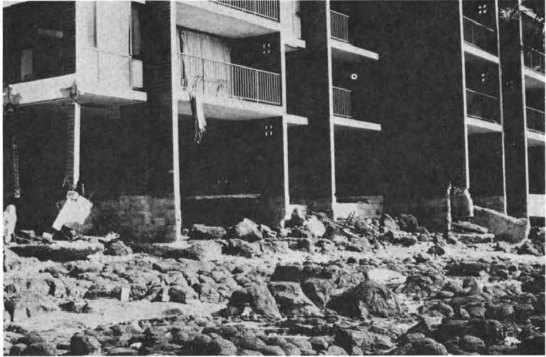
FIGURE 3.19 Damage to Kuhio Shores Condominium, Kauai (note scouring of footings).
