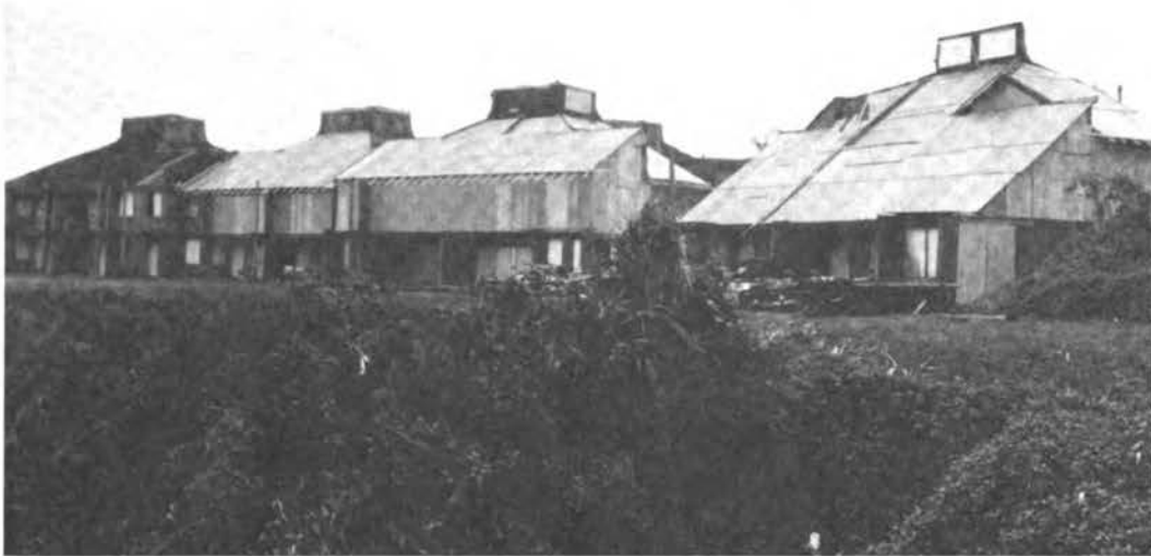
FIGURE 3.65 Damage to townhouses at Pali Ke Kua, Princeville, Kauai (note high percentage of glazed areas in damaged walls).
