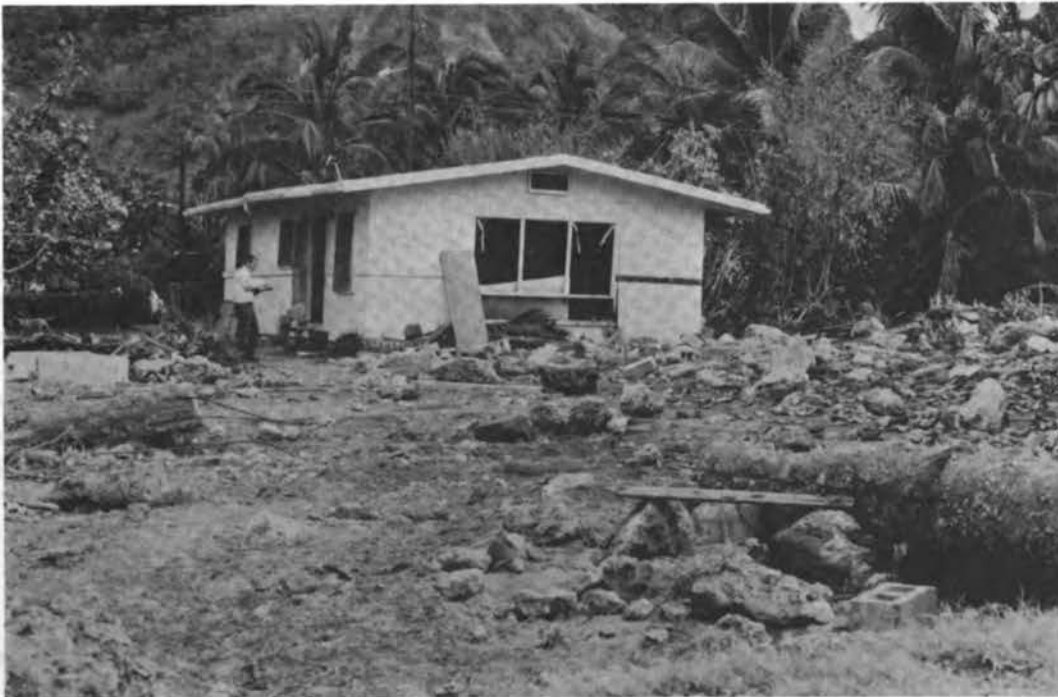
FIGURE 3.4 Damaged beachfront residence at Makaha, Oahu (note that home was transported off concrete slab foundation 100 yds inland by storm surge and wave action).
