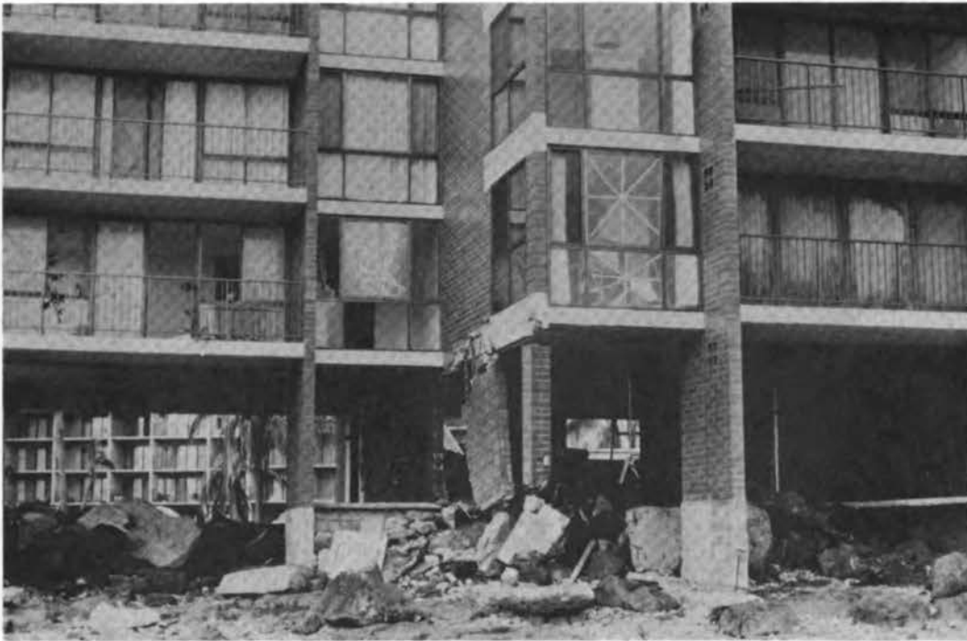
FIGURE 3.21 Damage to bearing walls of Kuhio Shores Condominium, Kauai (note large boulders transported to interior of building by storm surge and wave action).
