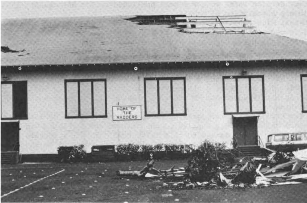
FIGURE 3.47 Wind damage to Kauai High School gymnasium.
