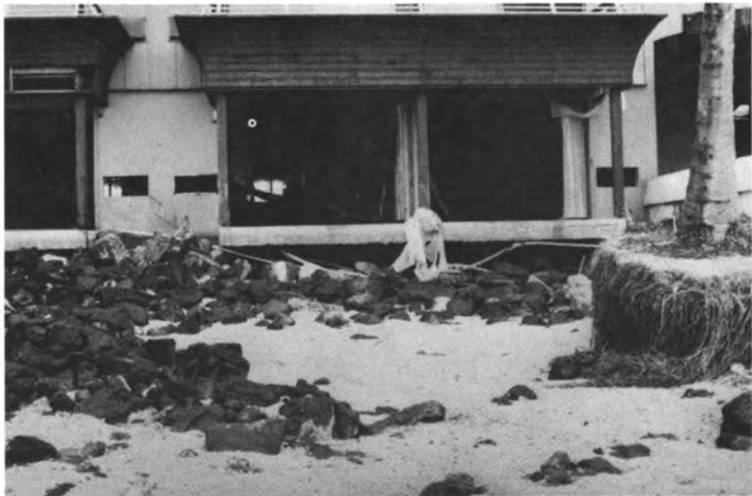
FIGURE 3.28 Erosion of footings of three-story unit at Sheraton-Kauai.
