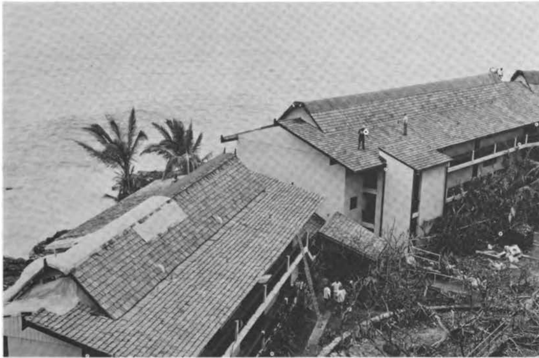
FIGURE 3.38 Cladding damage to condominiums at Makahuena Point, Kauai.
