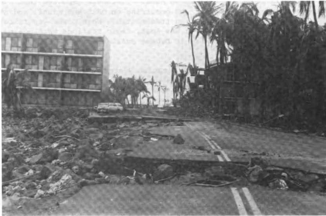
FIGURE 4.9 Severely damaged coastline road at Hoai Bay in the Poipu area of Kauai.
