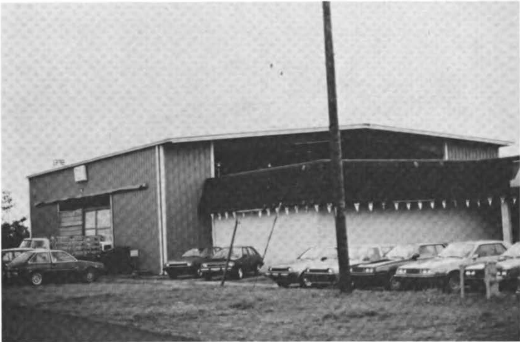
FIGURE 3.11 Damaged preengineered metal building at Kauai (note natural ventilation built into windward wall).
