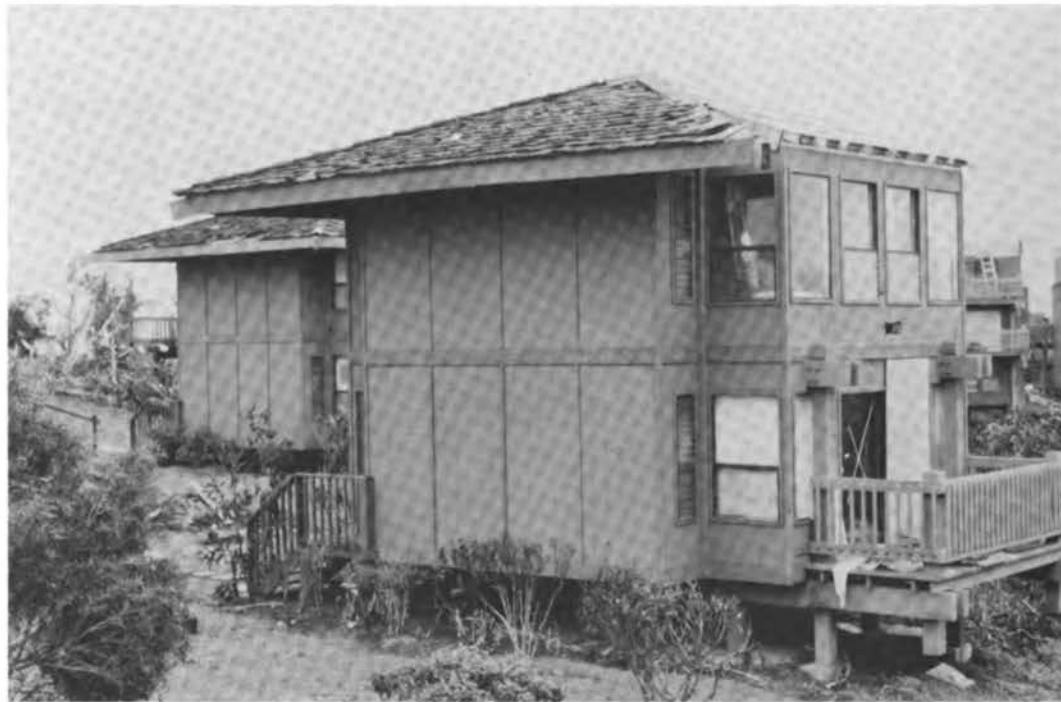
FIGURE 3.68 Damage to Hanalei Bay Villas on windward wall.
