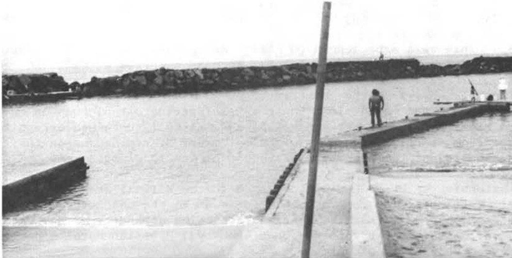
FIGURE 3.73 Storm surge and wave damage to Pokai Bay breakwater, Oahu.
