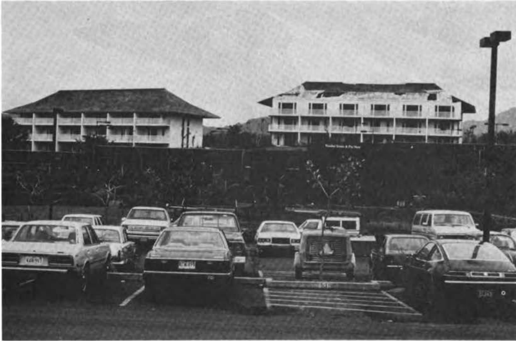
FIGURE 3.34 Roof damage to building inland from Poipu Beach, Kauai.
