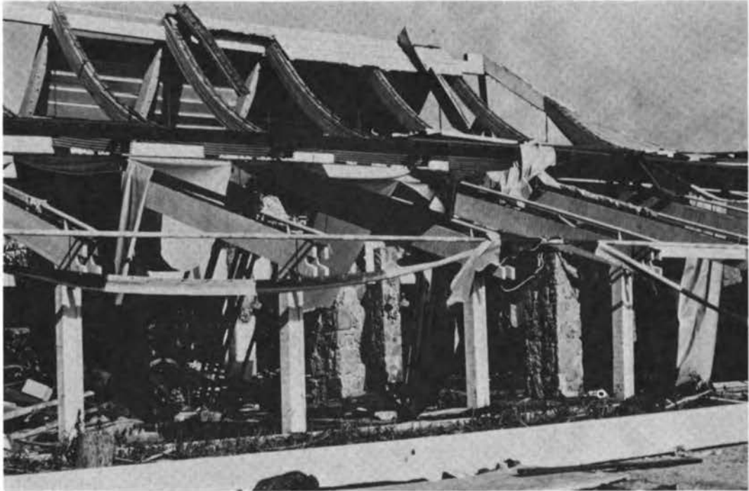
FIGURE 3.27 Flooding and wind-induced damage to Drum Lounge at Sheraton-Kauai.
