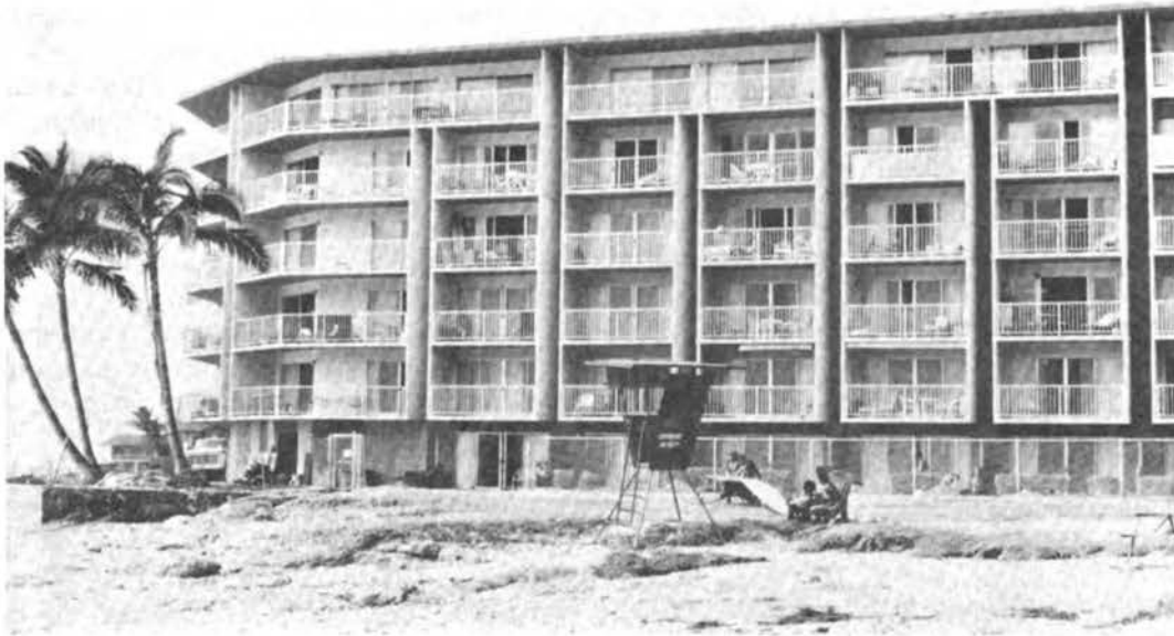
FIGURE 3.75 Water and wave damage to Makaha Shores Condominium, Oahu.
