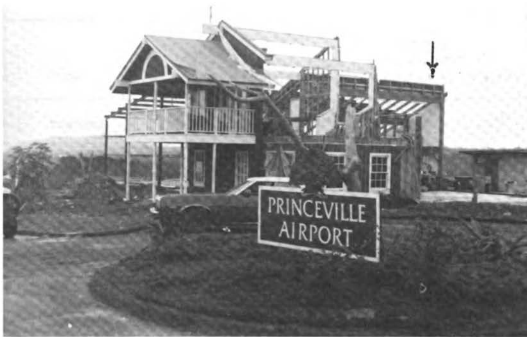
FIGURE 4.10 Partially destroyed aircraft hangar at Princeville Airport at Hanalei, Kauai.
