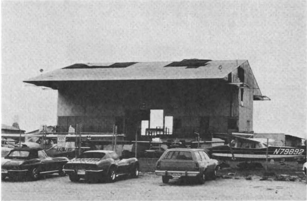
FIGURE 3.79 Old metal hangar building at Honolulu International Airport (note large portions of missing roof cladding).
