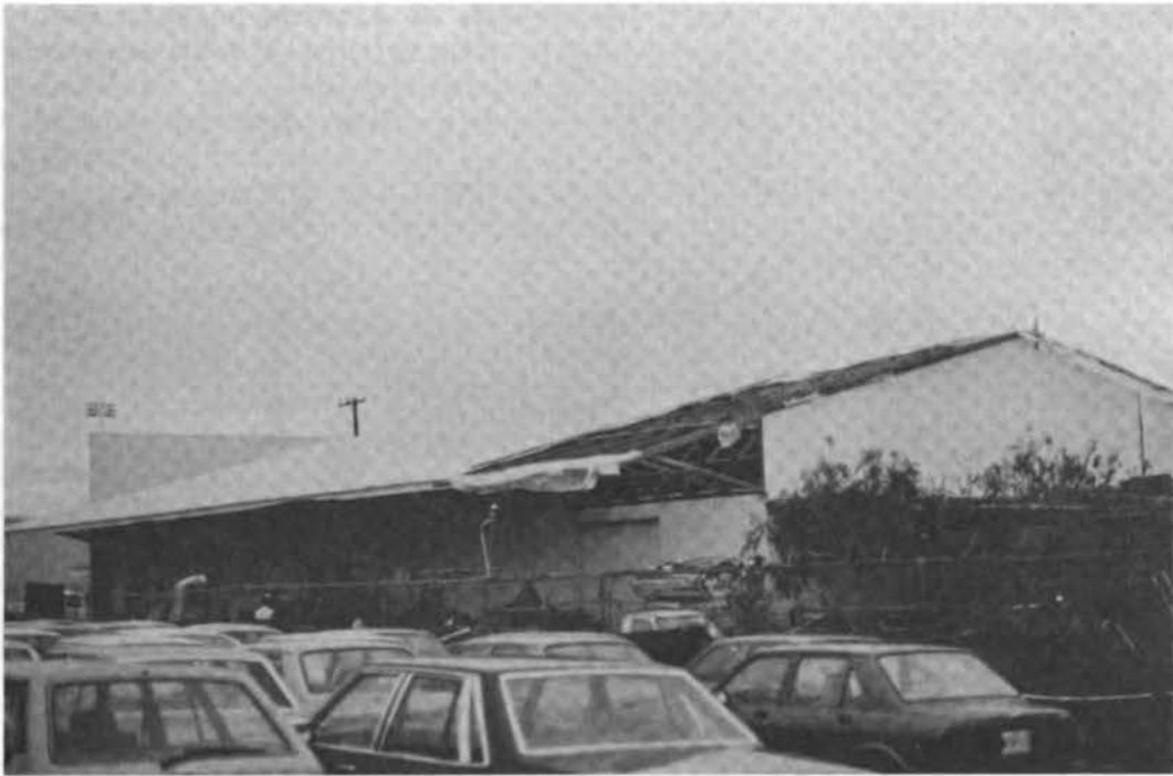
FIGURE 3.54 Damaged timber-framed warehouse building at Lihue, Kauai.
