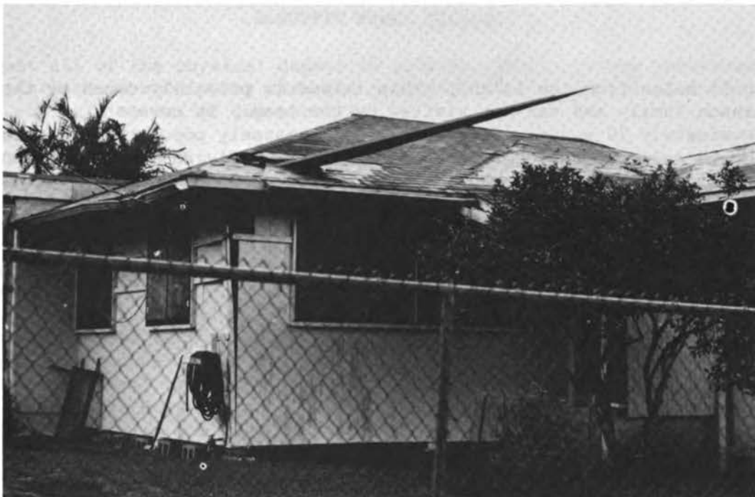
FIGURE 3.85 Missile damage to roof of residence at Kaneohe, Oahu.
