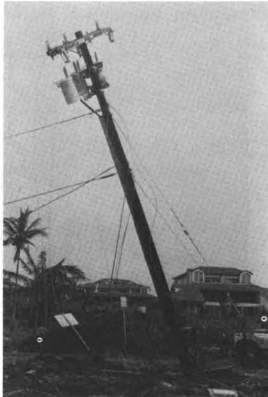
FIGURE 4.4 Power pole at Poipu, Kauai, that failed due to pole rupture at ground level.
