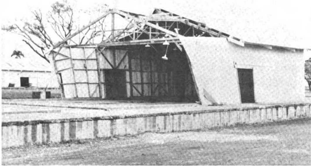
FIGURE 3.9 Damage to timber-framed building clad with light-gage metal sheeting (note that most of the damaged building had been removed at the time the photograph was taken).
