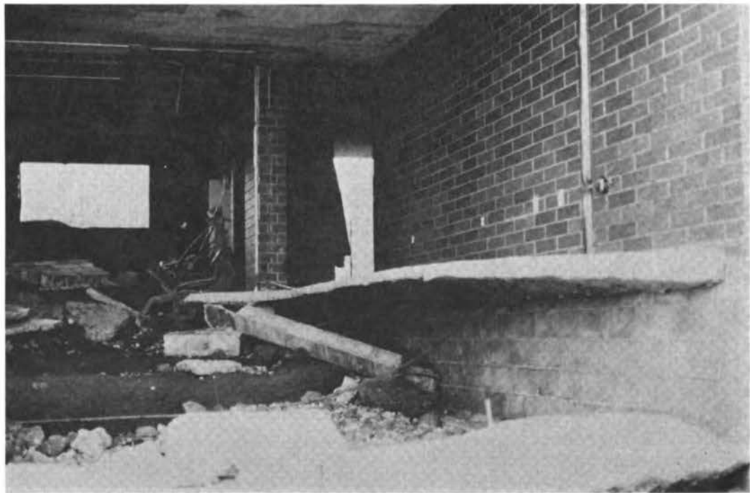
FIGURE 3.20 Damage at first-floor level of Kuhio Shores Condominium, Kauai (note variable thickness of floor slab and reinforcing steel exposed at bottom of slab).
