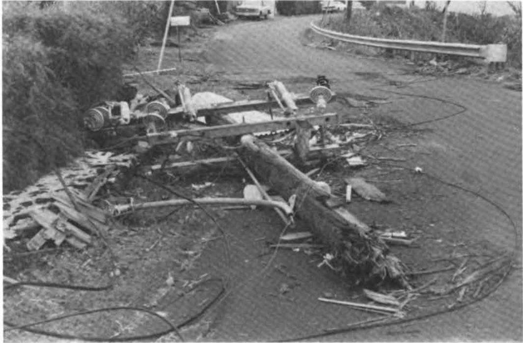
FIGURE 4.5 Power pole above Makahuena Point, Kauai, that failed at mid-pole height.
