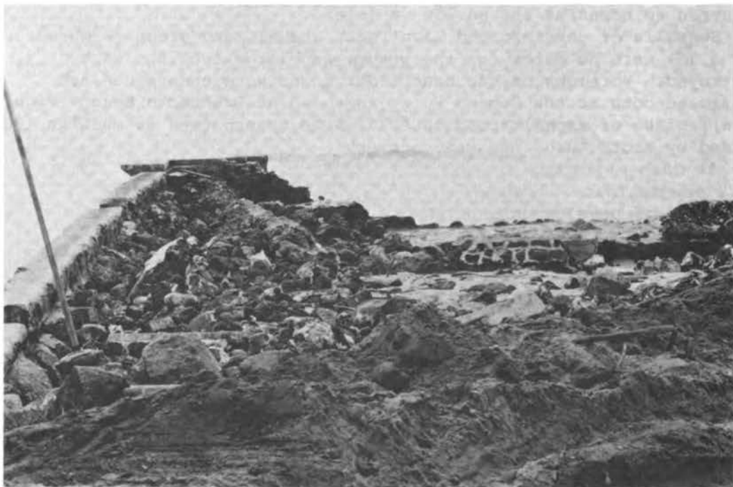
FIGURE 3.14 Damage to seawall at Poipu Beach, Kauai.
