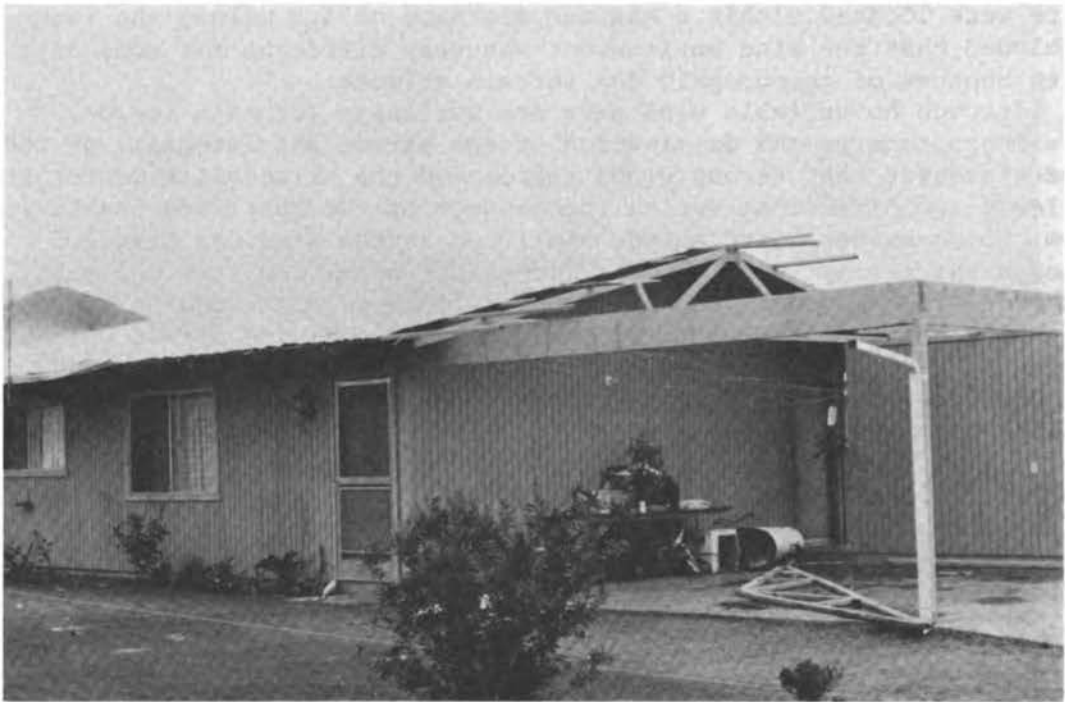
FIGURE 3.58 Loss of carport roof at Kapaa Meadows, Kauai.
