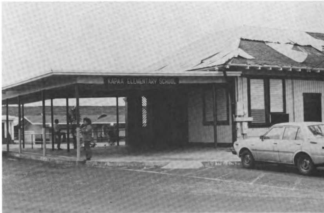
FIGURE 3.56 Damage to roof covering of Kapaa Elementary School (note light-gage corrugated metal sheeting nailed over existing roof).
