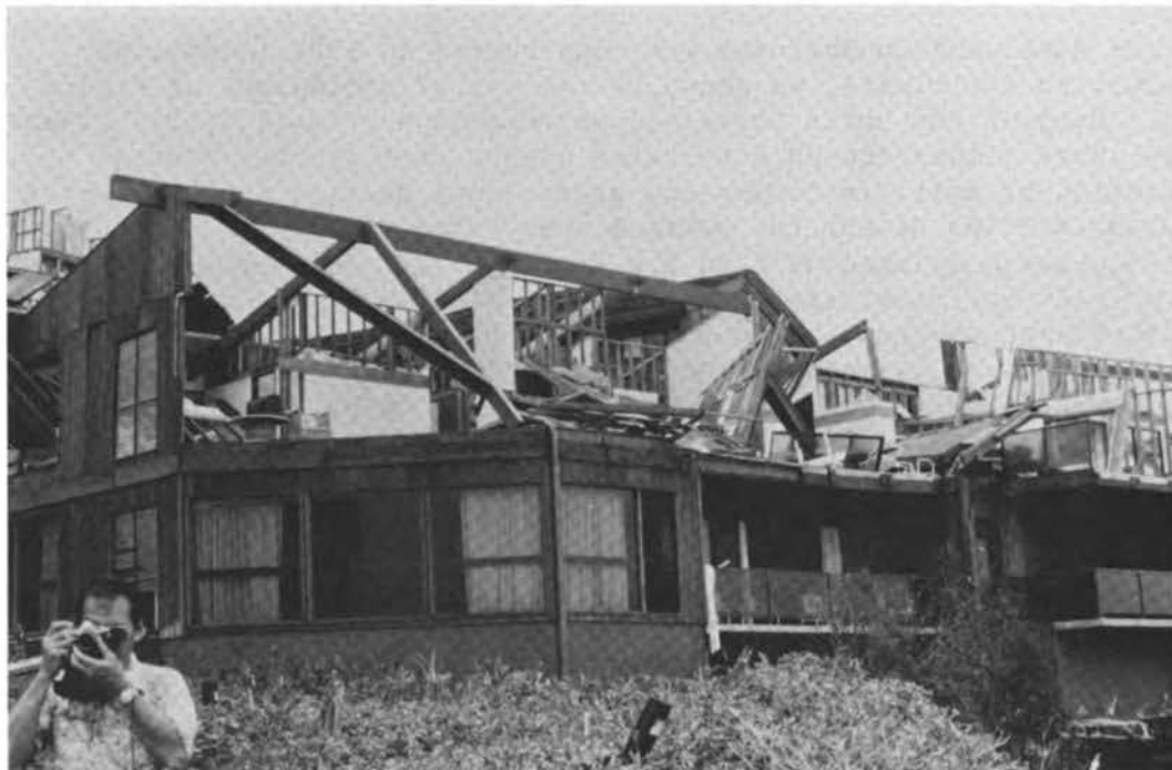
FIGURE 3.43 Wind damage to Makahuena Point Condominiums, Kauai.
