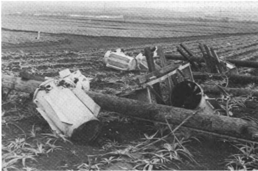
FIGURE 4.6 Pole-mounted transformers and circuit breakers damaged when wind-driven building debris knocked over a pole-supported customer substation near Kunia, Oahu.
