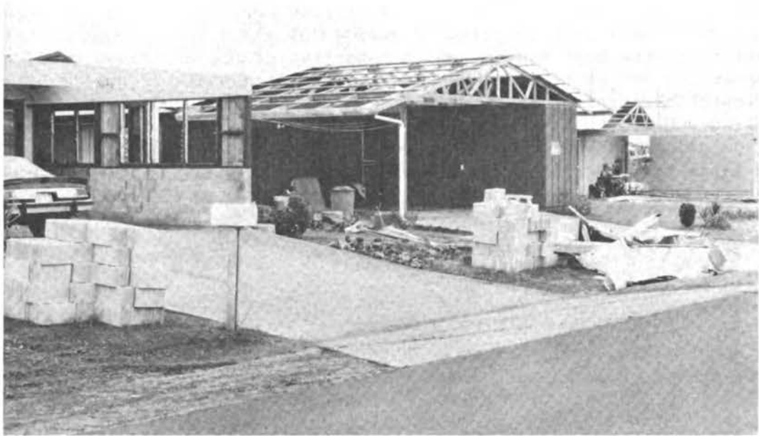
FIGURE 3.57 Damage to roof covering of single-family dwelling at Kapaa Meadows, Kauai.
