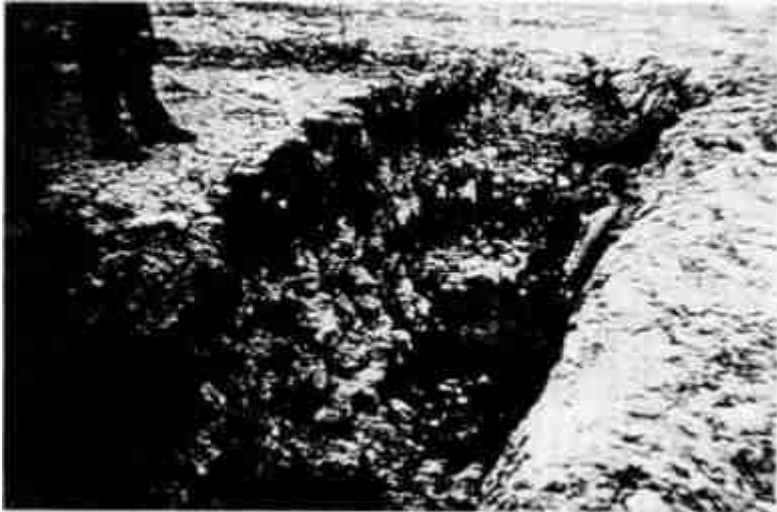
Figure 5-11 Erosion caused by seepage through floor of Helena Valley Reservoir.
