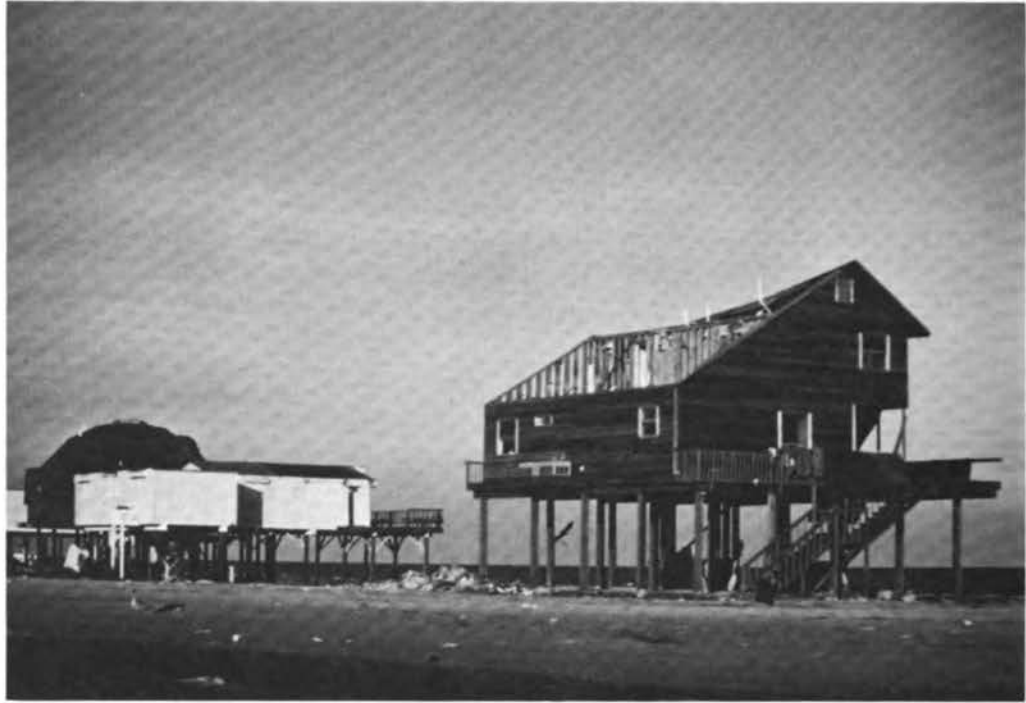
FIGURE 4.39 Example of a roof failure of a house in Terramar Beach.
