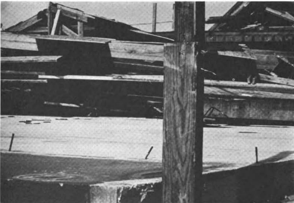
FIGURE 4.60 House washed away from its foundation slab by storm surge.
