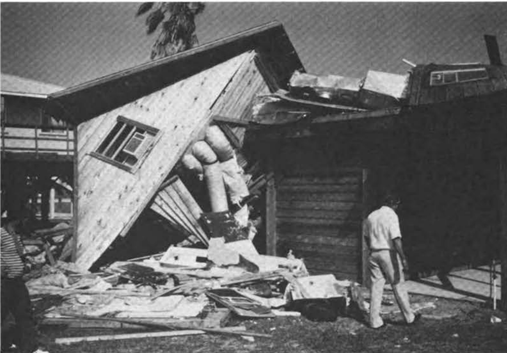
FIGURE 4.48 Typical example of poor connections between sub-systems.
