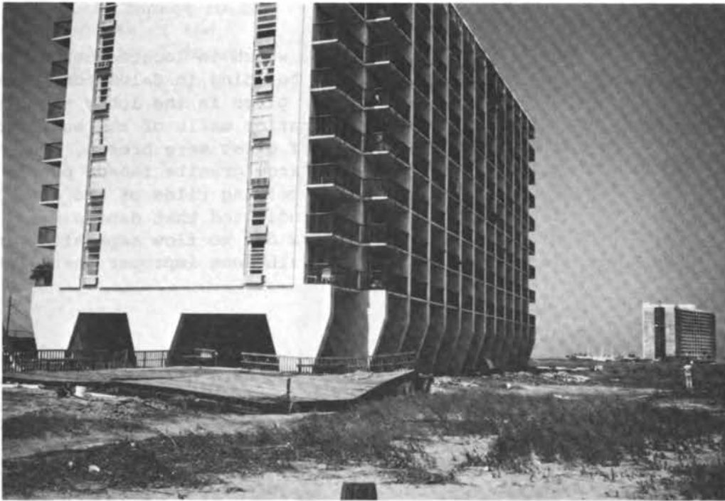
FIGURE 4.19 General erosion and damaged deck around Islanders Inn and the Galvestonian (in the background).
