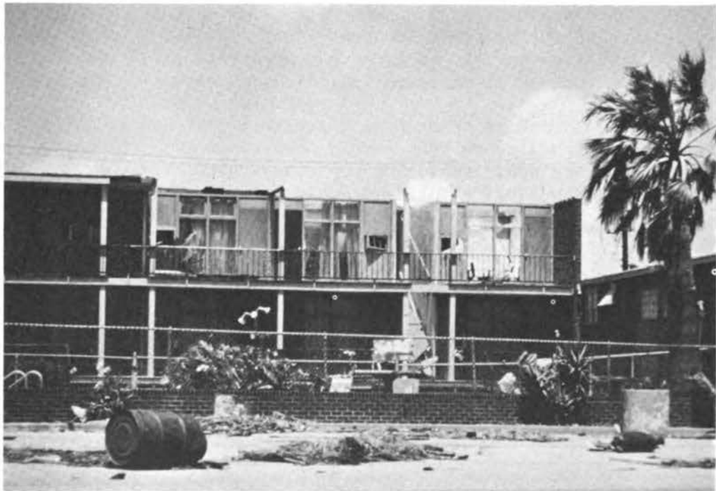
FIGURE 4.35 Partial loss of roof at a motel.
