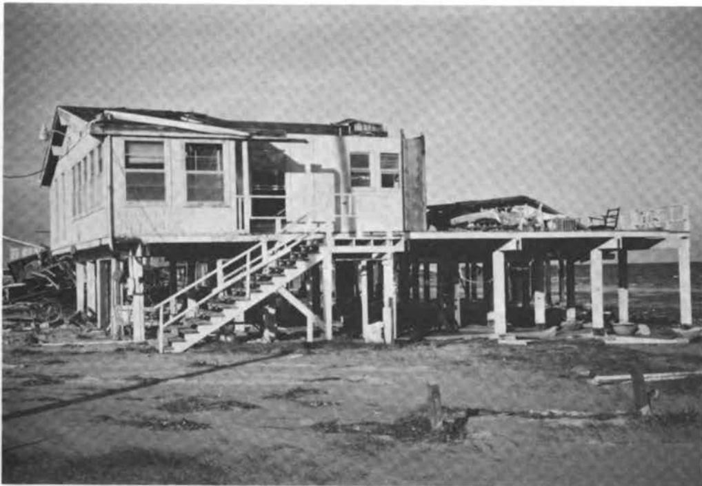
FIGURE 4.42 Typical example of partial collapse of a large house in Terramar Beach.
