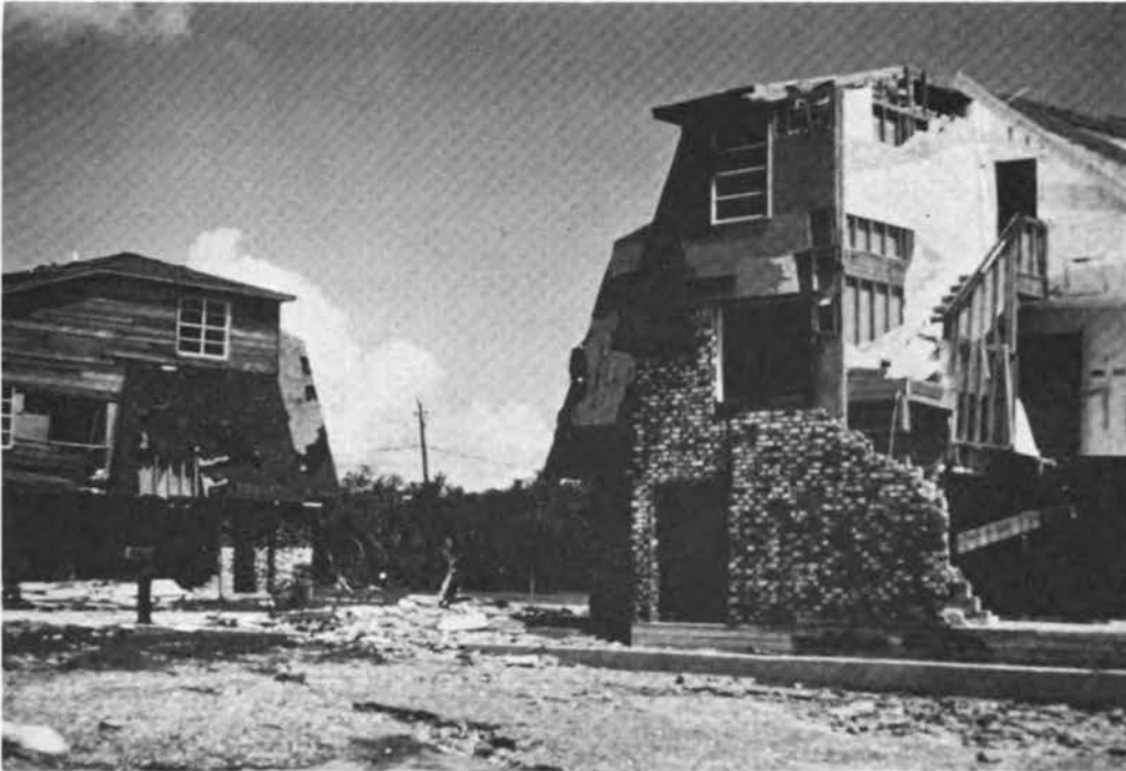
FIGURE 4.59 Failure of the roof and brick veneer wall of a condominium.
