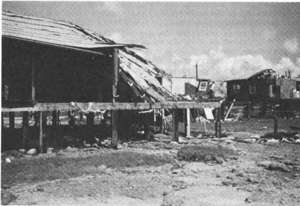
FIGURE 4.58 Bayfront house with a collapsed roof.
