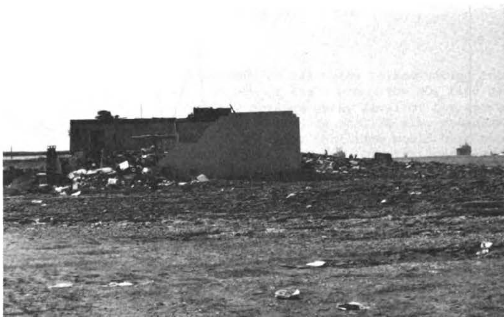
FIGURE 3.4 Scour and building damage near the intersection of the Galveston seawall and the west jetty of Galveston Inlet.
