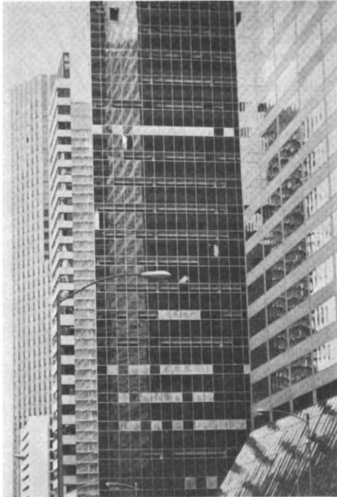
FIGURE 4.9 Glass damage to the northeast face of the Entex Building.
