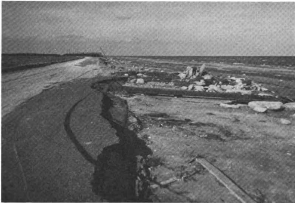
FIGURE 5.1 Typical washout of shoulder on San Luis Pass Road, Follets Island.
