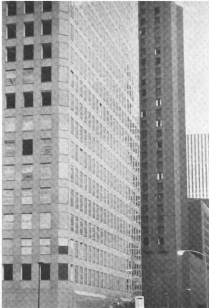
FIGURE 4.7 Window damage to the Hyatt Regency Hotel (the building in the background).
