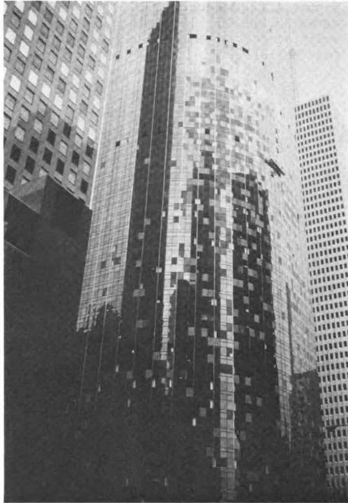
FIGURE 4.3 Glass damage on the southwest face of the Allied Bank Building. Dark shapes are reflections of adjacent buildings.
