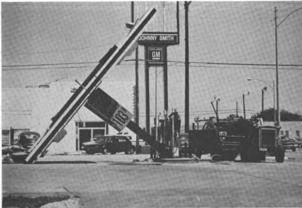
FIGURE 4.15 Example of failure of a roof support pedestal column.
