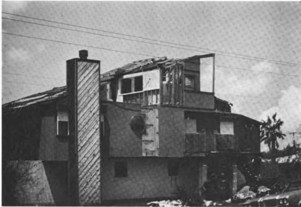
FIGURE 4.63 Roof damage to a condominium in Texas City.
