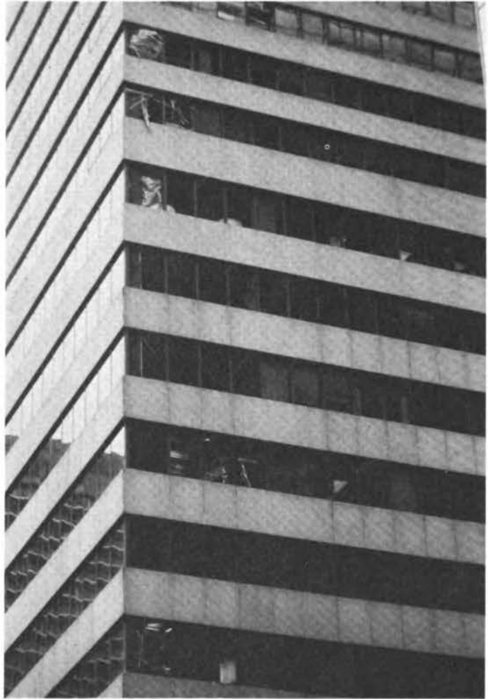
FIGURE 4.10 Window damage to the Sheraton-Houston Hotel.
