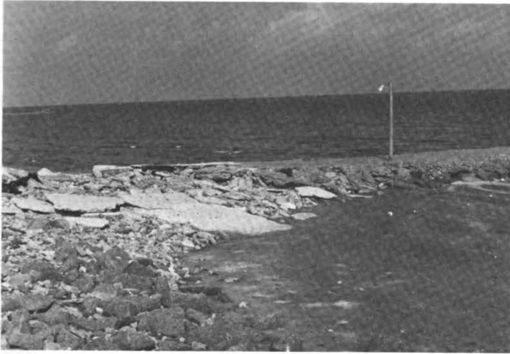
FIGURE 4.55 Damage to groin in front of the Galveston seawall.
