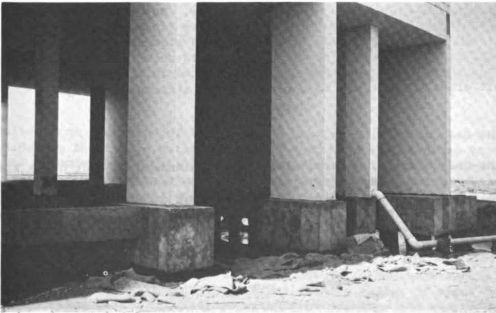
FIGURE 4.20 Erosion around the foundation of the Galvestonian.
