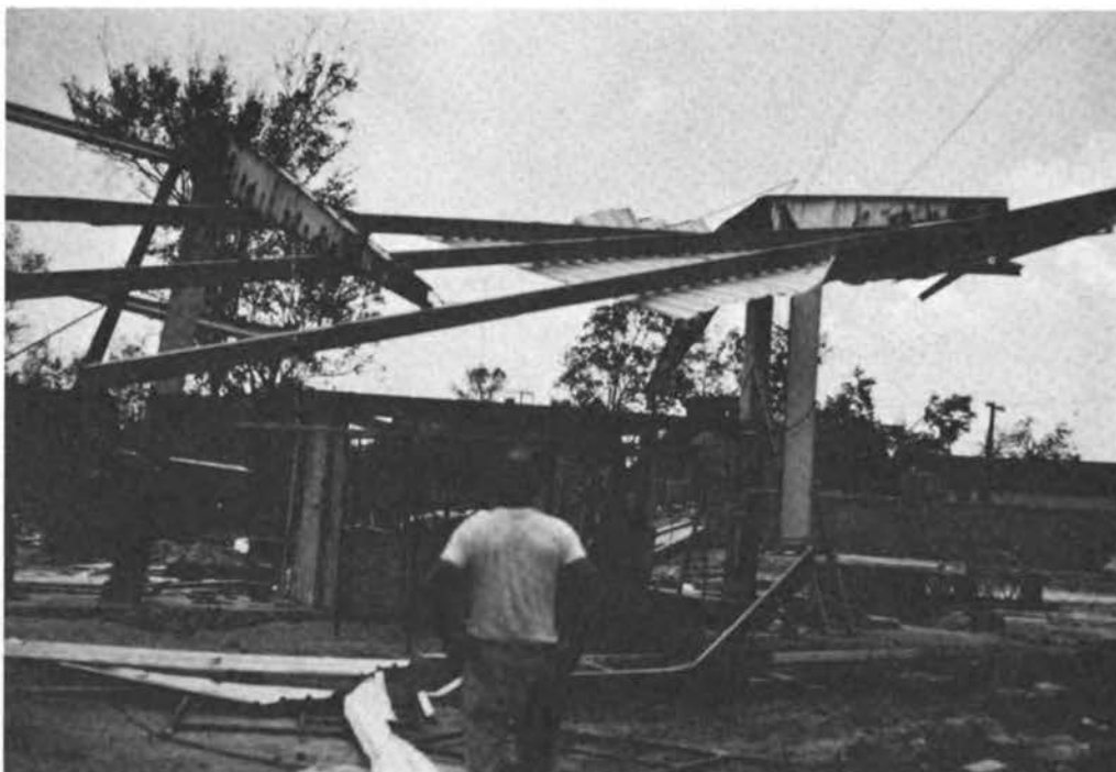
FIGURE 4.16 Failure of sheet metal roof at a gas station.
