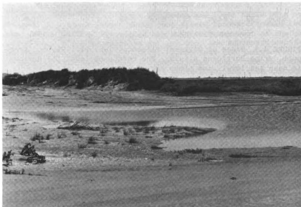
FIGURE 3.5 Front of scour channel and frontal dune on East Beach showing dune erosion. Scour channel was caused by flow confined between the dune and an adjacent beachfront condominium.
