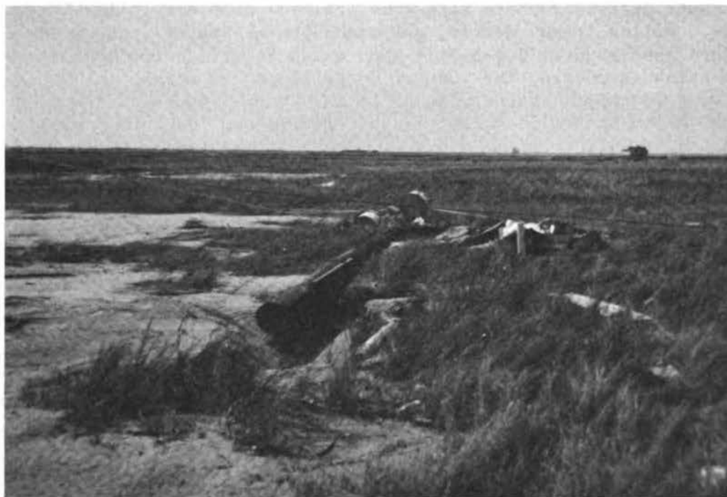
FIGURE 5.4 Typical failure of transformer pole on East Beach, Galveston Island.
