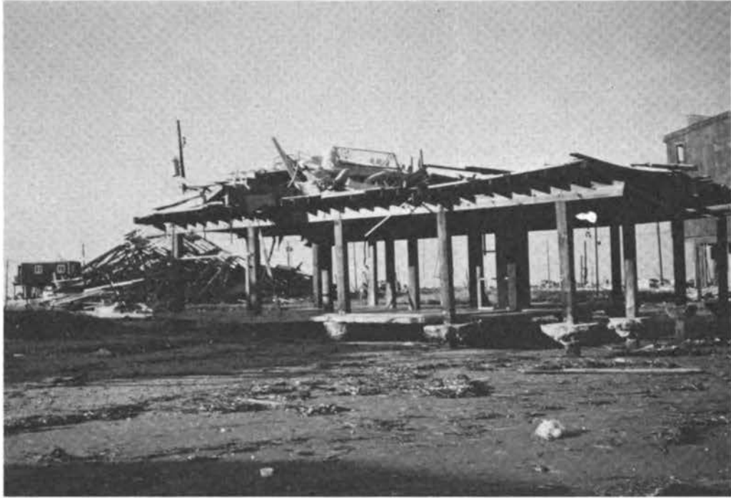
FIGURE 4.43 Example of a superstructure blown away by the wind. A mound of lumber, furniture, and appliances is in the backyard of the house.
