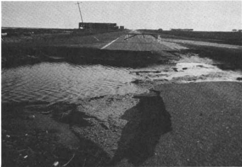
FIGURE 5.3 Total washout of shoulder and road on San Luis Pass Road, Follets Island.
