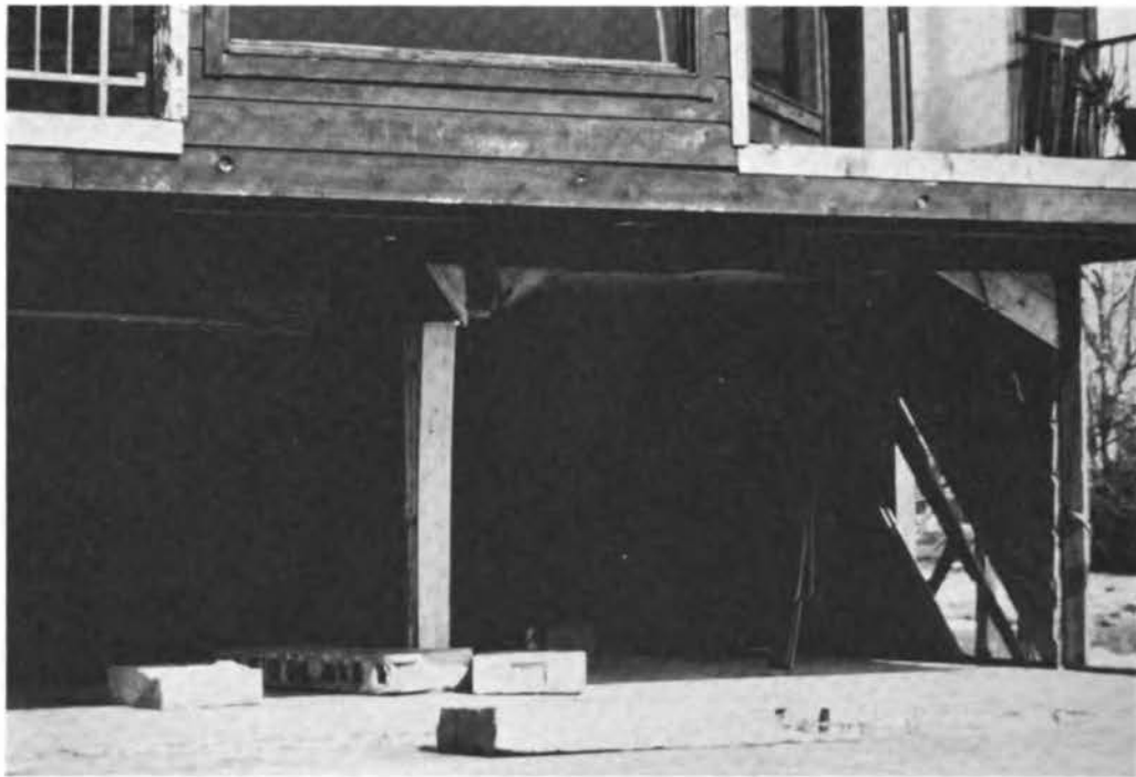
FIGURE 4.61 Damage to a grade-level enclosure.
