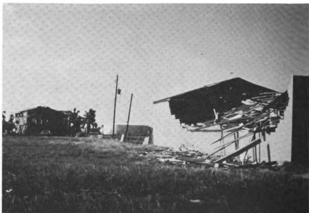
FIGURE 4.50 Damage to a large commercial warehouse building.
