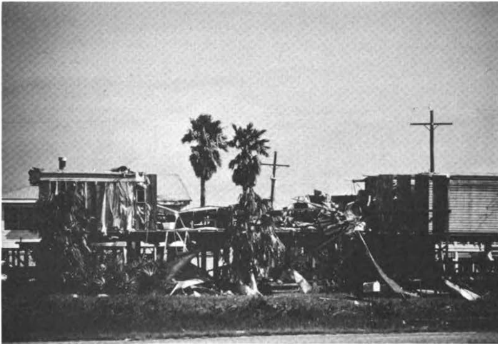
FIGURE 4.27 Damage to an elevated mobile home on West Beach.
