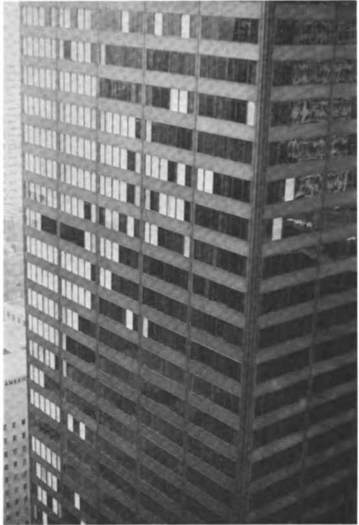
FIGURE 4.8 Closeup of glass damage to the Milam Building.
