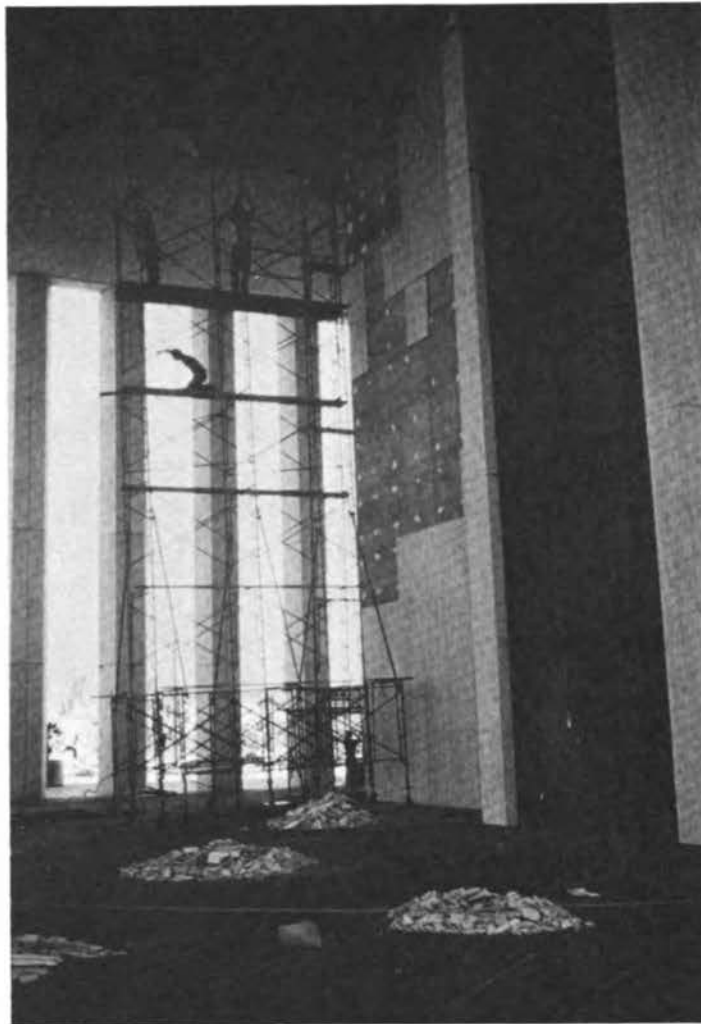
FIGURE 4.21 Damage to facade and glass of the American National Insurance Building.
