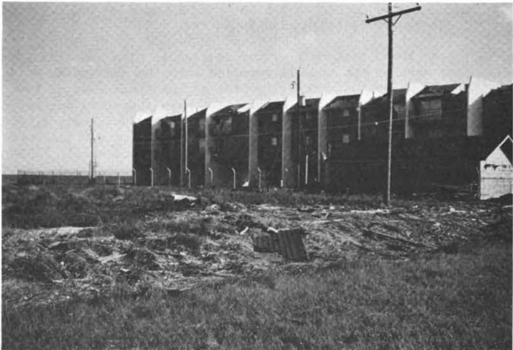
FIGURE 4.52 Damage to the roof and erosion around foundations of condominium units on the west side of San Luis Pass.
