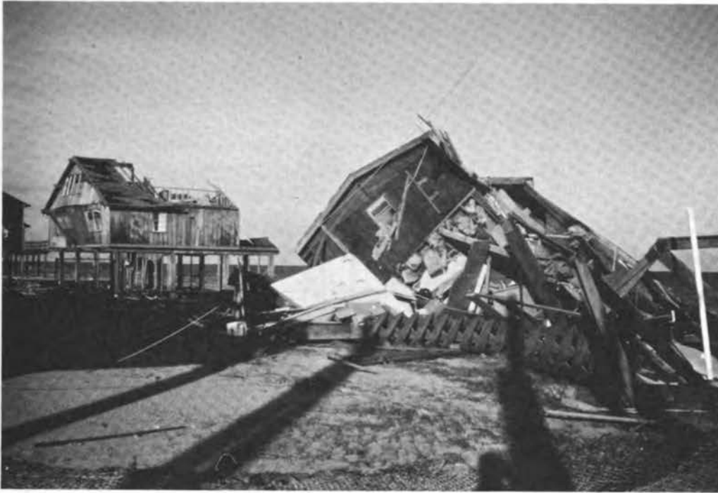
FIGURE 4.41 Example of overall collapse of a house and supporting structure.
