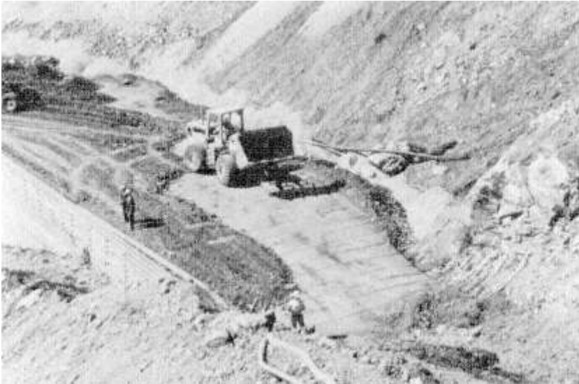
Figure 8 First reinforced earth wall constructed in the United States, along Highway 39 in the San Gabriel Mountains of Southern California.
