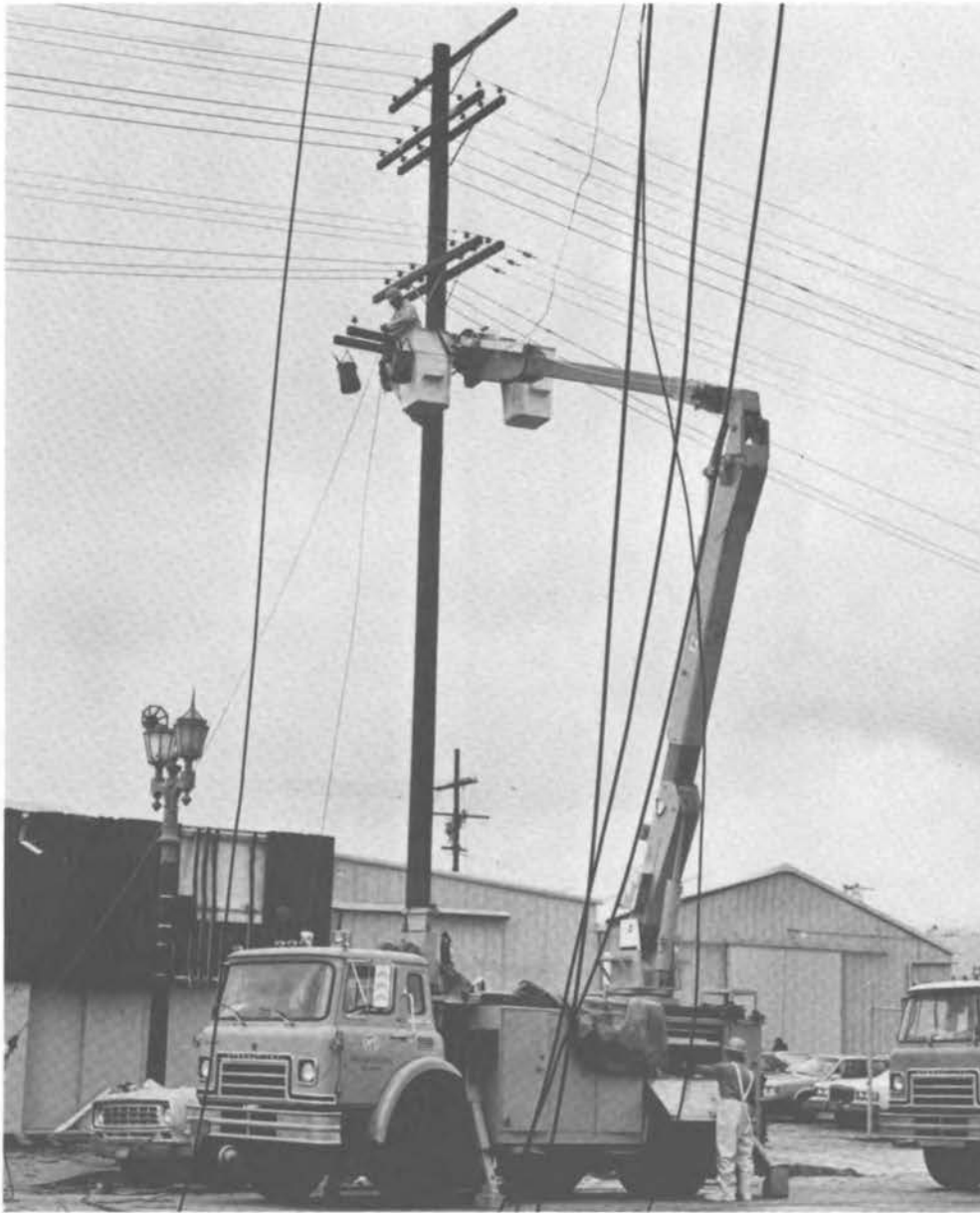
FIGURE 13 Restoration of electric power distribution lines by Los Angeles Department of Water and Power personnel.
