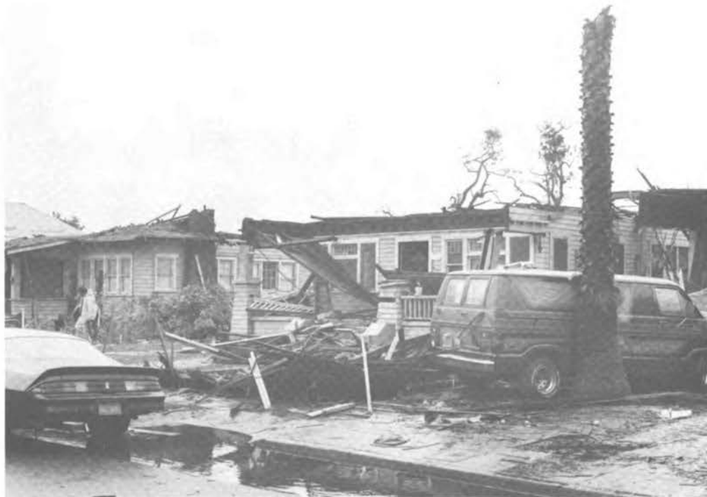
FIGURE 22 Damaged wood building in the 200 block of West Fortieth Place.
