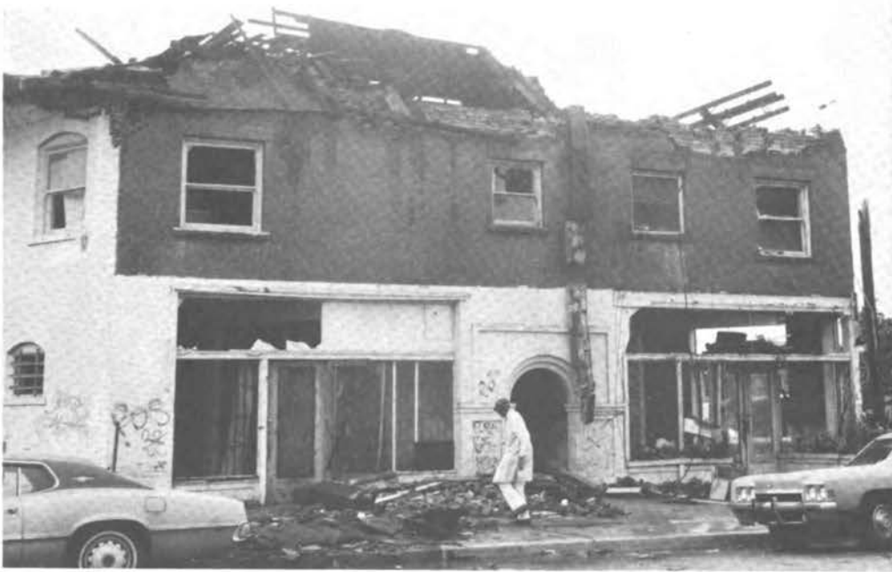
FIGURE 17 Collapsed masonry parapet.
