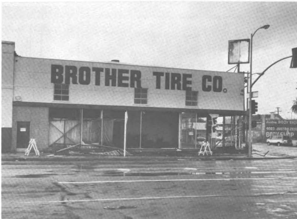
FIGURE 18 Failed storefront windows.
