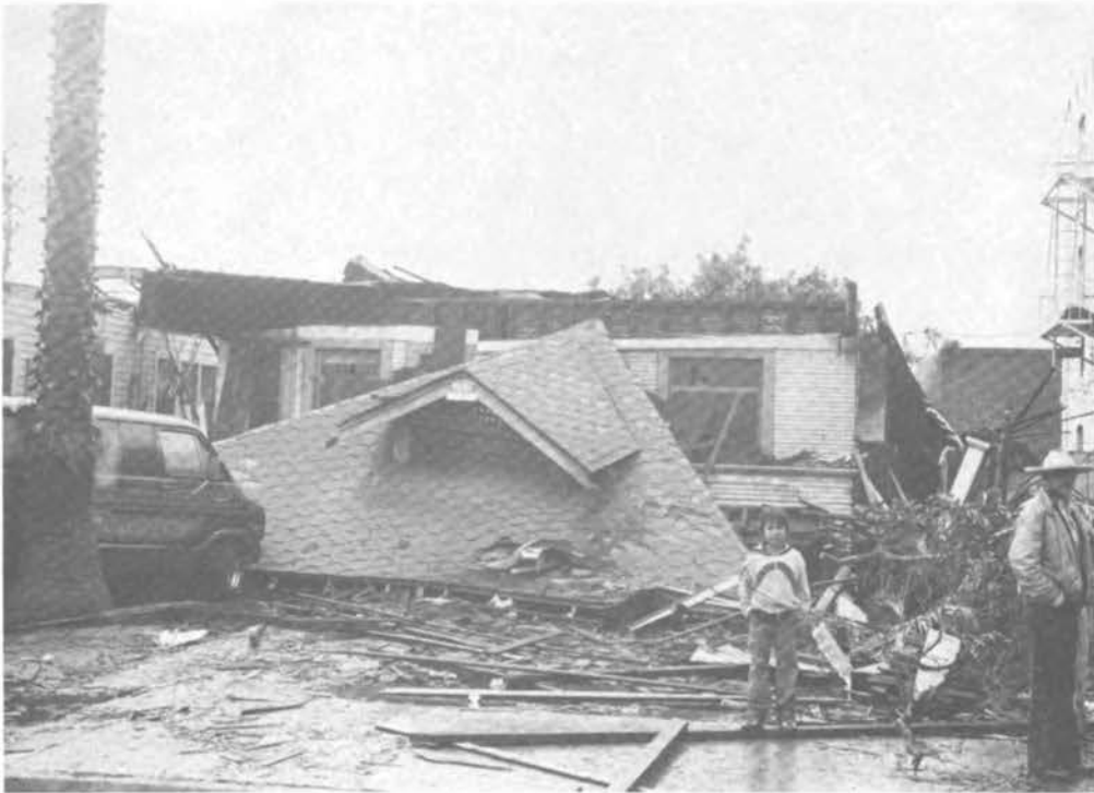
FIGURE 23 Collapsed roof at 260 West Fortieth Place.
