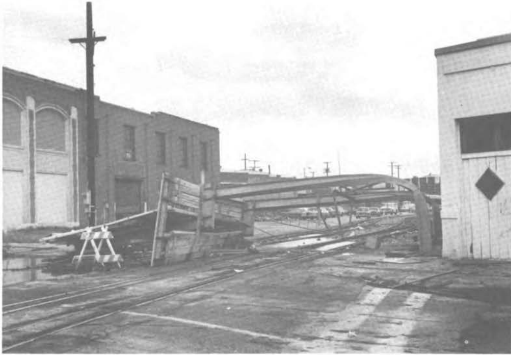
FIGURE 14A Industrial sign collapsed by tornado.
