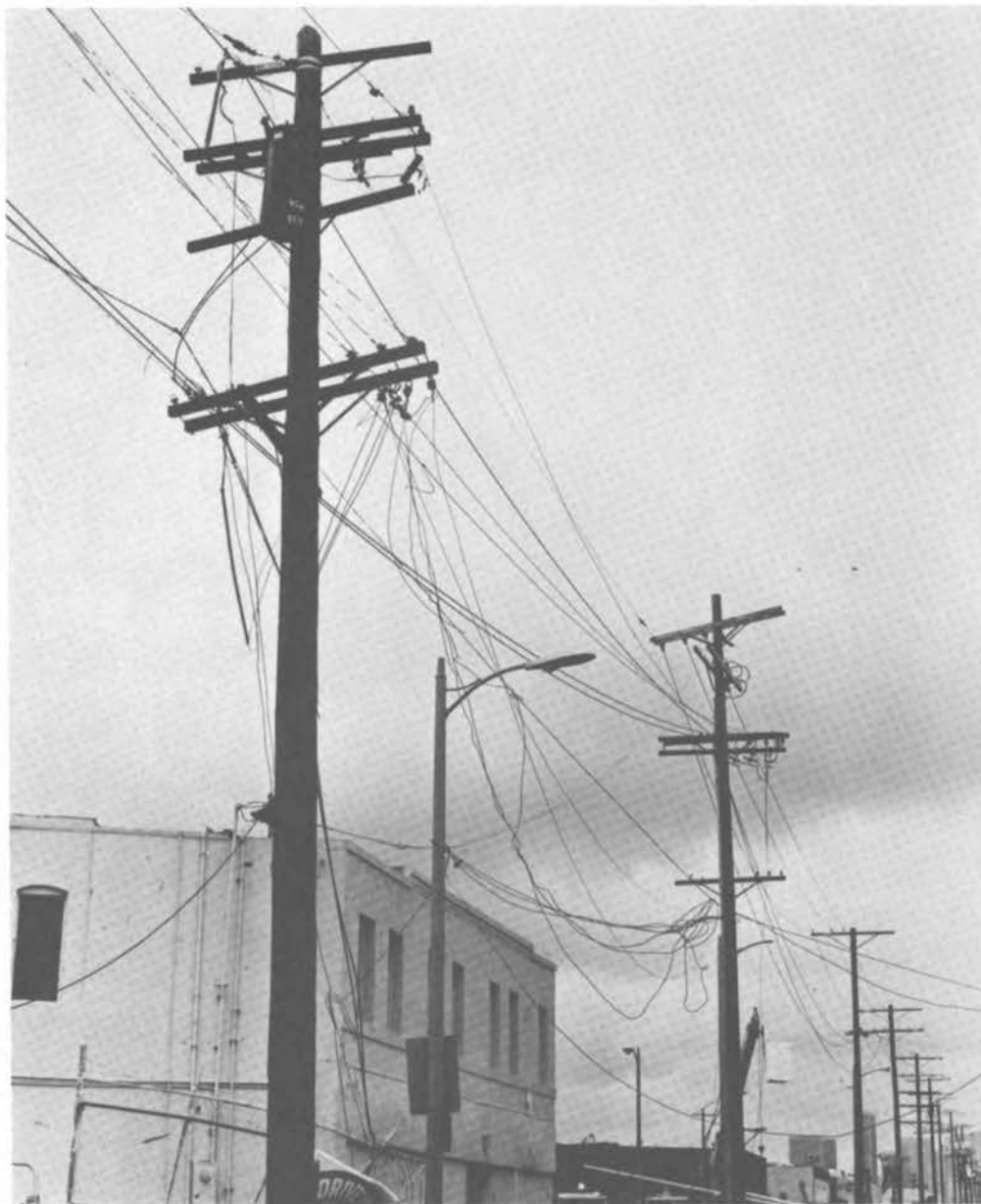
FIGURE 10 Damage to electric power distribution lines.
