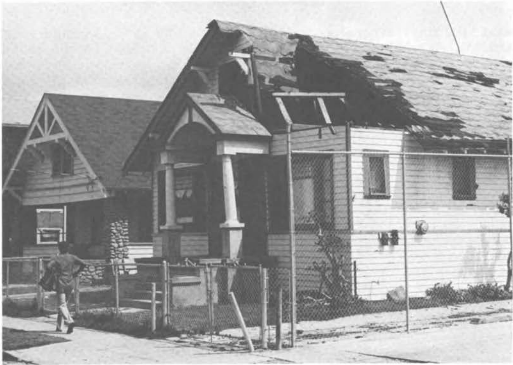
FIGURE 21 Damaged roof system at 268-70 West Forty-first Street.
