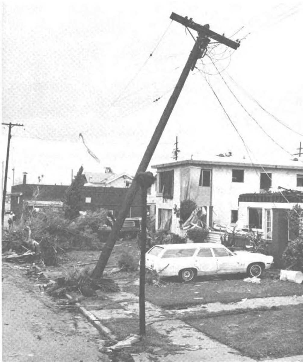
FIGURE 11 Wooden pole failure at ground level due to shear and flexural overstresses.
