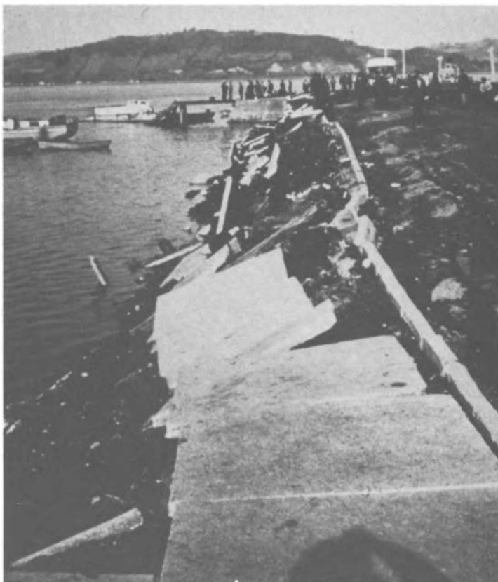
FIGURE 2-15 Example of a quay wall failure in Puerto Montt due to liquefaction during the 1960 Chilean earthquake. Photograph: Courtesy of G. W. Housner.
