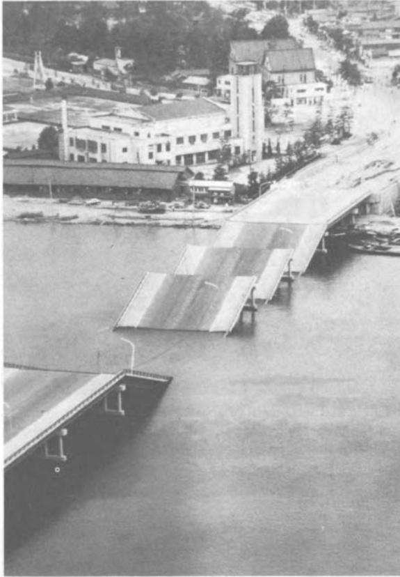
FIGURE 2-3 Failure of the Showa Bridge during the 1964 Niigata earthquake. Source: Seed and Idriss (1967).
