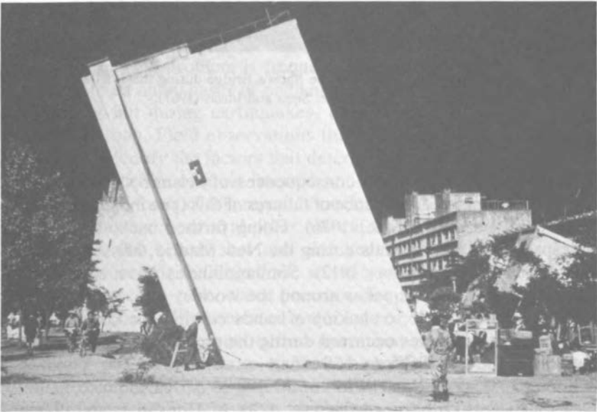
FIGURE 2-2 Close-up view of one of the apartment buildings affected by liquefaction during the Niigata earthquake. Photograph: Courtesy of G. W. Housner.
