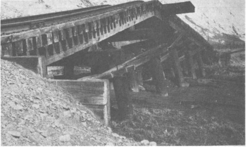
FIGURE 2-10 Bridge compressed and buckled by lateral spreading during the 1964 Alaska earthquake. Photograph: Courtesy of the U.S. Geological Survey.
