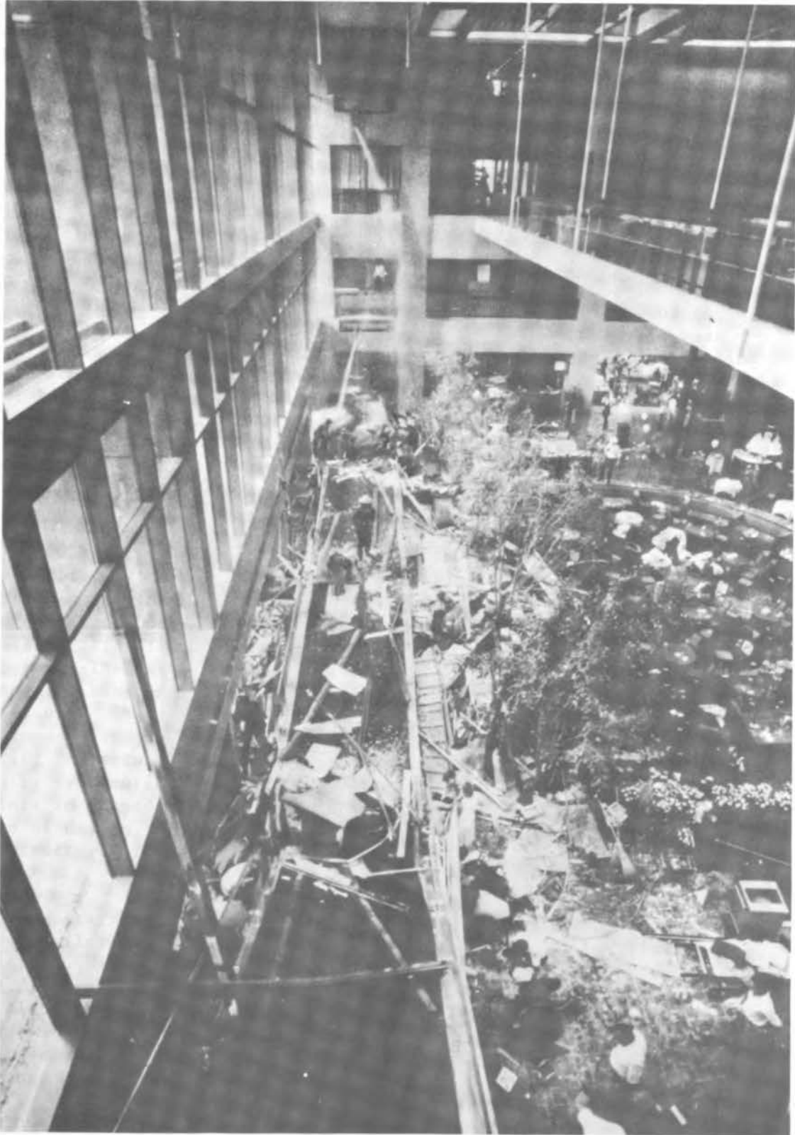
FIGURE 5 Walkways at the Kansas Hyatt Regency shortly after the collapse (reprinted by permission of the Kansas City Times, © 1981).
