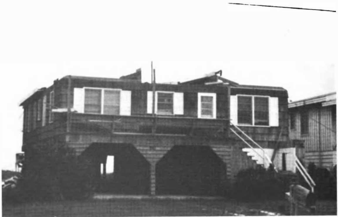
FIGURE 3.4 Roof damage, Holden Beach.
