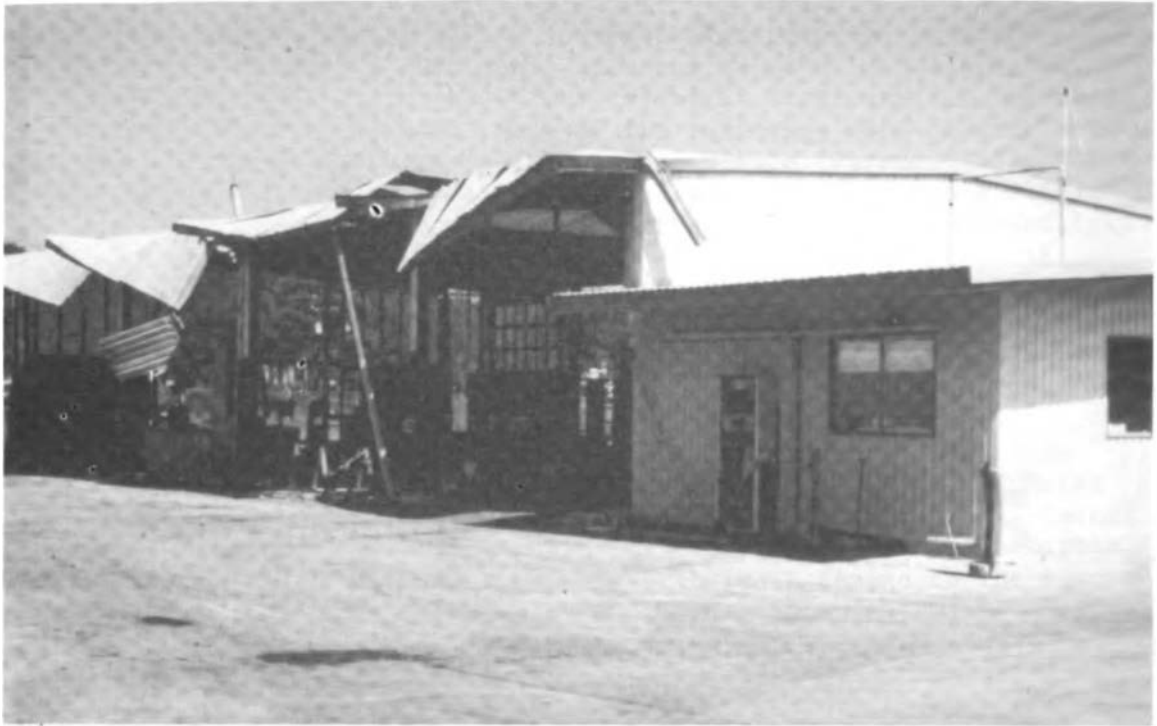
FIGURE 3.17 Damage to preengineered building, Southport.
