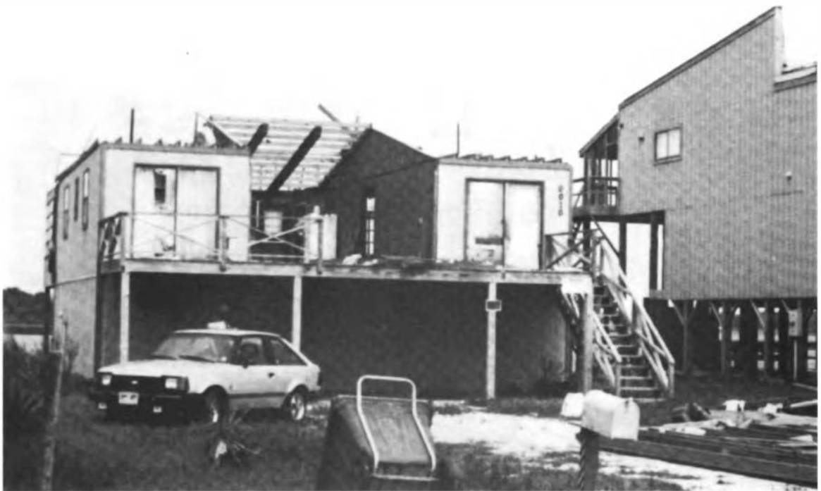
FIGURE 3.12 Roof damage to recently constructed house, Long Beach.
