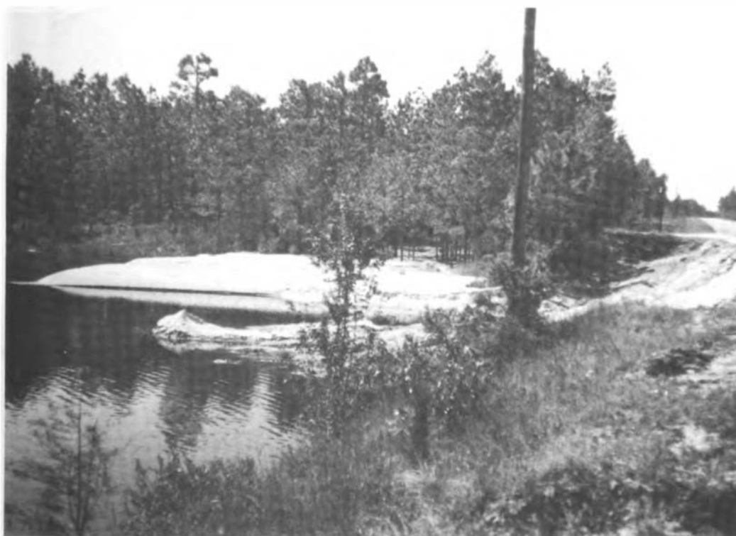
FIGURE 3.44 Part of dam 2 with partial stability failure.
