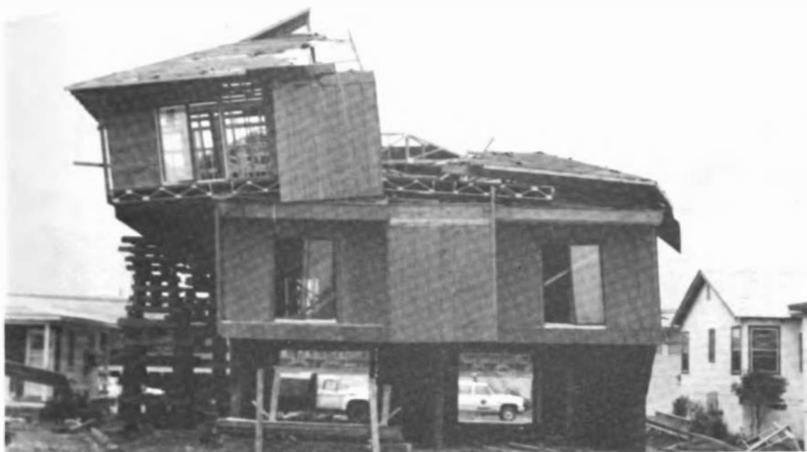
FIGURE 3.27 Shear failure of a condominium building, Carolina Beach.
