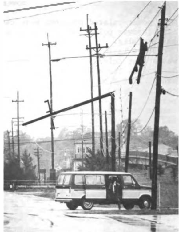
FIGURE 3.36 Downed telephone poles in Wrightsville Beach. The top of another pole hangs by a strand on the right. Photograph courtesy of Wilmington Morning Star , September 13, 1984; staff photograph by Gray Honeycutt.
