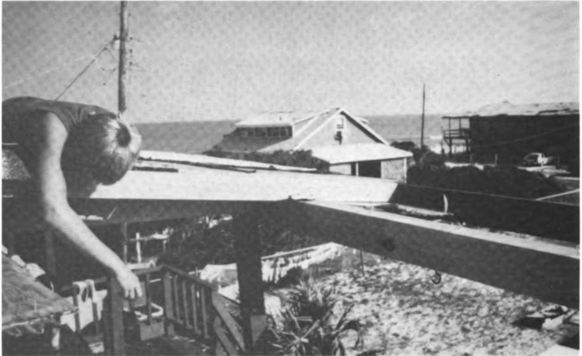
FIGURE 3.23 Incorrect use of hurricane anchors in a motel porch.
