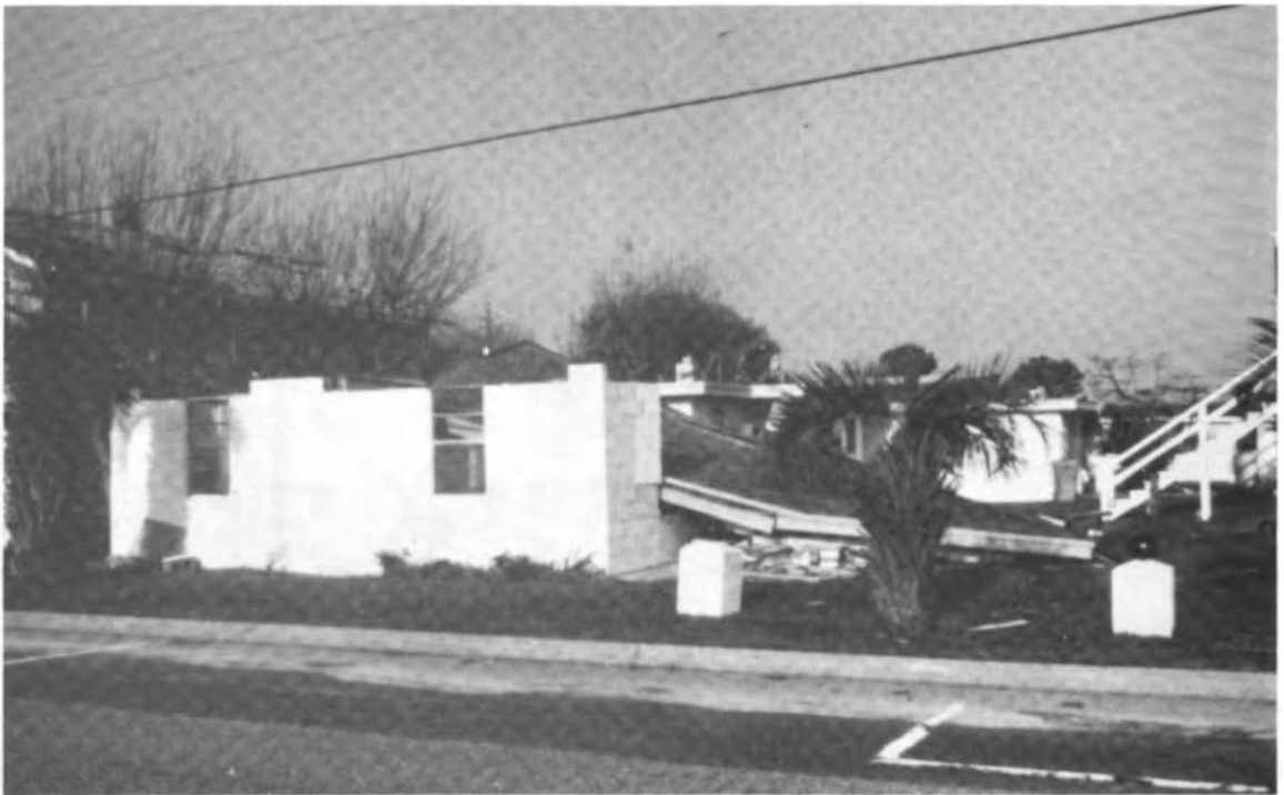
FIGURE 3.24 Loss of poorly anchored roof in a masonry building, Kure Beach.
