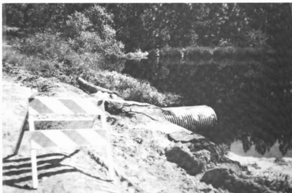
FIGURE 3.43 Drainage pipe of dam 3 on Boiling Spring Lakes clogged by fallen branches and debris.
