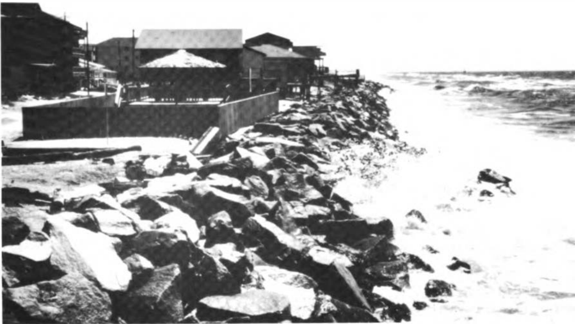
FIGURE 2.10 Beach erosion permitting storm waves to reach revetment in Carolina Beach.
