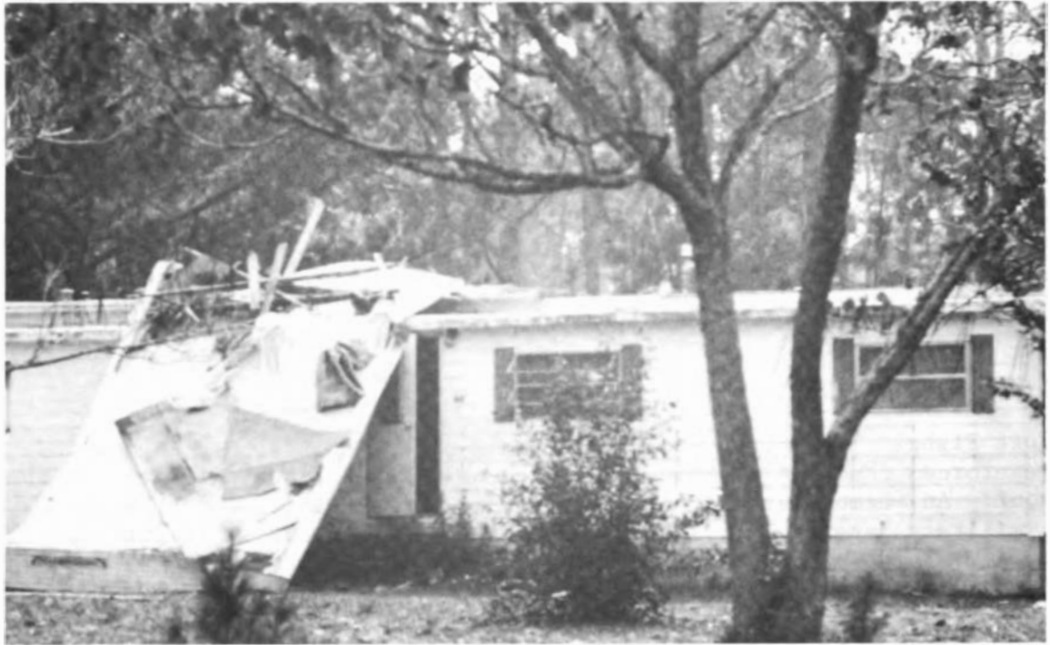
FIGURE 3.19 Loss of mobile home roof near Grouse Landing.
