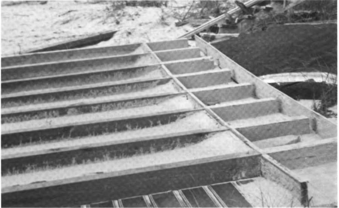
FIGURE 3.11 Detail of poor roof connection, "Blue Haven," Long Beach.
