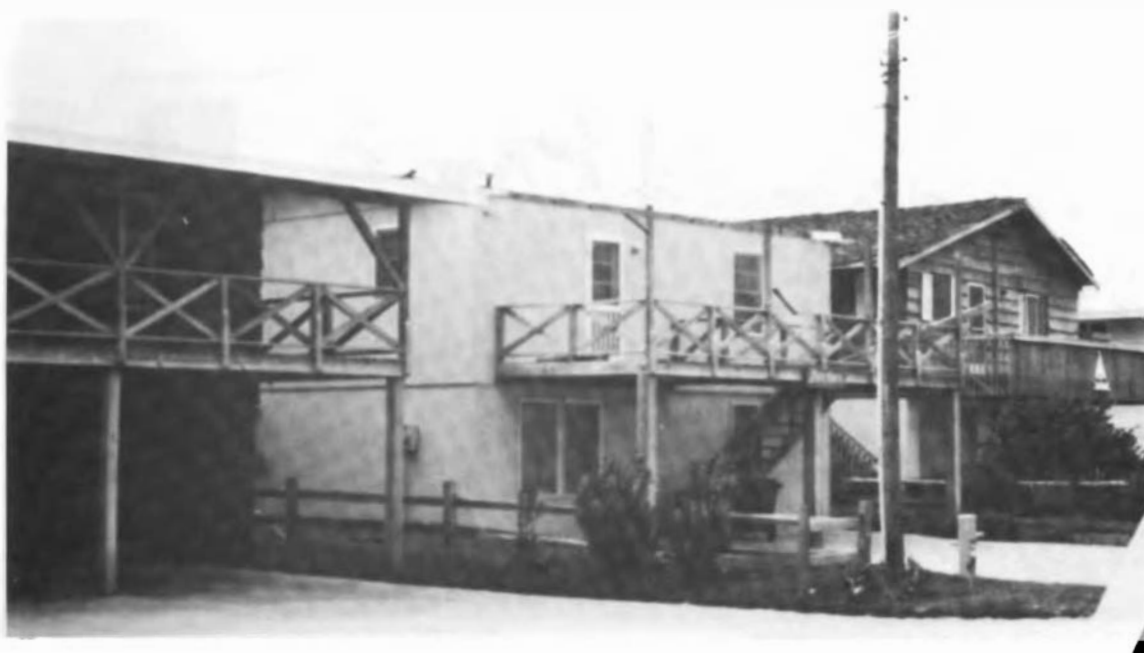
FIGURE 3.6 Porch and roof damage, Long Beach.
