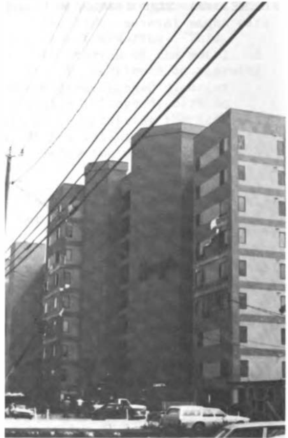
FIGURE 3.35 Cladding failure, North Myrtle Beach.
