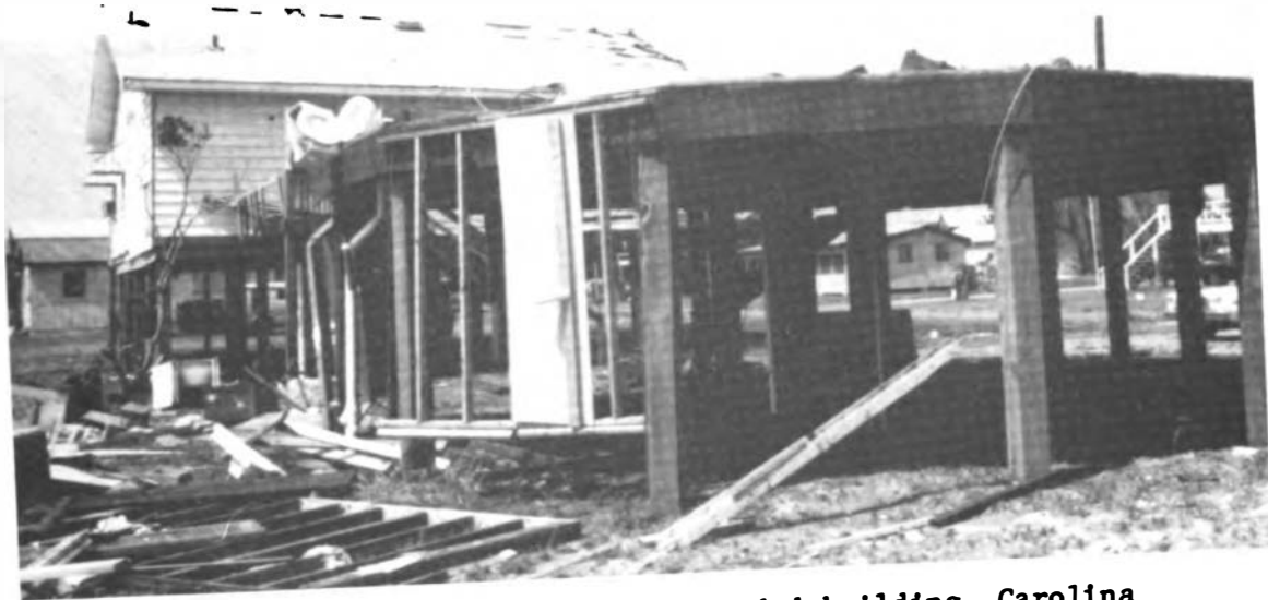
FIGURE 3.31 Complete failure of 12-sided building, Carolina Beach.
