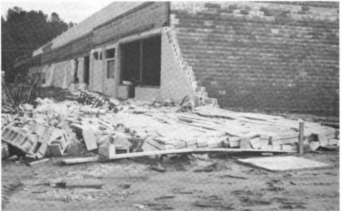
FIGURE 3.20 Failure of masonry wall in a shopping center under construction, Shallotte.
