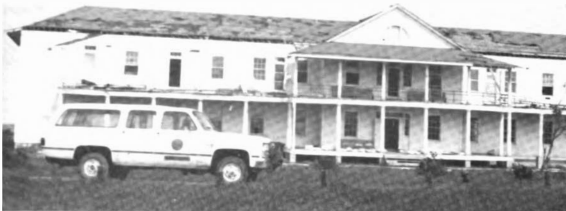
FIGURE 3.15 Porch damage to old military building, Fort Caswell.
