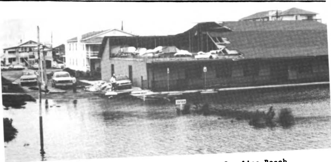
FIGURE 3.32 Restaurant roof failure, Carolina Beach.
