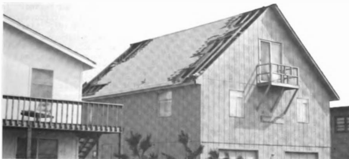
FIGURE 3.14 Eave and roof damage, Caswell Beach.
