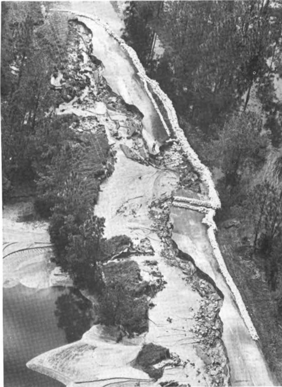
FIGURE 3.46 Washed-out section of road atop a dam in Boiling Springs Lakes. Sandbags placed by the U.S. Army Corps of Engineers kept the dam and other dams from collapsing. Photograph courtesy of Wilmington Morning Star , Saturday, September 15, 1984; staff photograph by Dan Sears.
