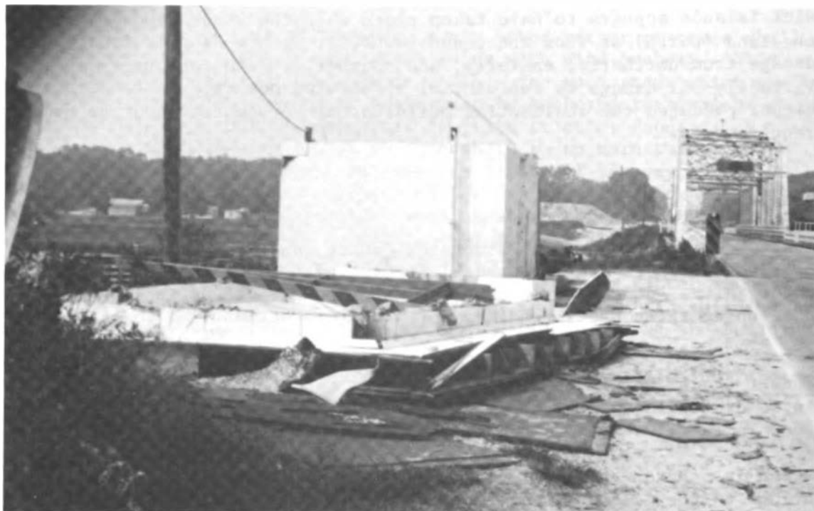
FIGURE 3.2 Roof failure of masonry building, Ocean Isle Beach.
