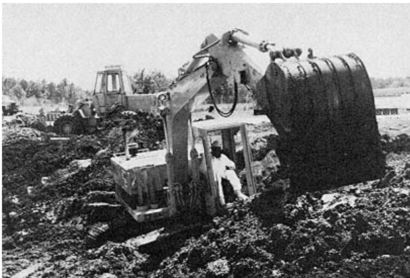
Figure 2 Lead-contaminated soil is removed at the Sapp Battery hazardous waste site in Florida's Panhandle.
