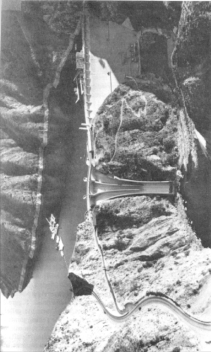
Figure 2-5 Morris Dam, California, was constructed over a known fault in the foundation rock with a vertical sliding joint formed in the concrete directly above the fault (2-64). The joint passes next to the galley entrance, visible on the downstream face.
