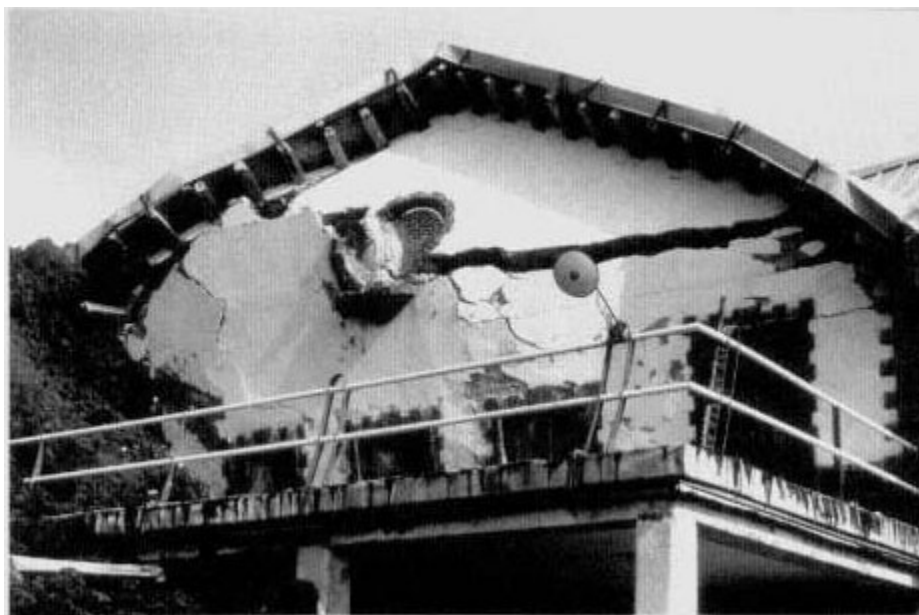
The stucco facade of this building shattered like an eggshell as lava flowing around the base of the three-story structure applied such pressure that the walls shifted and collapsed.
