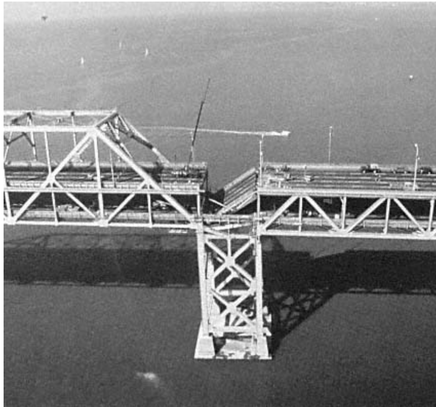
The spectacular damage caused to the highway and bridge systems of the San Francisco Bay area during the Loma Prieta earthquake is being studied for applications to updating building and safety codes.
