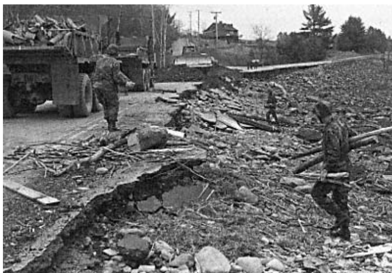
Different disasters can produce similar damage. Though it looks like an earthquake rocked this interstate to pieces, this Maine roadway was damaged by floodwaters and the resultant landslides. As is often the case for local-level response, the local National Guard Engineering Group mobilized for clean-up and repair during the state-declared emergency.
