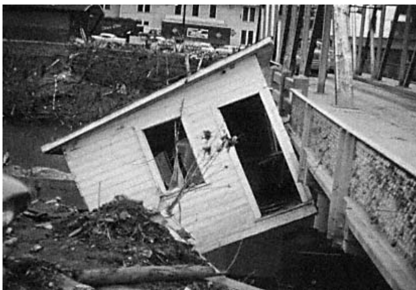
The haphazard wreckage of buildings blocks roadways and bridges—in this case a complete shack knocked off its foundation by an earthquake.
